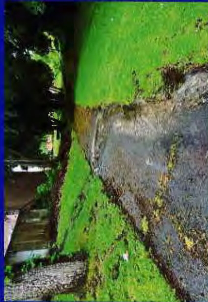
drainage issues and debris, looking to Exchange
