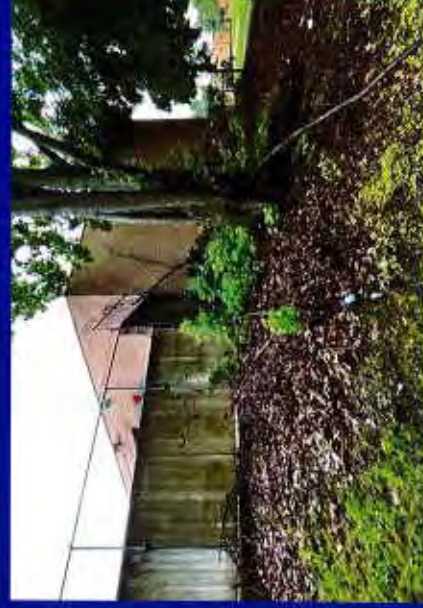
drainage issue area and adjacent property wall
