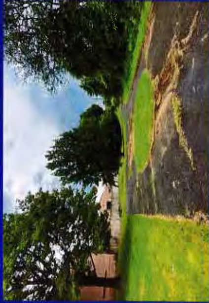
pavement area with unknown circle feature
