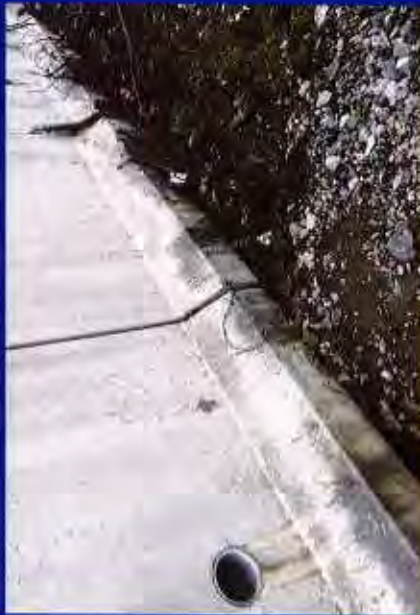
wall drain hole (one of dozens) with undercut
