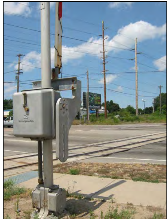
CSX railroad at-grade crossing with West Ridge Road, one of two such crossings in the Study Area.
