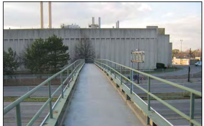
Pedestrian bridge over Mt. Read Boulevard looking west toward Building 339 in EBP.
