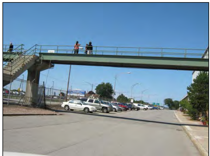
The pedestrian bridge over Mount Read Boulevard could be replaced to meet the needs of both EBP and trail users.
