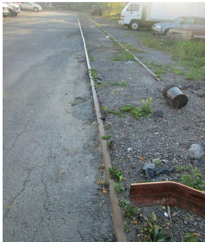
Rail corridor encroachment by existing business at 190 Murray Street.
