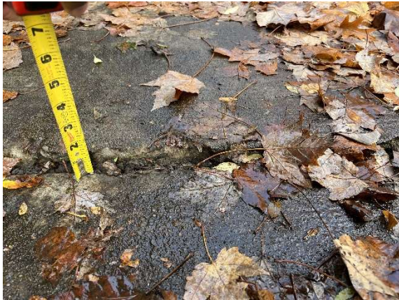
Photo Description Trip Hazard Replace sidewalk to remove hazard
