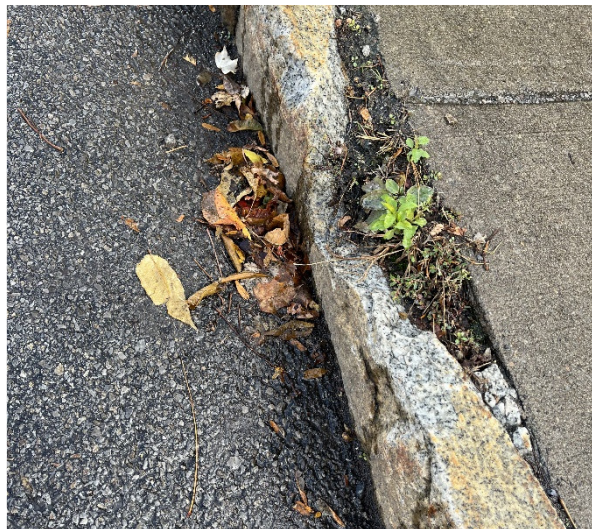
Photo Description Broken Curb Replace Curb
