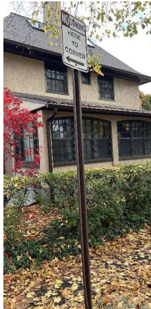
Photo Description Post Mounted Sign (Crooked Post) Faded Sign with Limited Reflectivity Sign and Post to be Replaced
