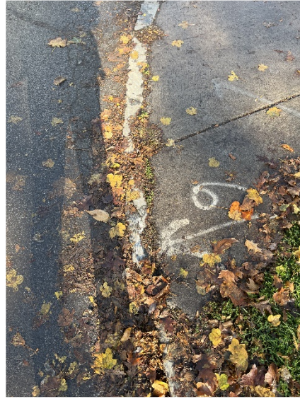
Photo Description Broken Curb Replace Curb
