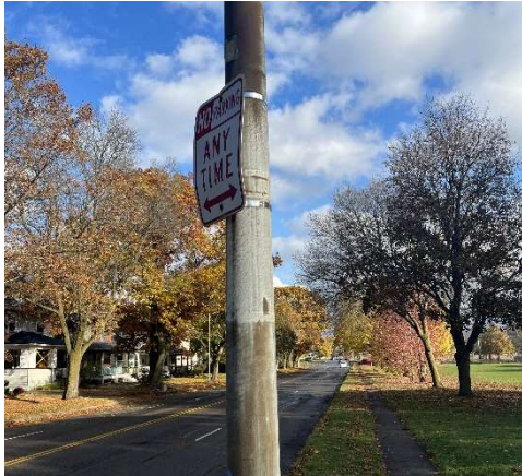
Photo Description Pole Mounted Sign (Band Mounted) Damaged Sign Sign Panel (only) to be Replaced
