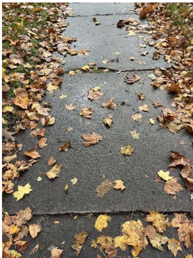
Photo Description Trip Hazard Replace sidewalk to remove hazard
