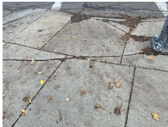
Photo Description Sidewalk Cracking Replace sidewalk to remove cracked sections
