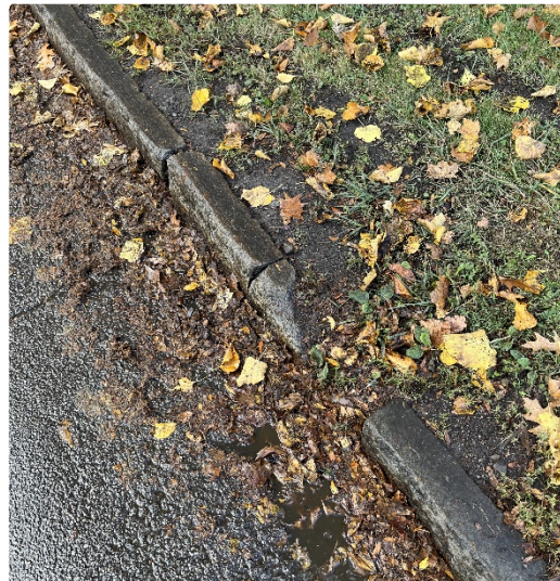
Photo Description Broken Curb Replace Curb
