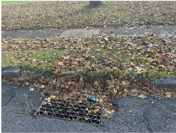
Photo Description Missing Curb Reset Curb
