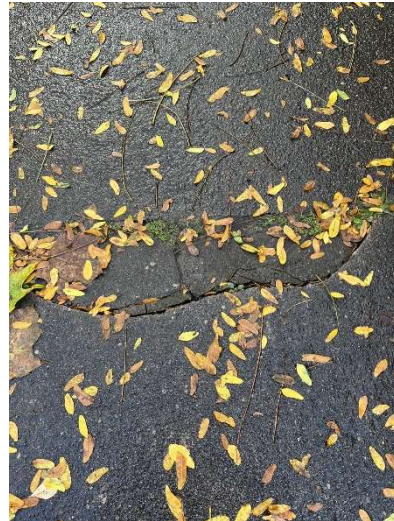
Photo Description Sidewalk Cracking Replace sidewalk to remove cracked sections
