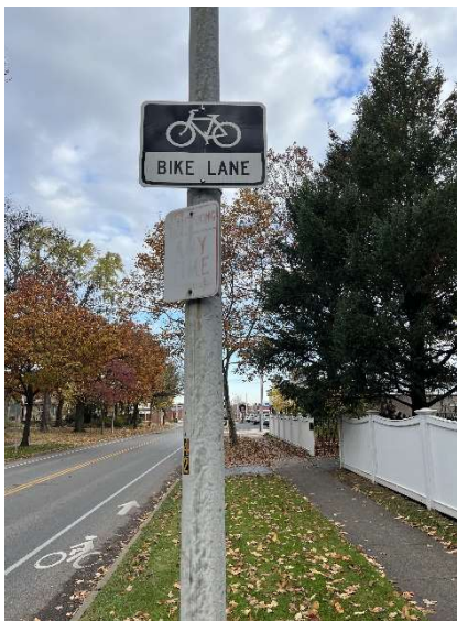
Photo Description Pole Mounted Sign (Band Mounted) Faded sign with Limited Reflectivity Sign (only) to be Replaced
