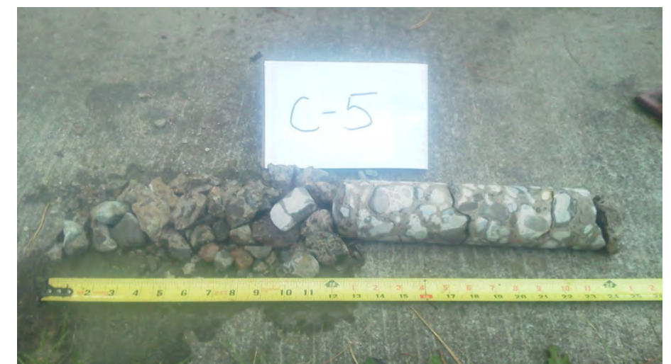
PHOTO OF CONCRETE CORE SAMPLE FROM THE WEST RIVER WALL
