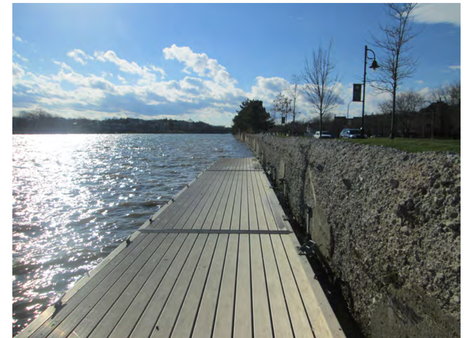
VIEW OF RIVER SIDE OF WALL LOOKING UPSTREAM FROM CORN HILL LANDING Waterfront Recreation and Natural Resources
