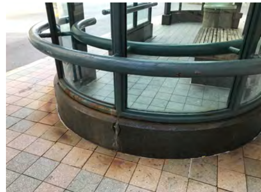
Deteriorated Bus Shelter
