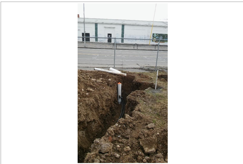
VEGE Extraction Well EX-6 and O2 injection point IP-6
