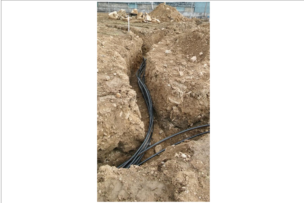
Trenches with VEGE extraction and O2 injection lateral lines
