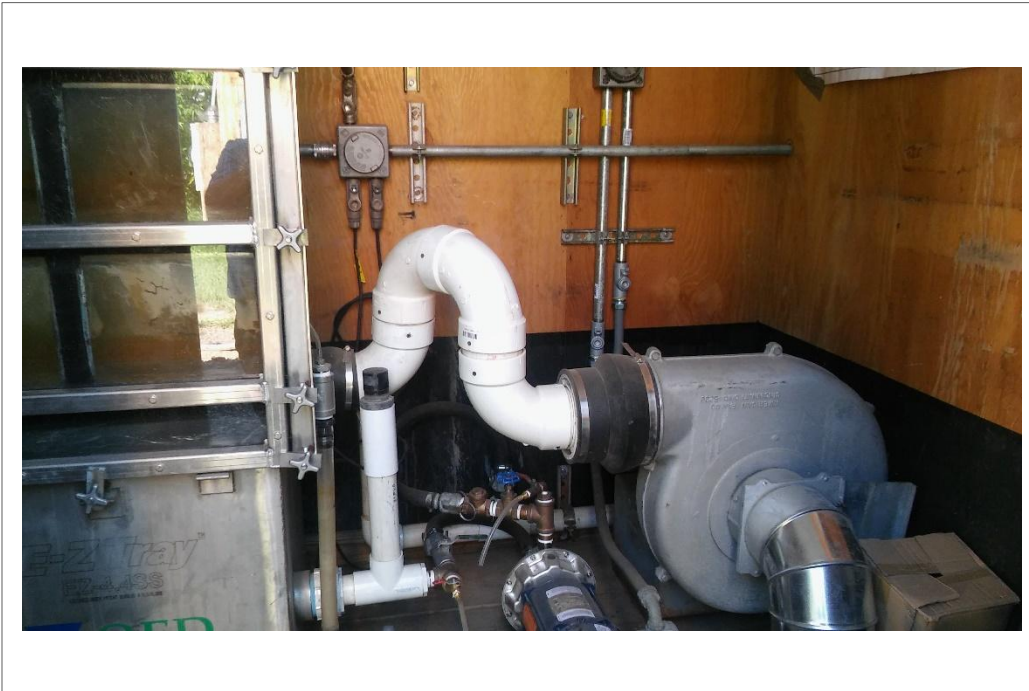
VEGE System air stripper and vacuum motor
