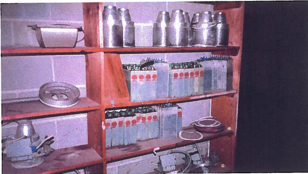
View of the batteries observed within the basement of low-rise apartment building #285.
