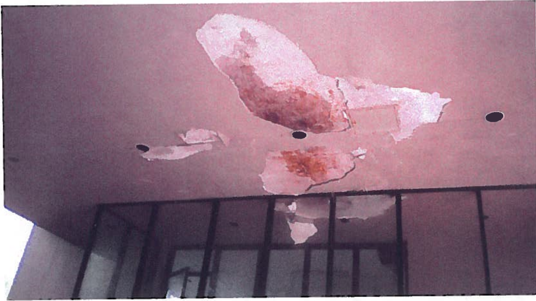
View of damaged concrete observed on the exterior portion of the low-rise apartment buildings.
