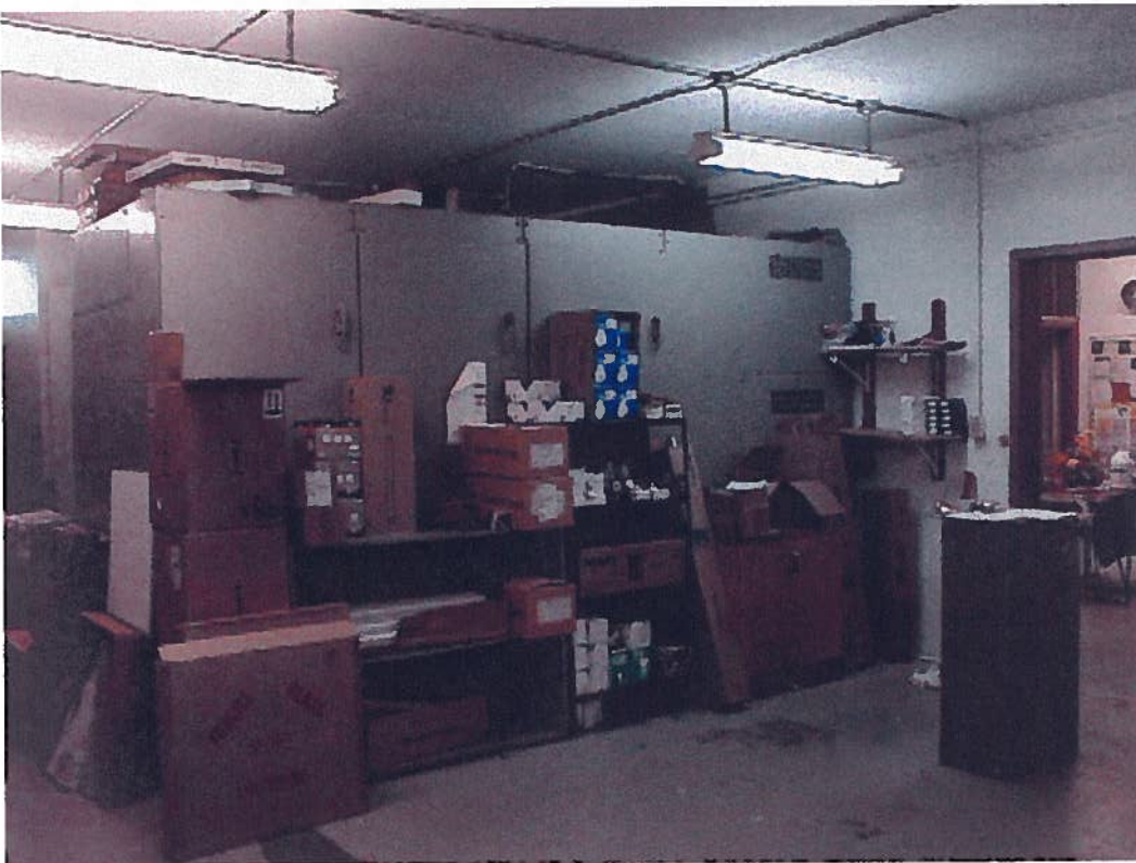
View of the transformers observed in the high-rise apartment building.
