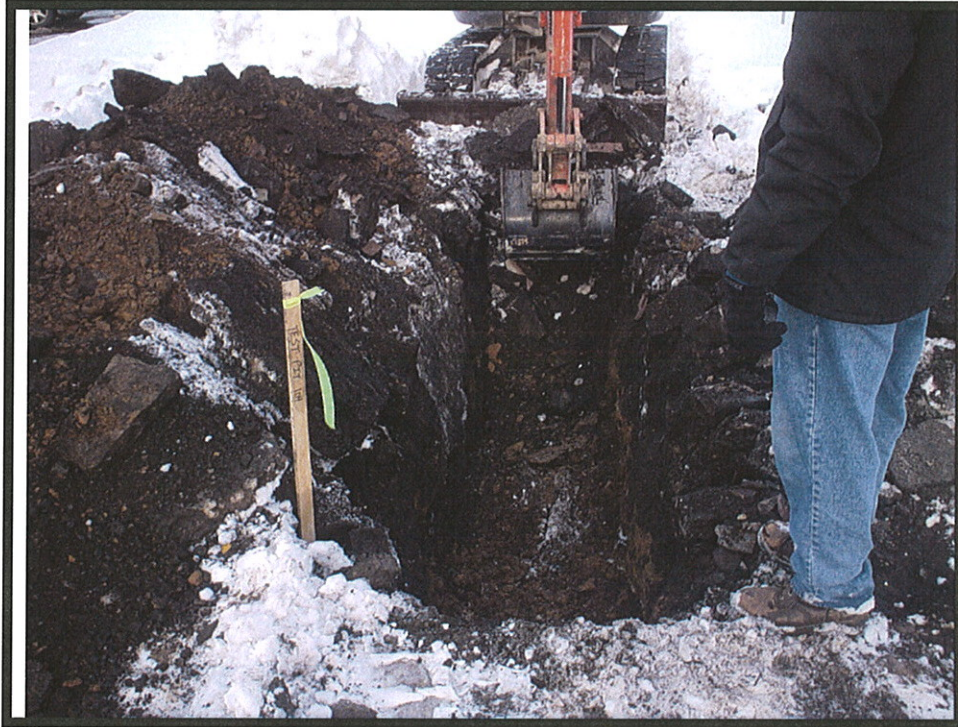
View of the TP-104 showing light brown native soil and weathered bedrock
