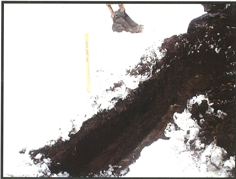
View of the TP-109 showing fill materials layer and native soil layer
