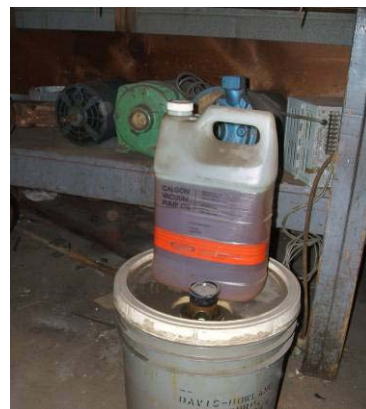
Lubricants - McCurdy's sub-basement
