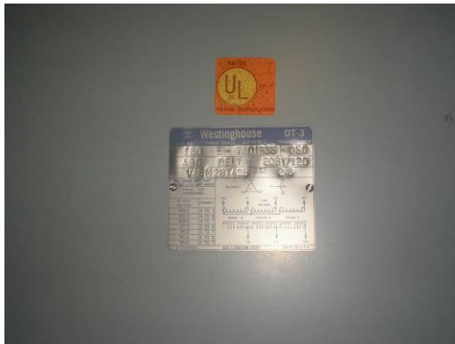
Transformer – dry type, 6 th floor
