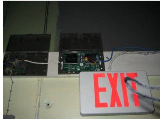
Exit sign in basement
