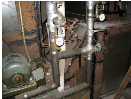
Mechanical room in basement of B. Forman Building
