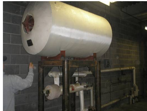
Hot water tank in elevator penthouse
