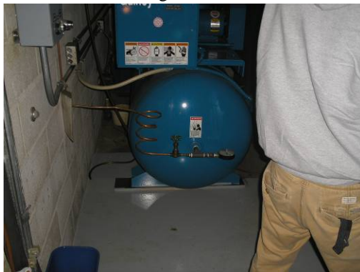
Compressor on 7 th Floor
