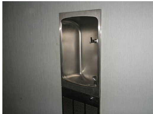
Water fountain on 16 th floor
