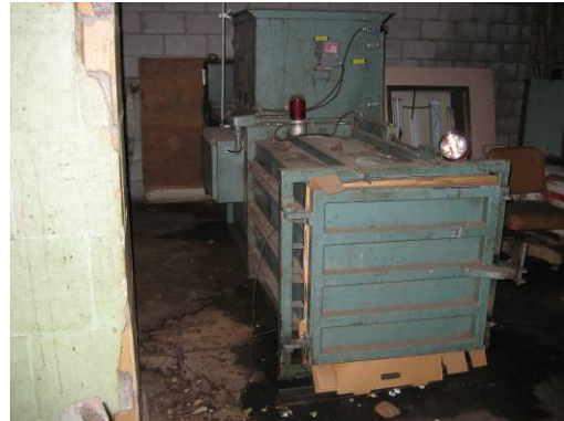
Cardboard Compactor in basement
