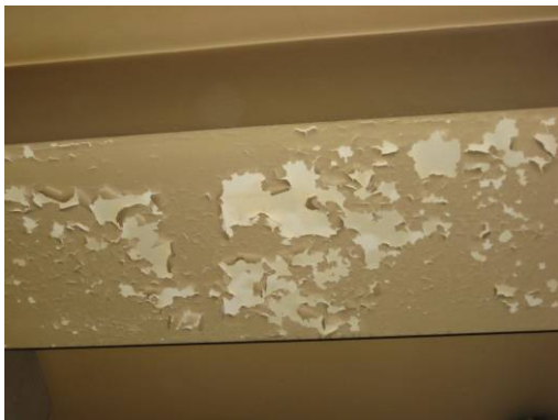
Peeling paint in basement
