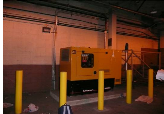
Natural gas generator at underground service tunnel near McCurdy's Building
