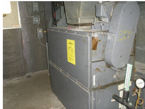
Blower on 15 th floor
