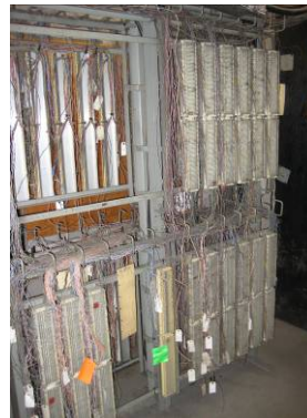
Telephone connection in telephone room of basement
