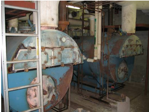
Boilers in boiler room
