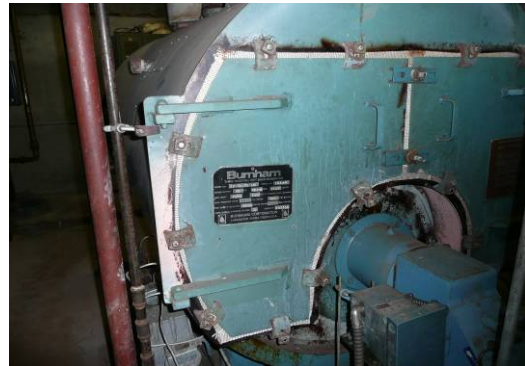
Boiler in sub-basement of McCurdy's Building
