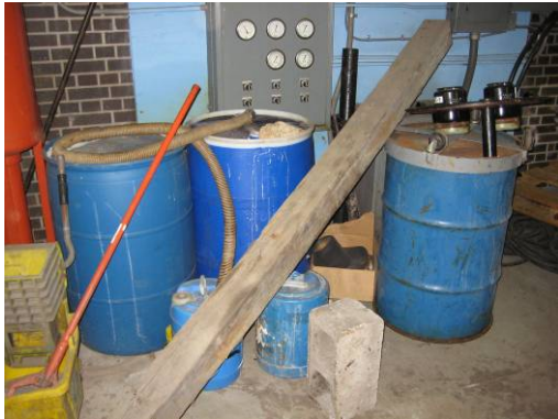
Drums (one full) in boiler room
