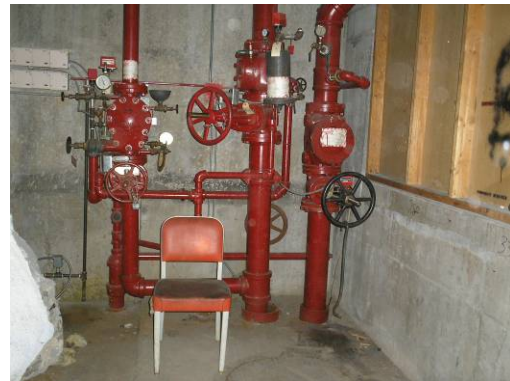
Fire suppression piping
