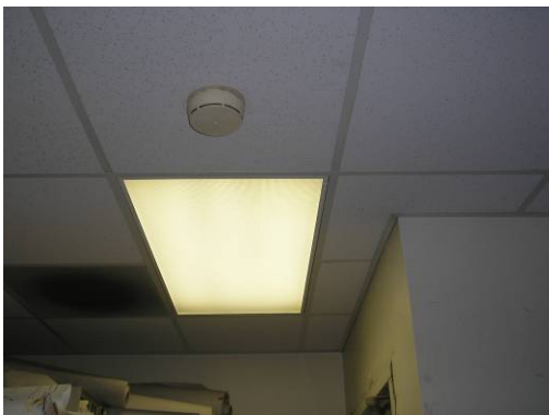
Fluorescent lights on 3 rd Floor
