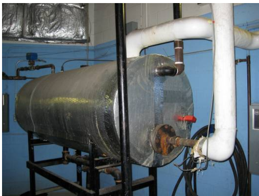
Expansion tank in boiler room
