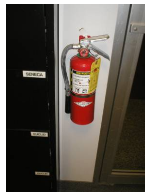
Fire extinguisher on 3 rd Floor
