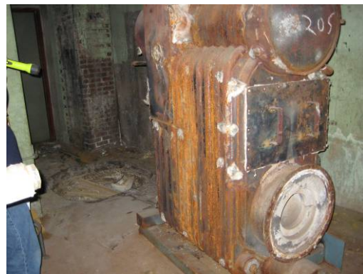
Boiler core in boiler room
