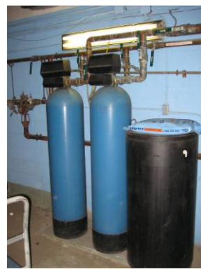
Water softener in Boiler Room
