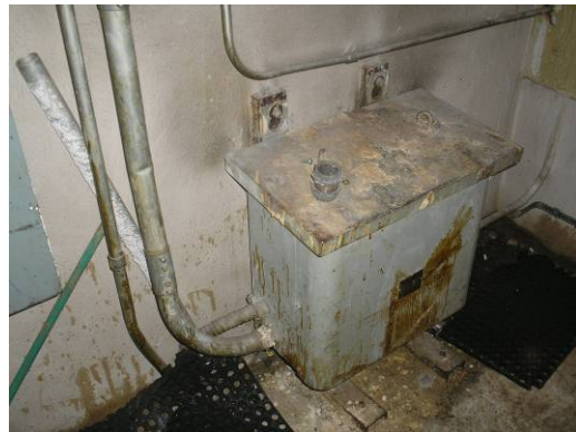
Transformer on 14 th floor
