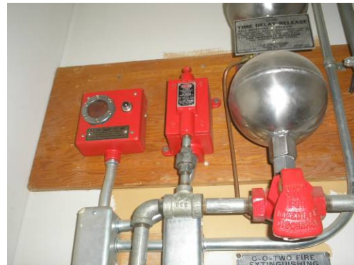
Fire suppression system on 7 th Floor
