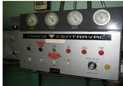
Chiller Control panel
