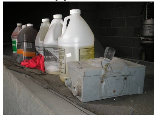
Chemicals in Elevator penthouse
