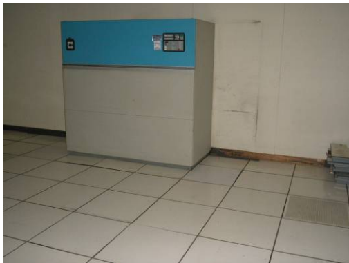
A/C Unit on 7 th Floor
