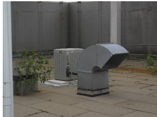
Air conditioner on roof
