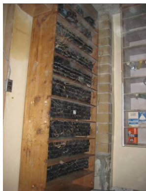
Ballasts in storage area of McCurdy's Building
