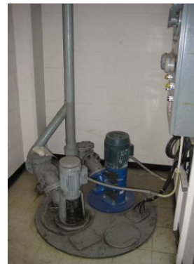
Sump and pumps in basement
