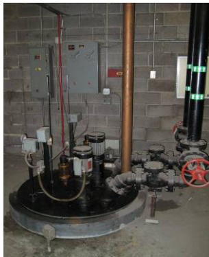
Sump pit and pumps to sewer in the northwest end of mechanical area
