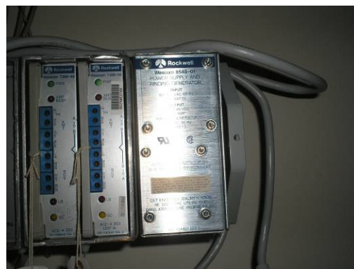
Controls for generator on 10 th floor
