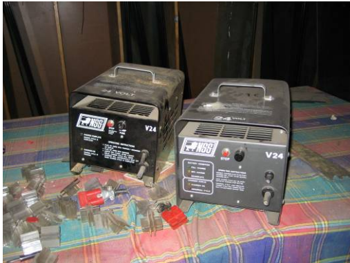
Power converters in basement
