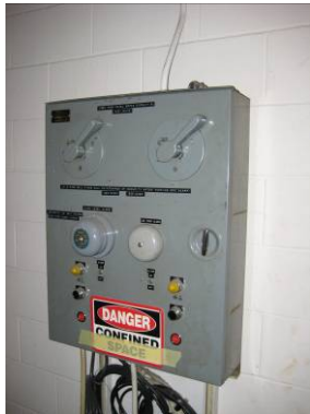
Panel for sump pumps in basement
