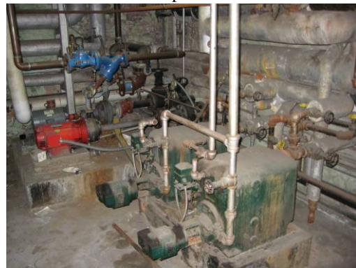
Oil filled vacuum pump in mechanical room
