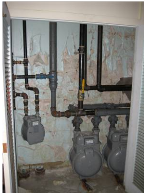
Gas meters in basement of B. Forman Building
