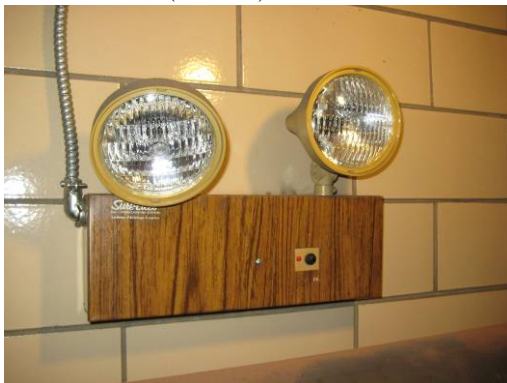
Emergency lighting in boiler room
