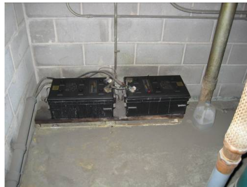
Batteries for electric generator
