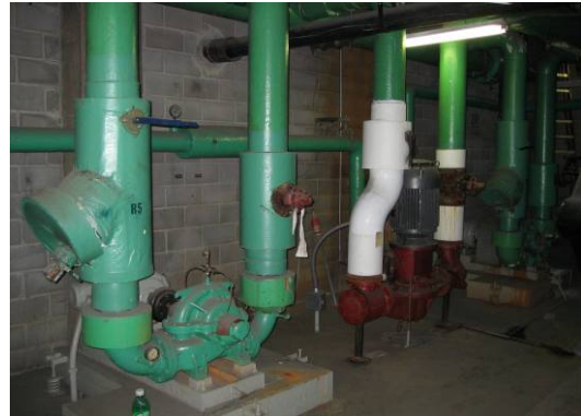
Cold water pumps
