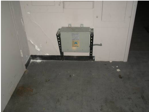
Transformer on 7 th Floor
