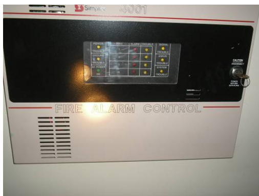
Fire alarm control on 10 th floor
