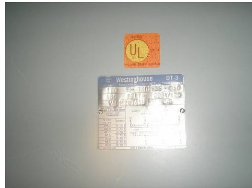
Transformer (dry type) on 7 th Floor
