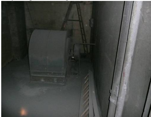
Vent fan in underground service tunnel near Seneca Building loading dock
