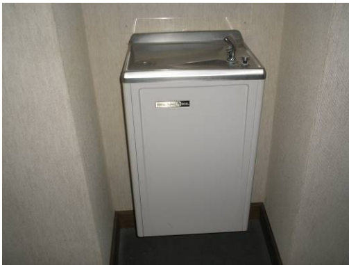
Water fountain on 7 th Floor
