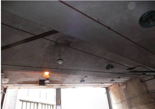
Mercury lamps at underground service tunnel entrance
