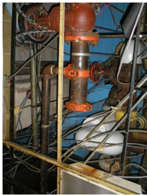
Piping on 14 th floor
