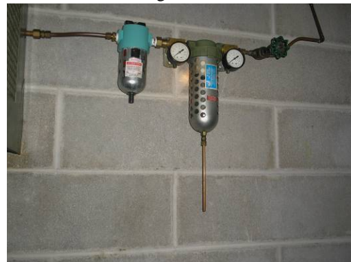
Air line Filter on 7 th Floor
