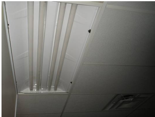
Typical fixture on 4 th Floor
