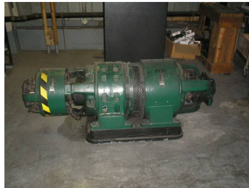
Oil filled motor - elevator penthouse
