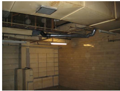
Fluorescent lights in basement
