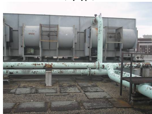
Equipment on roof
