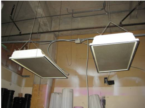
Fluorescent light fixture in basement
