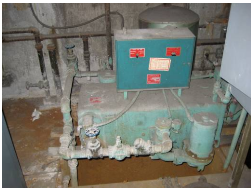
Oil-filled vacuum pump basement of B. Forman
