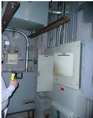
3 rd Floor mechanical room near stair A at Seneca Building
