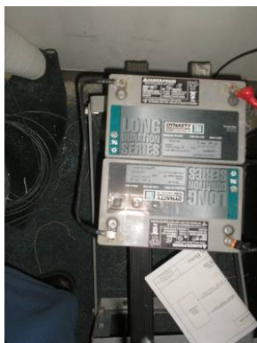
Batteries on 16 th floor
