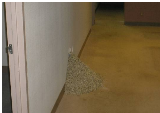
Vermiculite in wall 9 th floor
