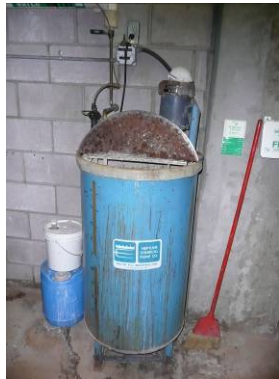
Descaler mixing tank Sub-basement of McCurdy's
