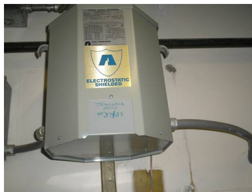
Transformer on 11 th floor
