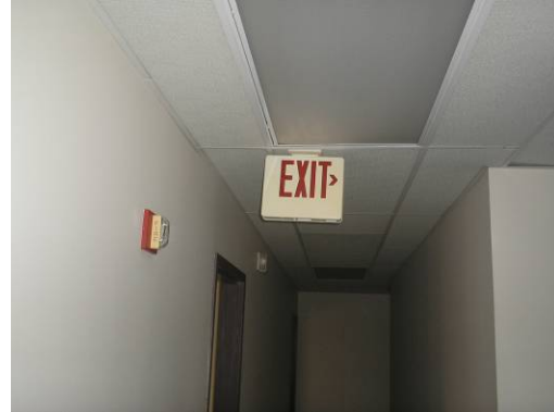
Emergency lighting and Exit sign on 4 th Floor
