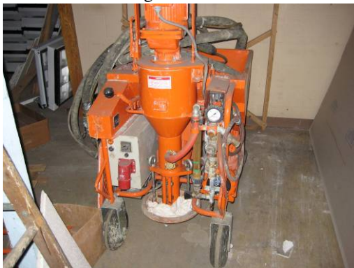
Cement pump in basement
