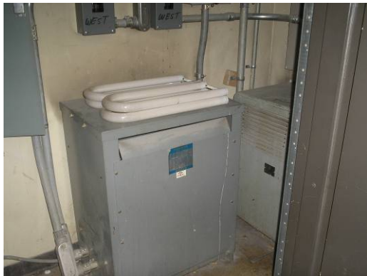
Transformers 16 th floor
