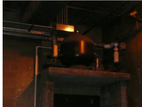
Compressor in underground service tunnel
