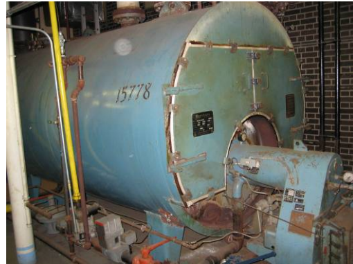
Boiler in boiler room
