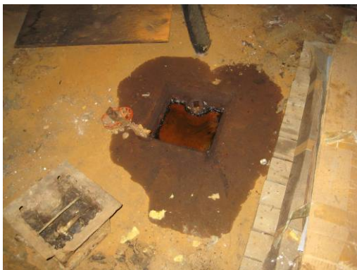
Staining on floor in basement
