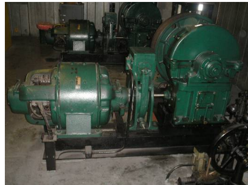
Elevator penthouse motor
