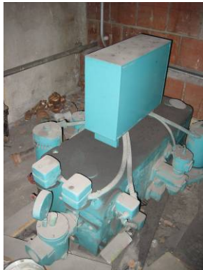
Vacuum pump in back room of basement
