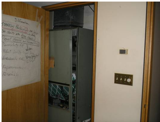
AC Unit on 15 th floor
