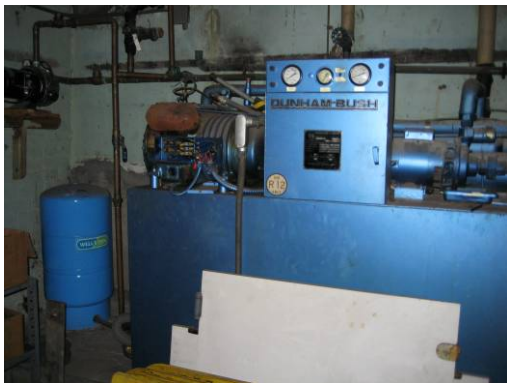
Cooling unit in basement
