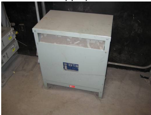
Transformer on floor in telephone room of basement
