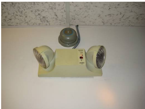
Emergency lights in hall basement
