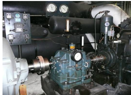
Out of service chiller in sub-basement of McCurdy's
