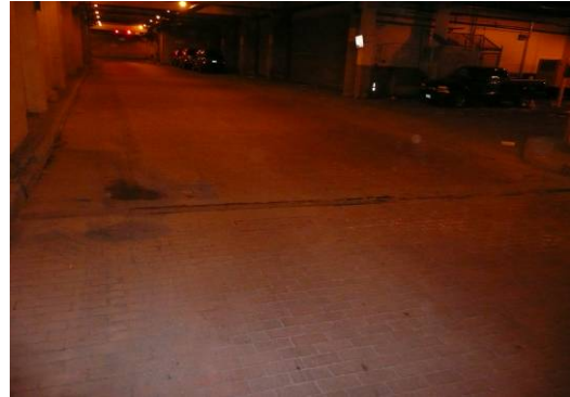
Floor drain in underground service tunnel
