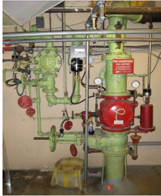
Fire system in basement of B. Forman Building
