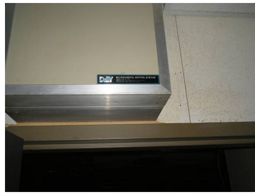
AC Unit on 14 th floor
