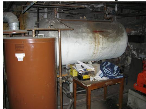
ACM wrapped water tank basement in B. Forman Building
