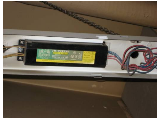
Light ballast in basement
