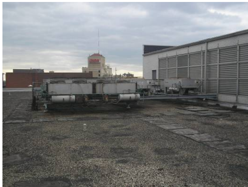
Equipment and penthouse on roof
