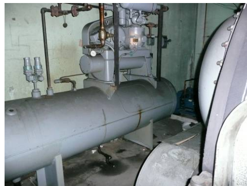
Chiller Equipment in sub-basement of McCurdy's
