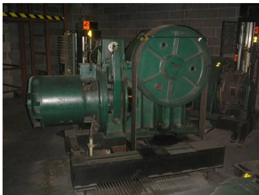
Elevator penthouse equipment
