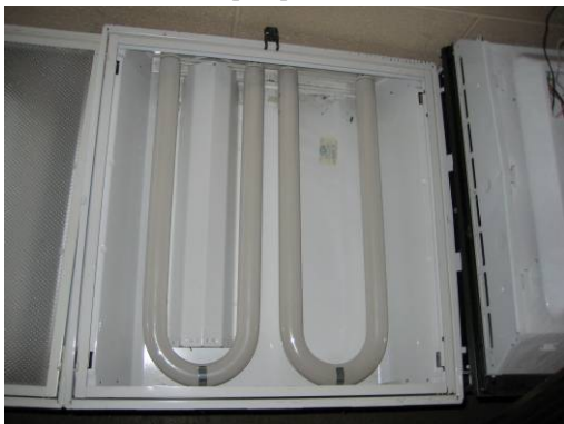
Fluorescent light fixtures in basement
