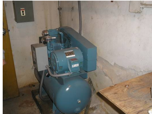
Compressor in basement
