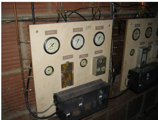
Panels in mechanical room in basement of B. Forman Building
