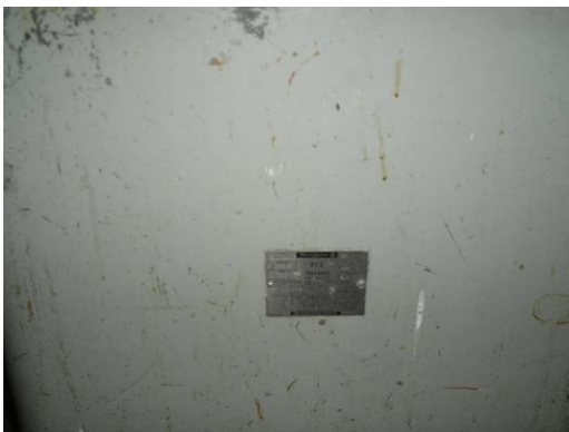
Transformer on 8 th Floor
