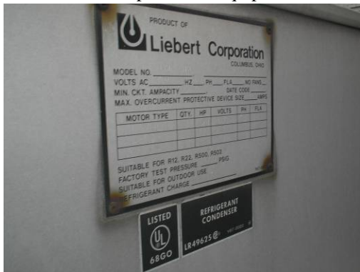
Refrigerant Condenser on roof
