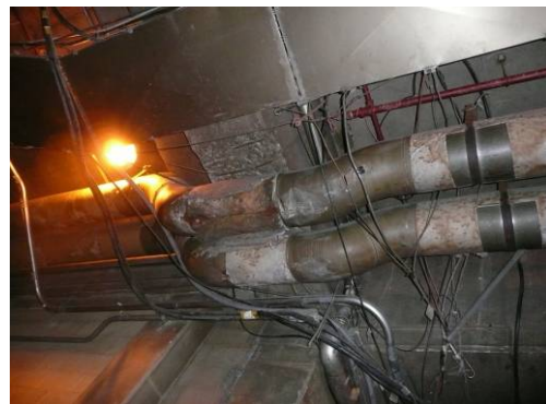
Utilities in underground service tunnel
