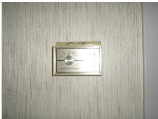
Thermostat on 6 th floor
