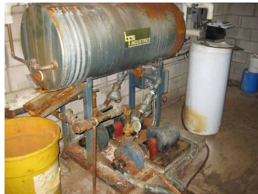
Descaling agent tank in boiler room
