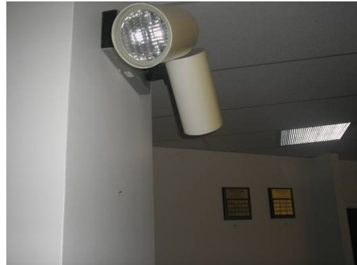
Emergency lighting on 3 rd floor
