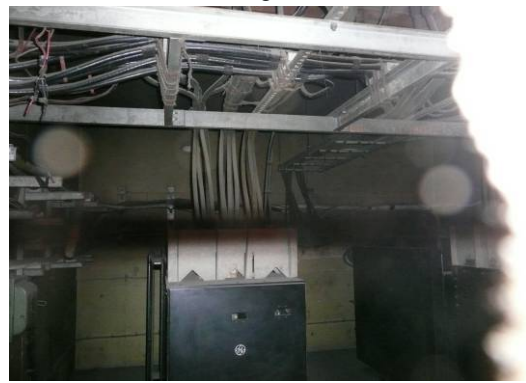
RGE transformer room in underground service tunnel
