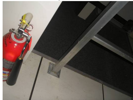
Fire extinguisher 6 th floor
