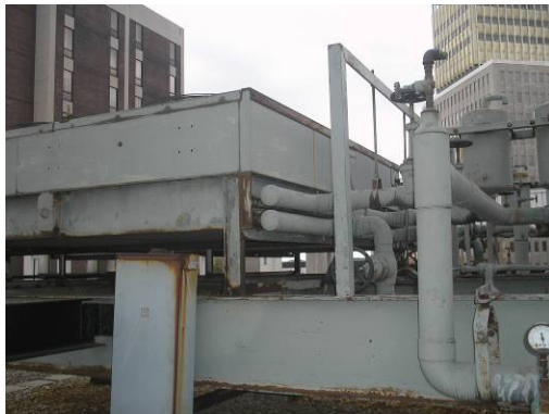
Cooling tower on roof
