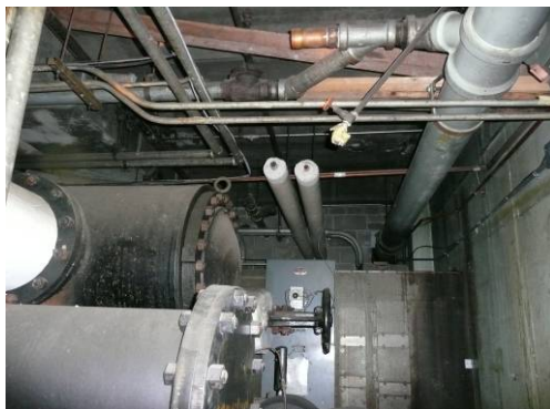
Chiller Equipment in sub-basement of McCurdy's
