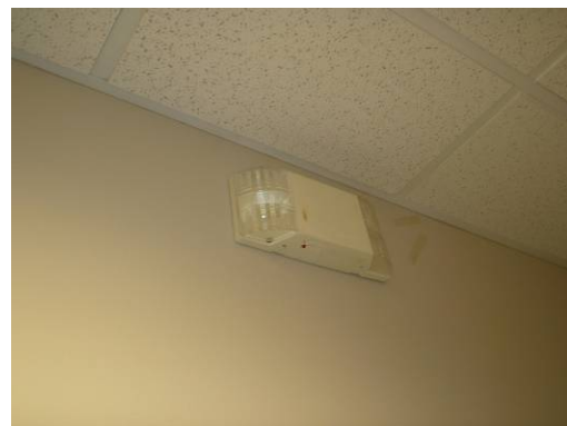
Emergency lighting on 3 rd Floor
