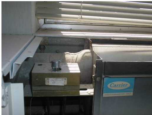
AC Unit on 13 th floor
