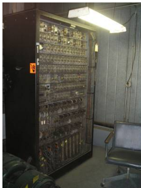
Elevator penthouse panel w/ capacitors
