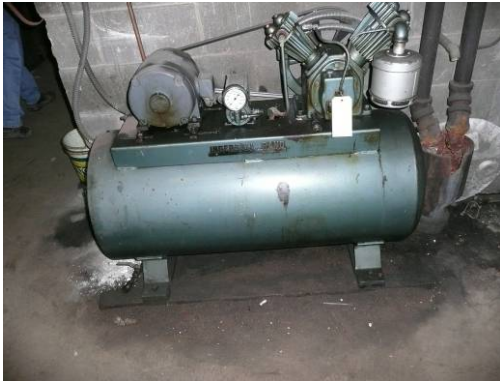
Compressor in sub-basement of McCurdy's Building
