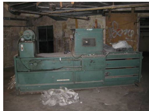
Box compactor in basement of B. Forman Building
