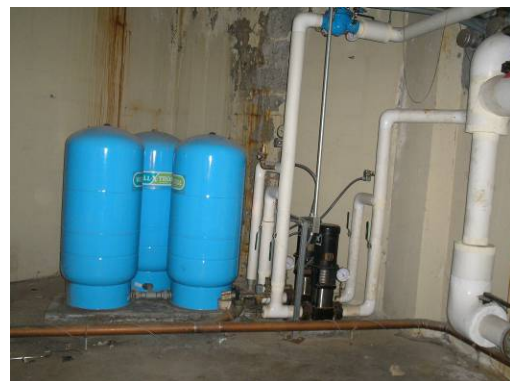
Water softener system
