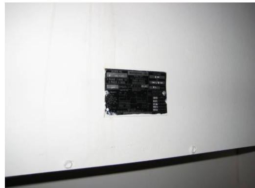
Transformer (dry type) on wall in basement
