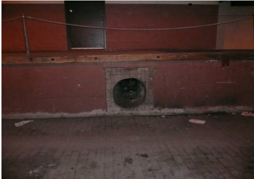
Tunnel pipe under loading dock of McCurdy's Building
