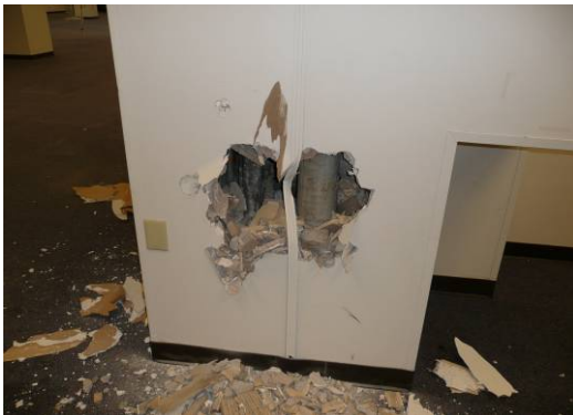
6 th Floor of B. Forman Building – vermiculite in wall
