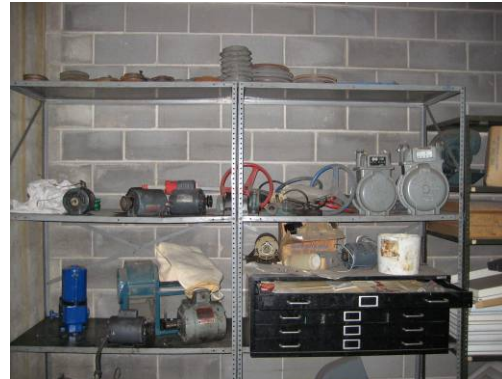
Electric motors and gas meters
