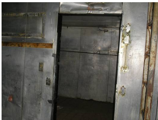
Equipment on 14 th floor
