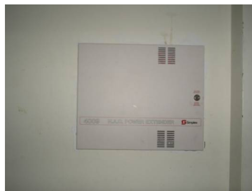
Power extender on 8 th floor
