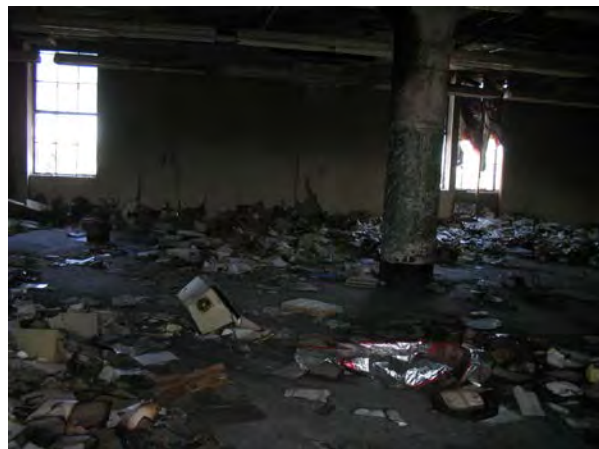
Photo No. 6 – Burned office materials following arson fire in 415 Orchard St. building, 2006.
