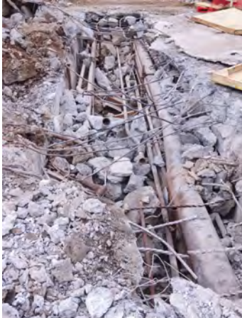
Photo No. 11: Asbestos containing pipe trench.
