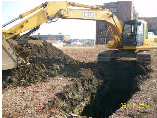
Photo No. 54 – View looking east at excavation of test pit TP-19 on berm, 2011.
