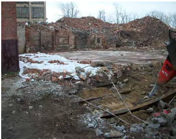
Photo No. 3 – AOC-1: Steel reinforced concrete over cap over Tank 9 vault (10,000 gal tank).
