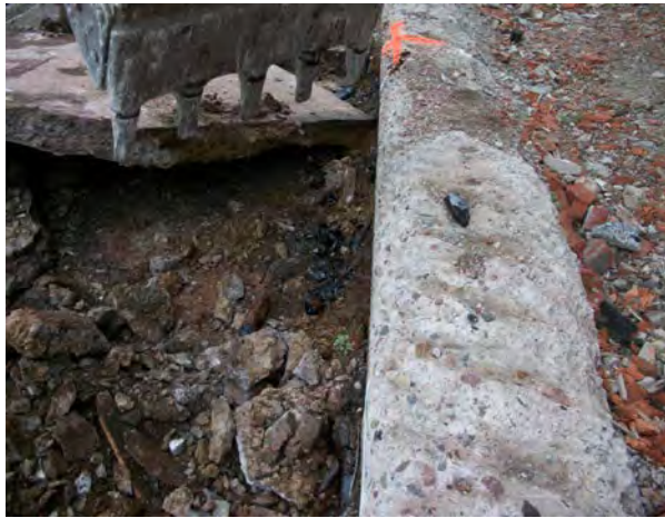
Photo No. 33- AOC-2: Concrete slab removal at SE corner plating area. Note UST vault wall.
