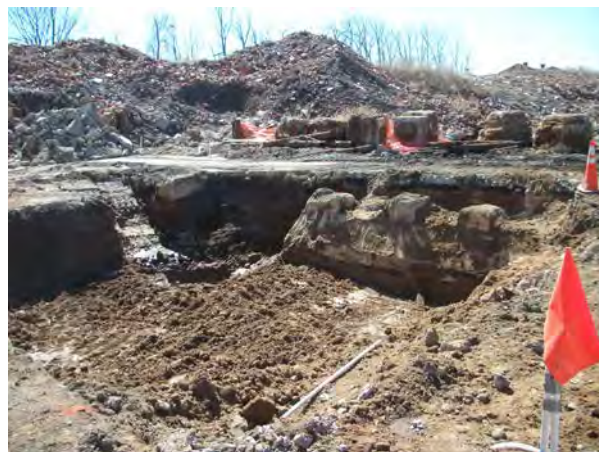
Photo No. 42- AOC-2: Looking southwest from northeast corner at buried concrete footer structure.
