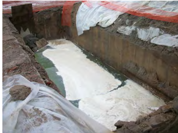
Photo No. 20 – AOC-1: Tank 9 Vault full of chromium-impacted water from tunnel
