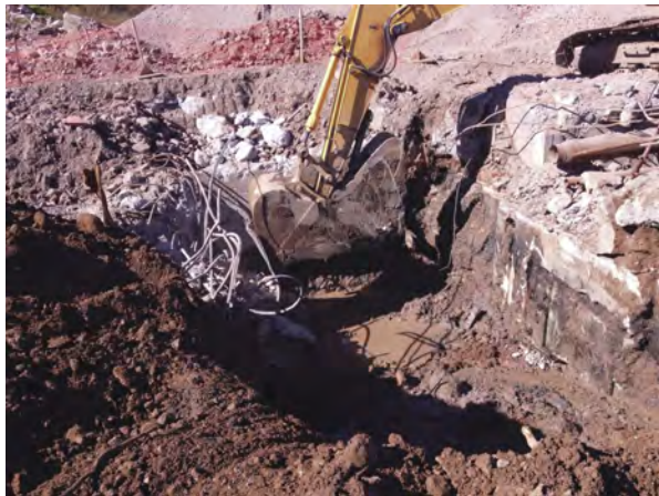
Photo No. 21: Groundwater infiltration.
