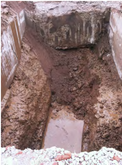
Photo No. 9: Groundwater entering test pit.
