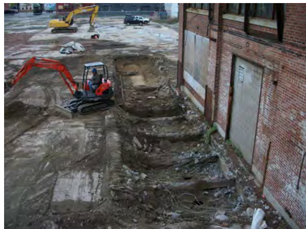
Photo No. 6 – AOC-1: View looking north at uncovered UST farm and vault system.
