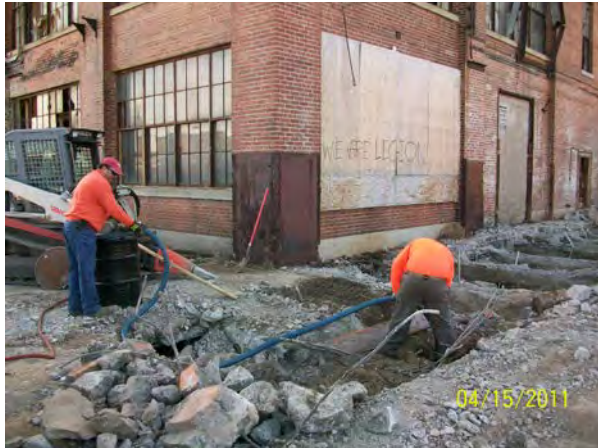
Photo No. 13 – AOC-1: Looking southeast at TREC removing waste product with drum vac..
