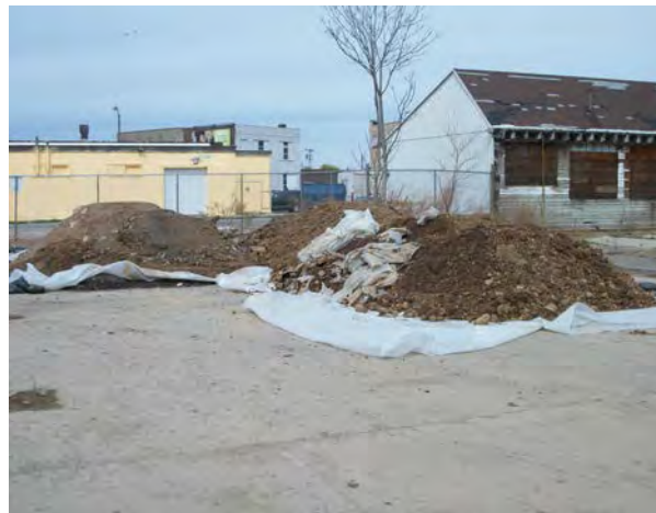
Photo No. 40 – AOC-2: Stockpiling of contaminated soil on northern portion of Site.
