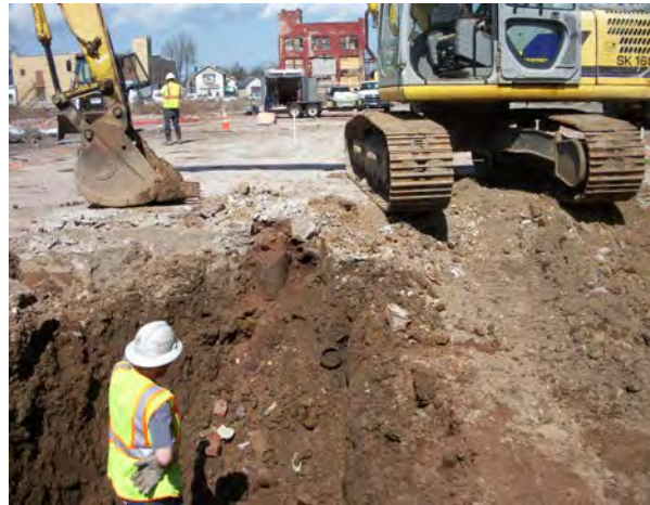
Photo No. 34 – AOC-2: Initial soil removal in plating area. VCT crock being removed, center.
