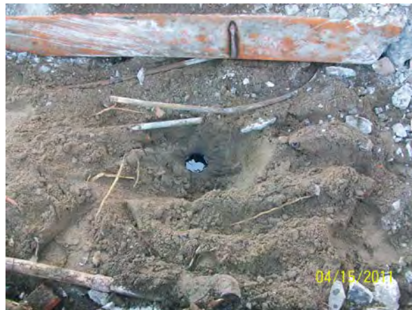
Photo No. 12 – AOC-1: Uncovering Tank 7. Note it is full of product.
