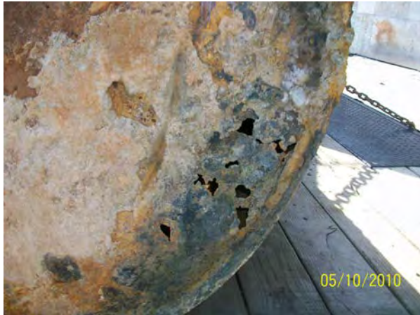
Photo No. 19 – AOC-1: Tank 7 rust holes.
