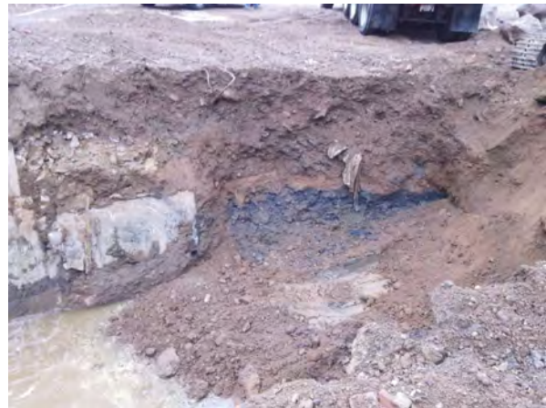
Photo No. 22: Petroleum contamination.
