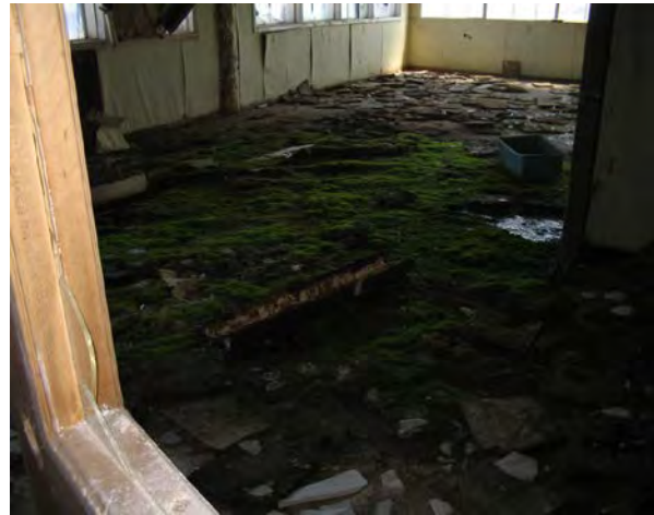
Photo No. 4 – Moss growing on interior floor of 415 Orchard St. building, 2006.
