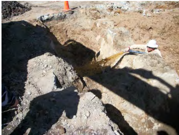
Photo No. 45– AOC-2: View of remedial molasses mixture being applied to exposed soil.
