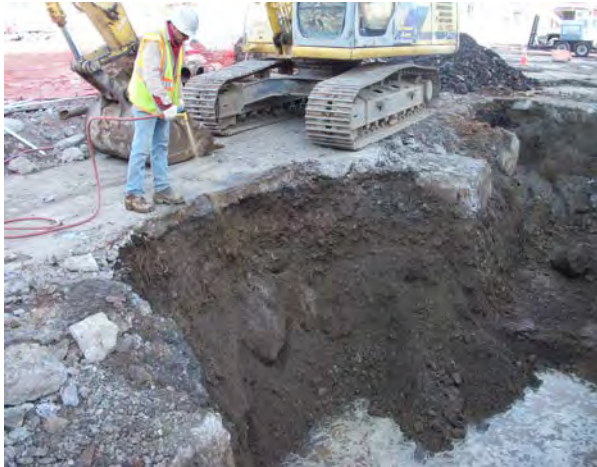
Photo No. 37 – AOC-2: Applying remedial molasses solution to west wall of excavation.
