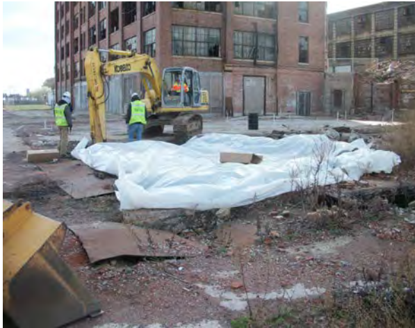
Photo No. 25 – AOC-2: Looking east;OPTECH laying out poly to hold concrete chimney base contents.
