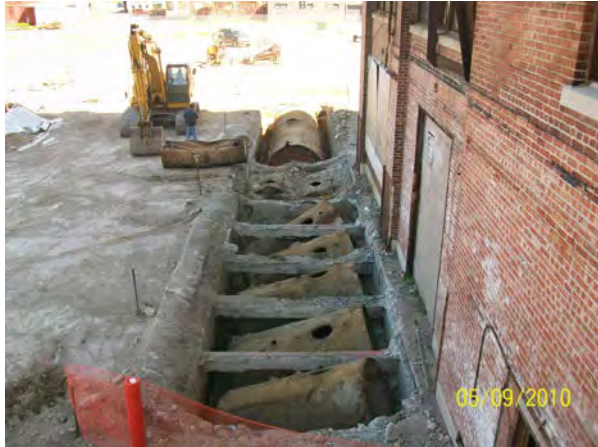
Photo No. 51 – View of 9 USTs contained within concrete vault system, 2011.
