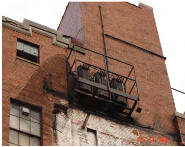
Photo No. 10. – 3 electrical transformers mounted on south wall of 415 Orchard St. building, 2006.
