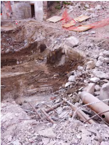
Photo No. 15: Example of encountered subterranean contents. Sheet piling, concrete piling, concrete walls, and pipes.
