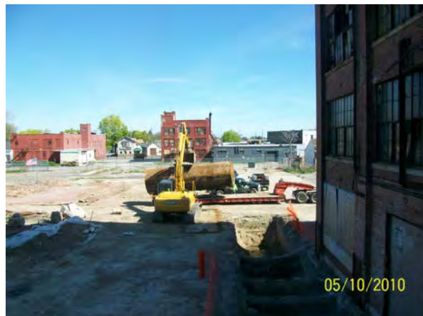
Photo No. 18 – AOC-1: Removing 10,000-gal Tank 9 and placing on trailer for disposal.
