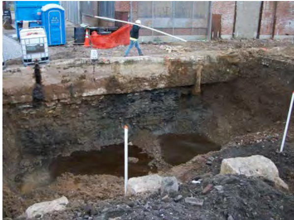
Photo No. 49 – AOC-2: Exposed east wall of plating area/Tank 9 vault wall after molasses.
