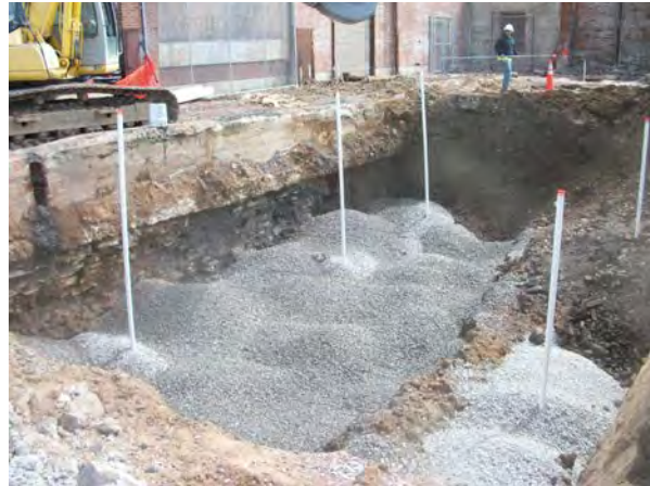
Photo No. 50 – AOC-2: View to south at backfilled wells with clean stone fill.
