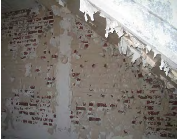
Photo No. 7. – Peeling interior paint during lead survey in 415 Orchard St. building, 2006.
