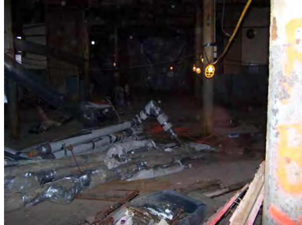
Photo No. 14 – Asbestos-containing piping during 354 Whitney St. abatement, 2008.
