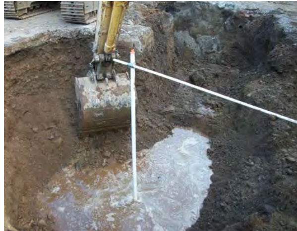
Photo No. 38 – AOC-2: Installing backfill well PA-09 in western portion of excavation.
