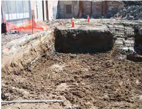
Photo No. 43 – AOC-2: Looking south at PA-14 area. Note concrete wall of Tank 9 vault.
