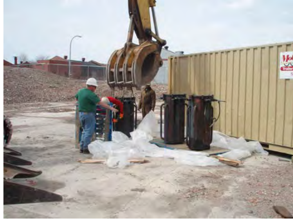
Photo No. 20 – Transformers from 415 Orchard St. building staged for disposal, 2008.
