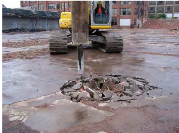
Photo No. 38 – Hoe-ram breaking concrete slab at floor drain for test pit access, 2008.
