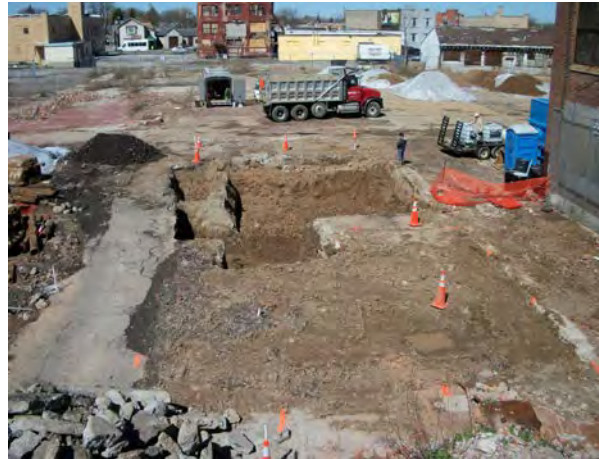
Photo No. 44 – Looking north at northern half of open excavation & staged soil piles.
