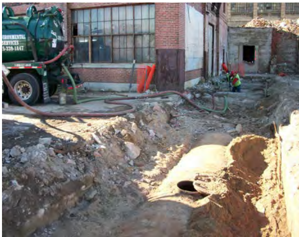
Photo No. 9. – AOC-1: View looking south at UST product removal by Egan Env.
