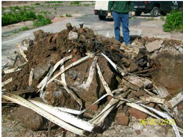
Photo No. 57– View of solid waste and fill materials in vehicle lift vault.
