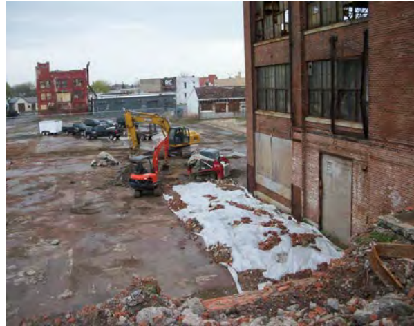
Photo No. 2 - AOC-1: Concrete removal at Tank 9 vault and poly cover over UST vaults.
