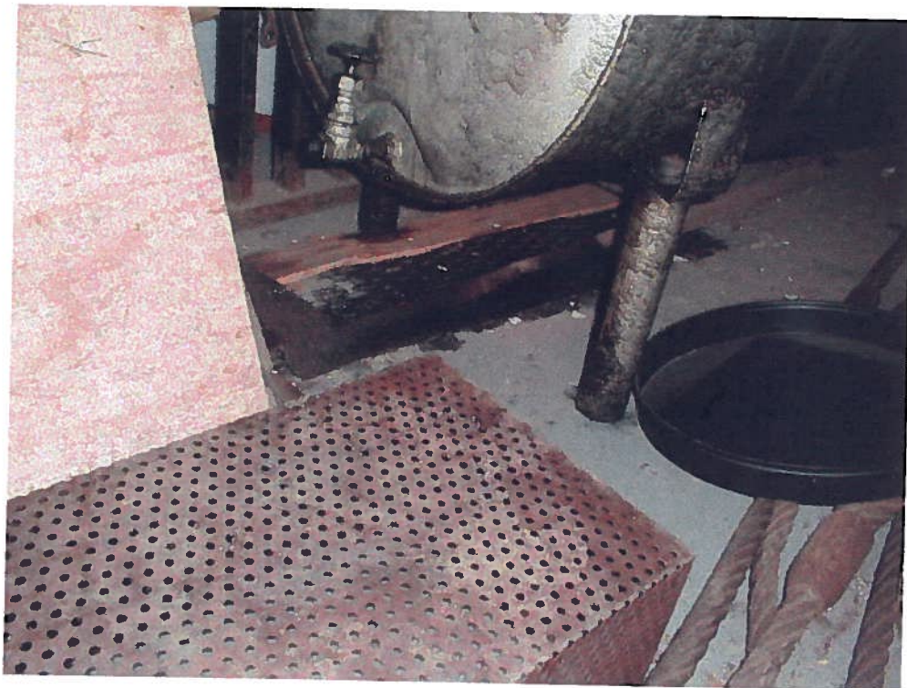
367 Orchard Street; stain beneath the AST
