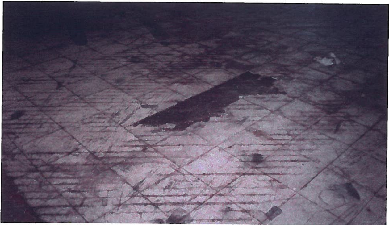
354 Whitney Street; damaged 12"x12" floor tiles determined to be asbestos-containing material through testing
