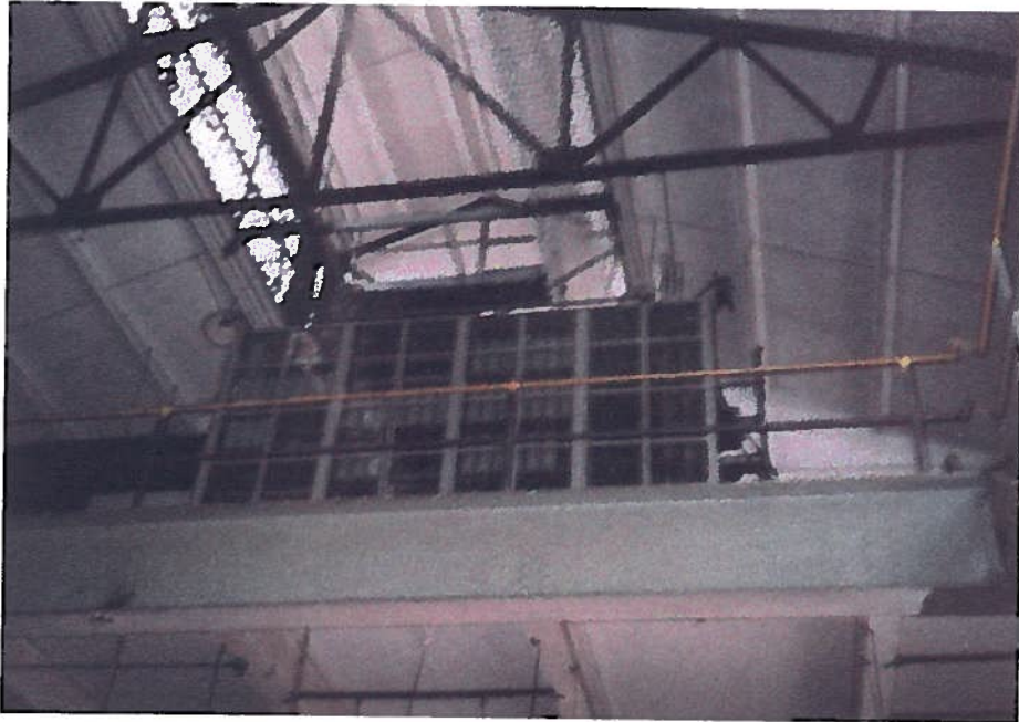
354 Whitney Street; view of electrical equipment in engine room in east wing of building
