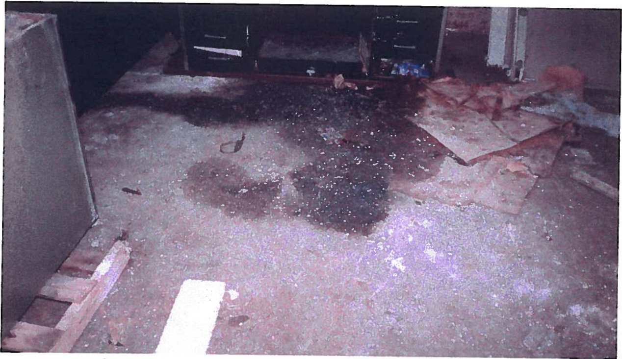
354 Whitney Street; staining on concrete floor on first floor
