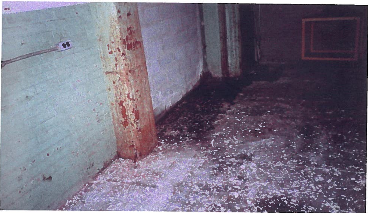
354 Whitney Street; staining on concrete floor in first floor tunnel area where USEPA removed drums and containers
