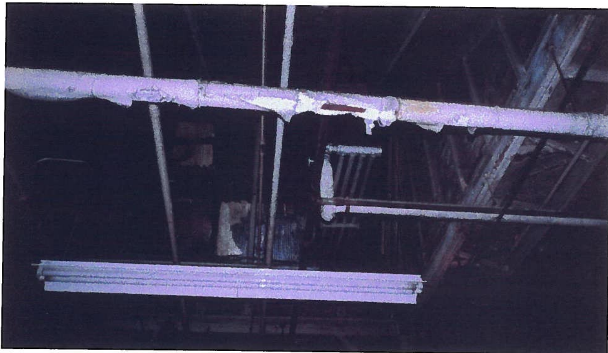
367 Orchard Street; damaged suspect asbestos containing material
