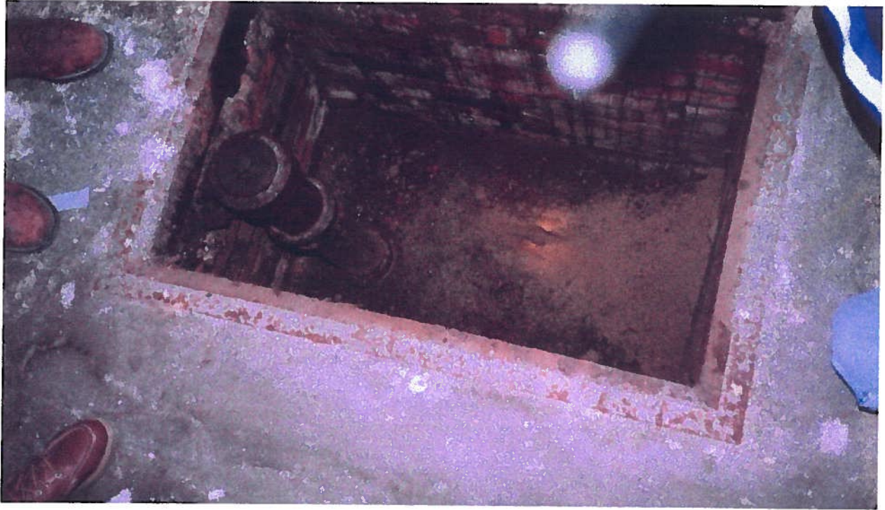
415 Orchard Street; brick-lined pit with metal plate cover housing apparent pipe cleanout
