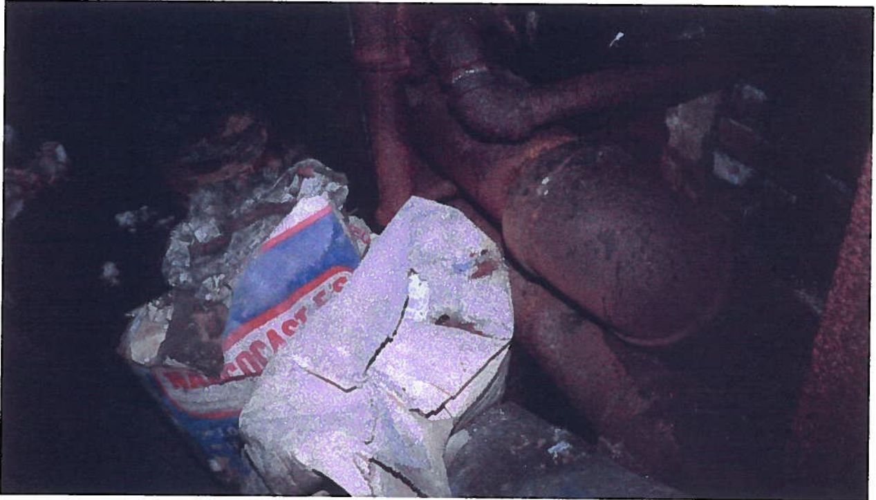
354 Whitney Street; bags of suspect asbestos-containing pipe mudpack material located south of boiler room
