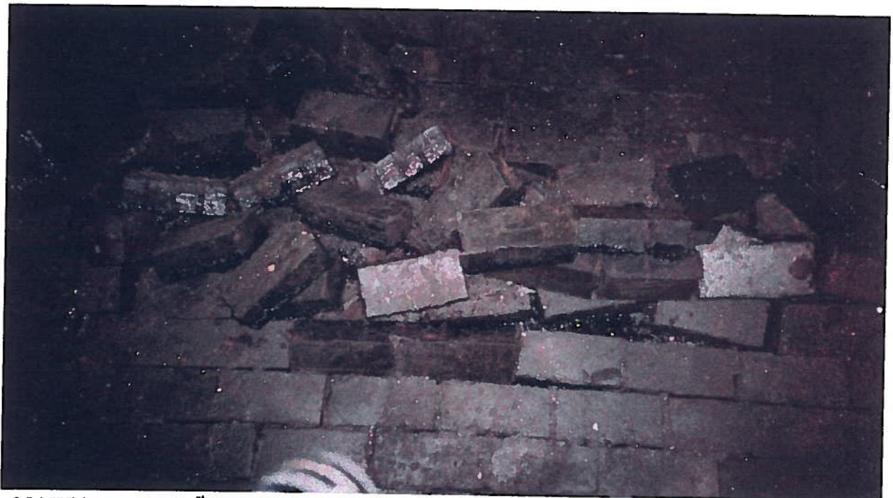
354 Whitney Street 1 st Floor – damage to floor that has exposed apparent petroleum-based (tar-like) mastic.
