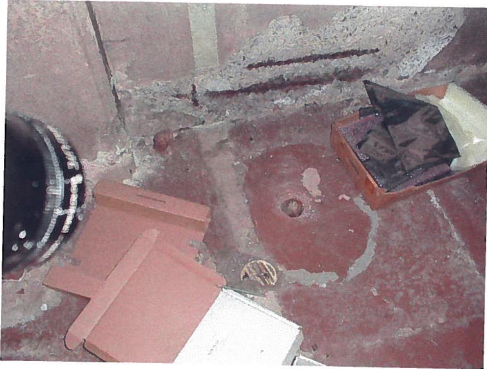
367 Orchard Street; floor drain, 1 st floor
