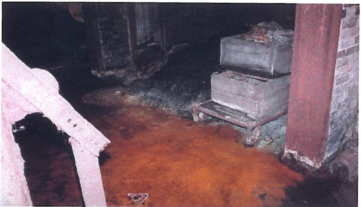
354 Whitney Street; view of apparent coal pile and orange leachate in south end of boiler room
