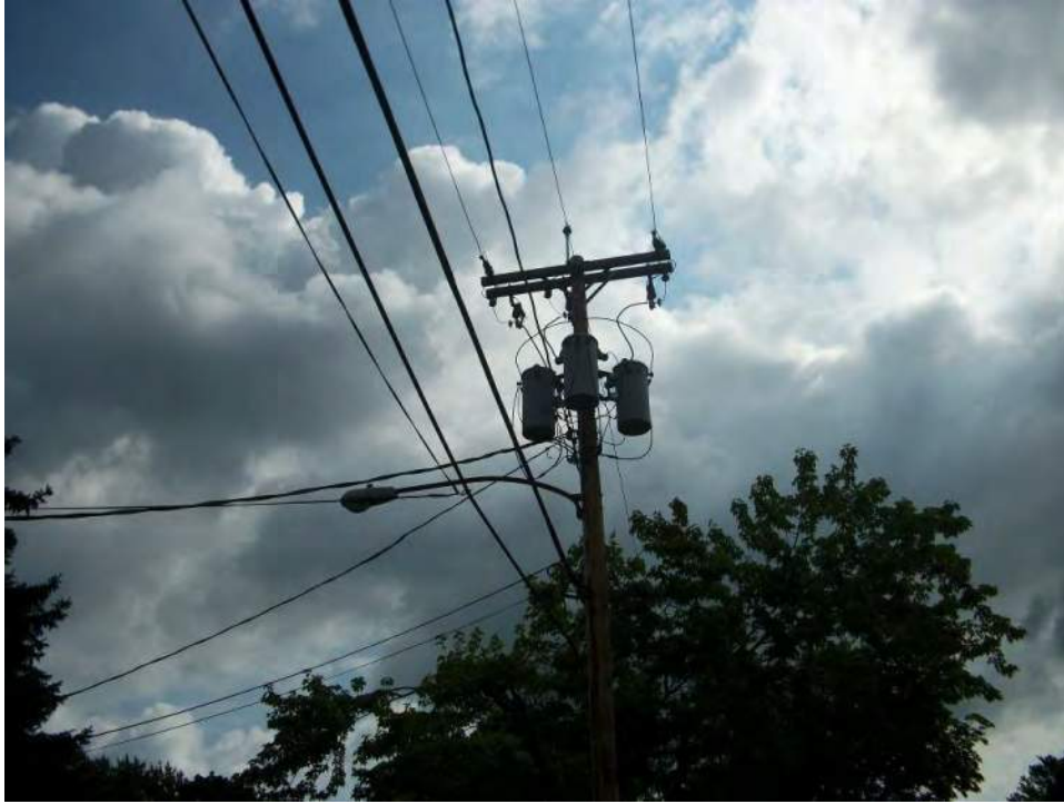
View of RG&E pole-mounted transformers located near the northeast property corner along Sullivan Street.
