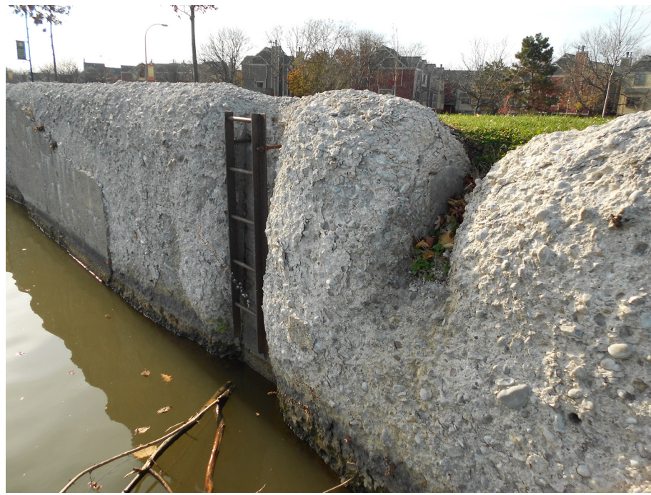
VIEW OF WALL SHOWING CONCRETE IN POOR CONDITION
