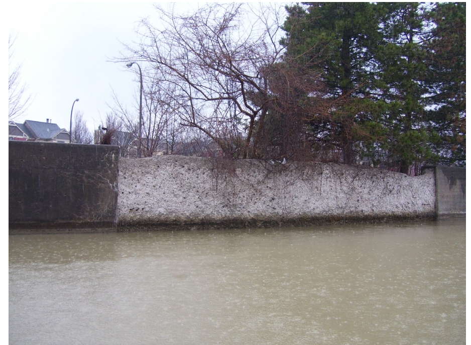
VIEW OF WALL SHOWING CONCRETE IN POOR CONDITION
