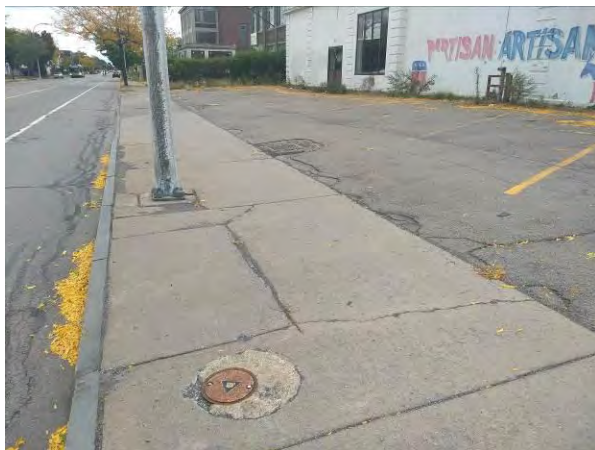
Photo No. 11 Monitoring well in sidewalk of 1185-1223 E. Main Street looking east; and location of former USTs.
