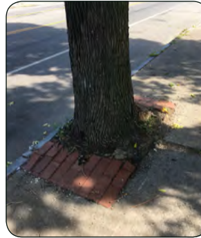
Special Condition Photo: Tree grate grown into root flare
