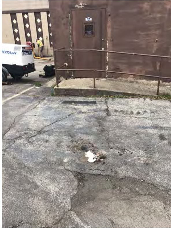
Temporary monitoring well TMW-12-24 in foreground, hand clearing utilities with compressed air knife system at test location TB/TMW-05-32 in background – looking northeast
