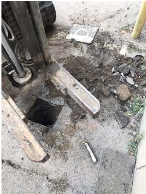
Set up track-mounted Geoprobe direct-push drill-rig at test location TB/TMW-05-32 that was hand-cleared of buried utilities to depth of approximately 4 feet.
