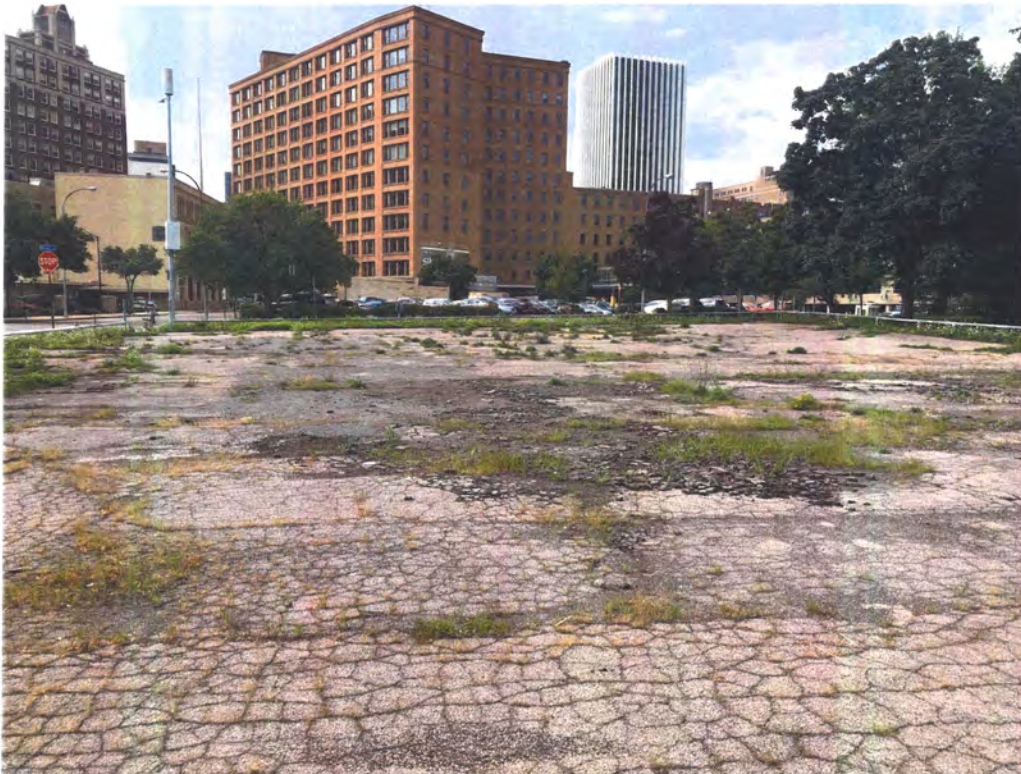
The central portion of the parking lot on the assessed property looking south on 8/27/2018.
