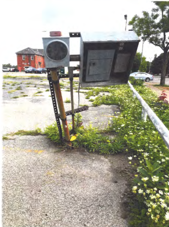
Electrical equipment located along the southeastern edge of the assessed property looking north.
