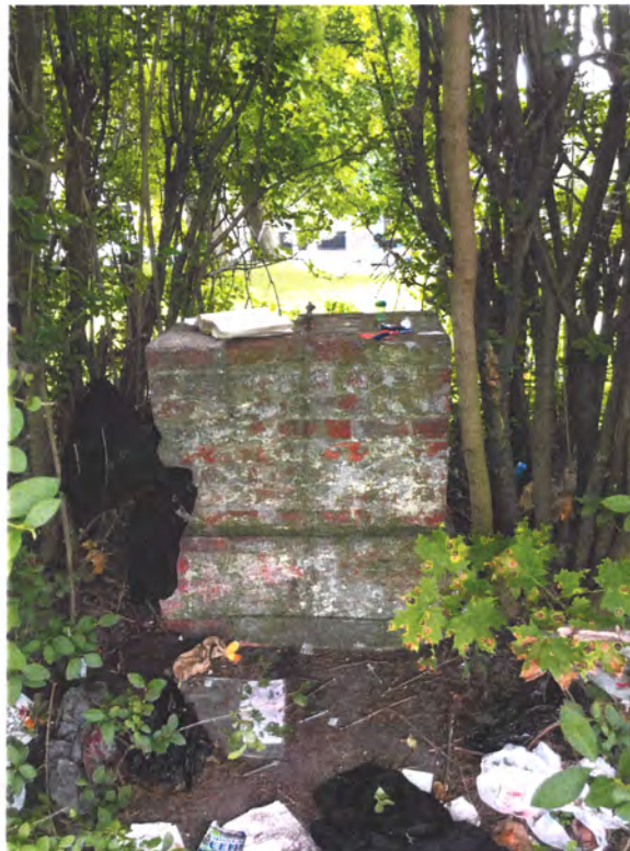
Brick monument of unknown use in treed hedgerow on the southcentral portion of the assessed property looking southwest.
