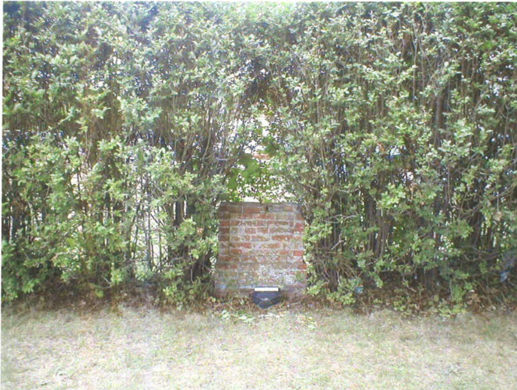
View of a brick structure located on the southwest portion of the assessed property.
