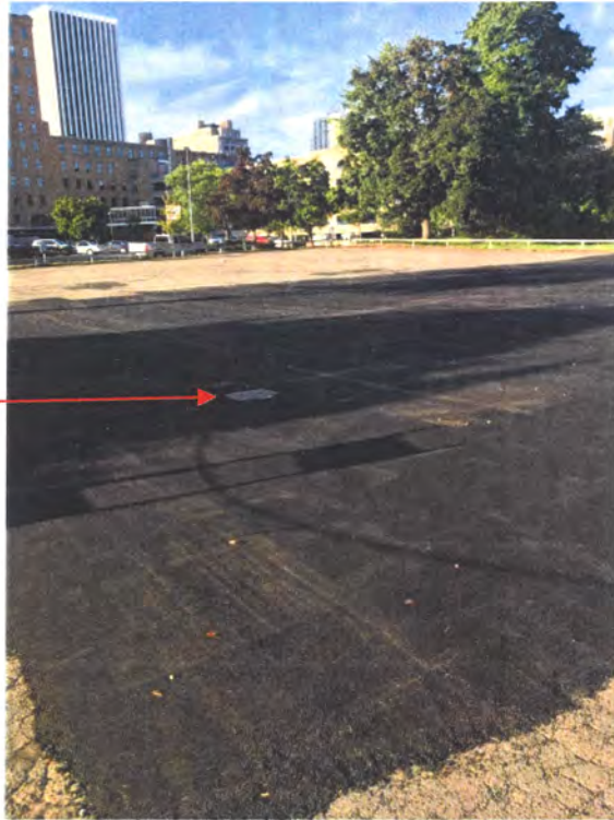
View of newly paved asphalt (observed during the 9/17/2018 site visit) in the central portion of the parking lot on the assessed property looking southwest. The catch basin is also visible.
