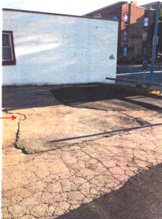
View of an approximate 8' x 12' rectangular-shaped asphalt patch in the parking lot on the northeastern portion of the assessed property, which could be associated with a former UST, looking northeast.
