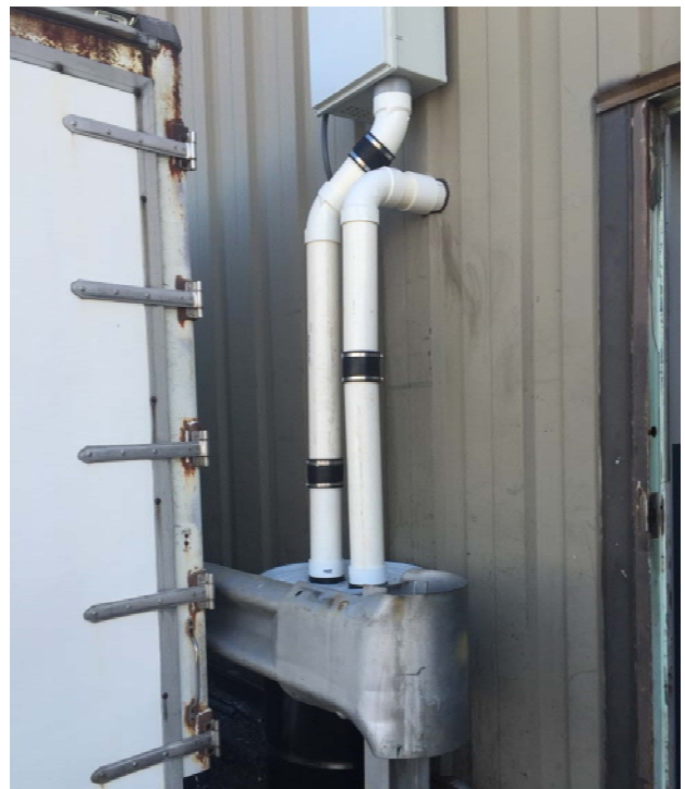
Exterior piping, knock-out tank and fan (April 2017)
