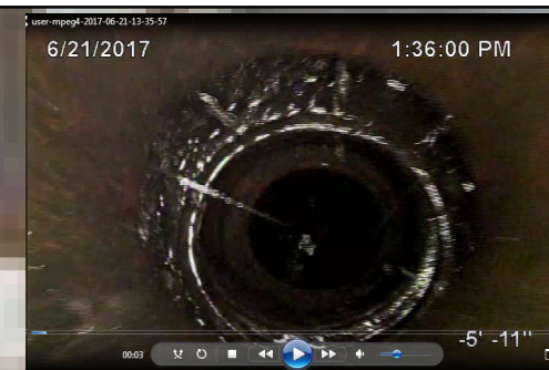
Typical break in vertical piping (locations 1, 2, 3, 4, 8, 10)
