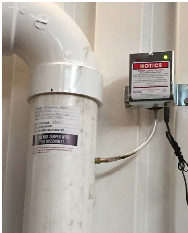
Alarm and labeling (March 2017)
