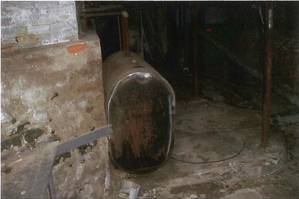
Property #84 (24 West Avenue) - View of heating oil AST in basement of building.
