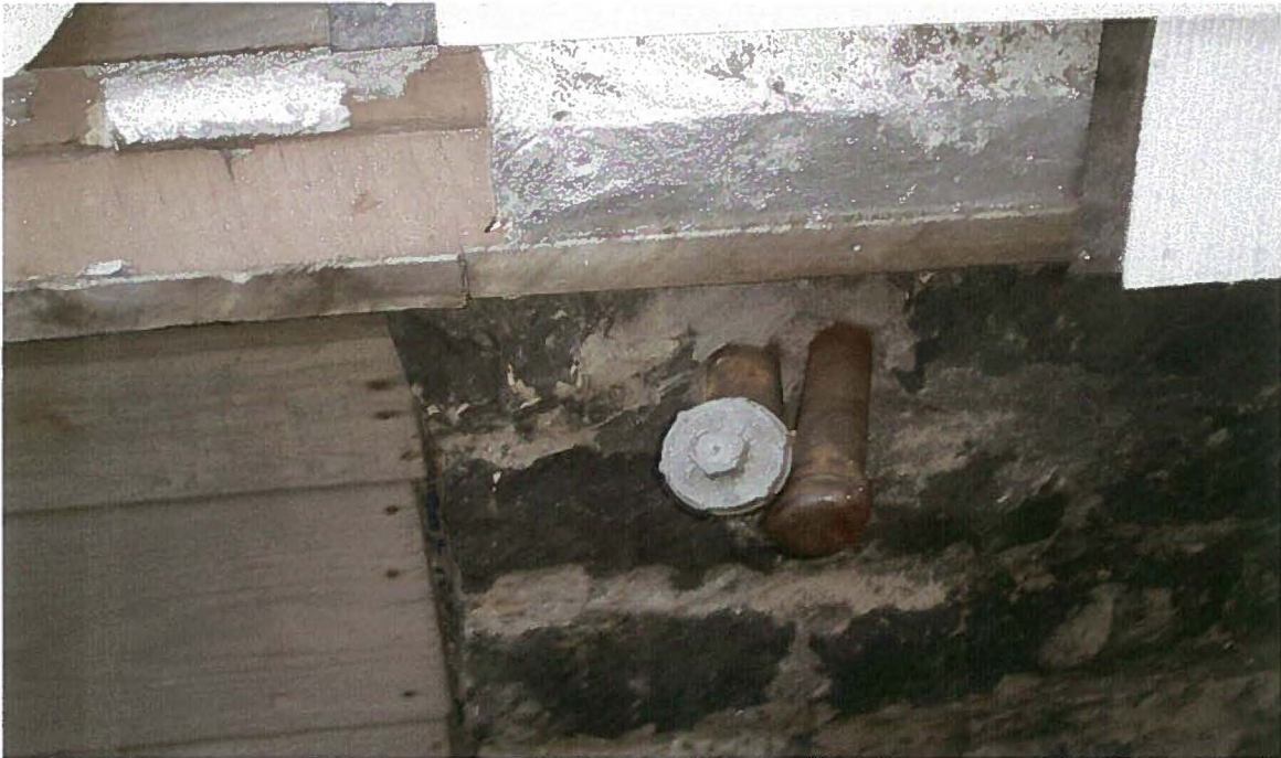
Property #58 (4 Kensington Street) - View of vent and fill pipes associated with apparent residential heating oil tank.
