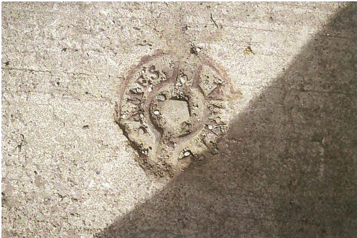
Property #71 (239 Silver Street) - View of potential fill port in sidewalk surface in front of property.
