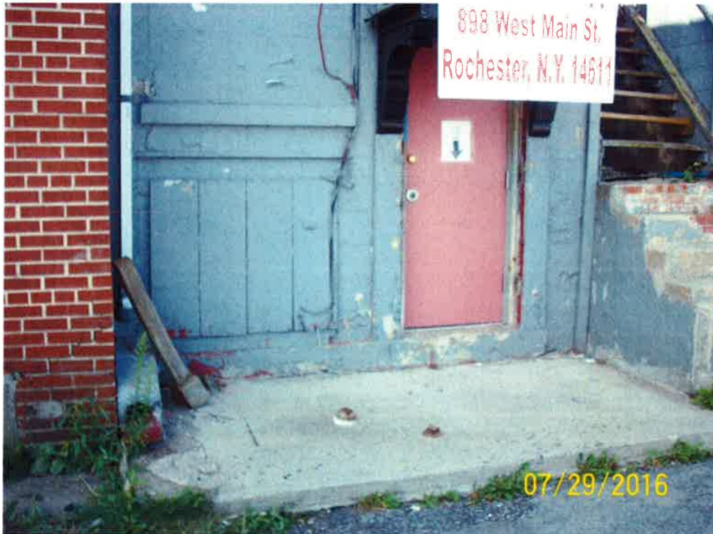
View of the rear (northern portion) of the 898 W. Main Street part of the assessed building.
