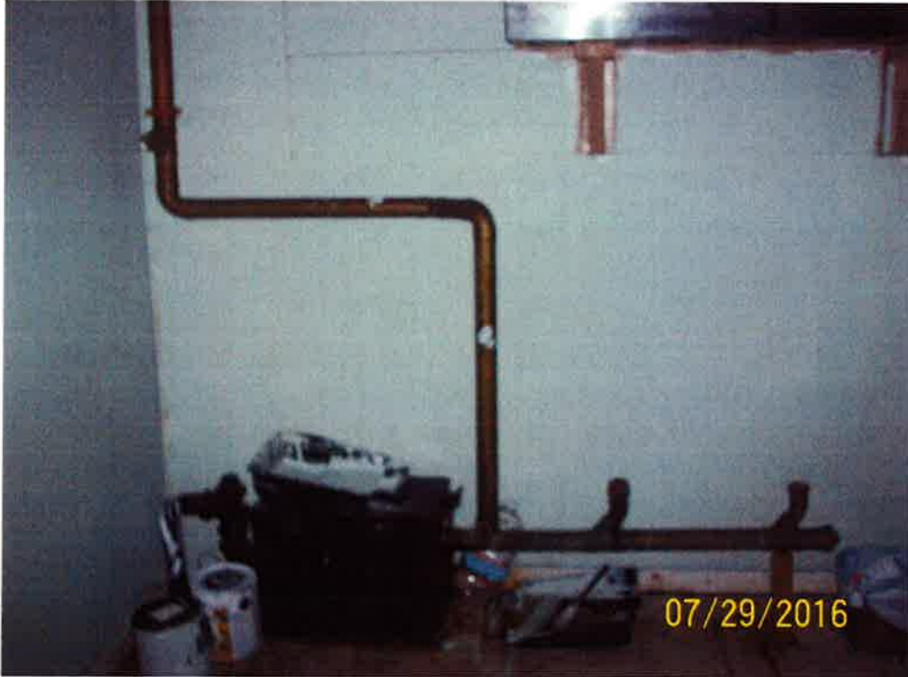
View of the grease trap located in the kitchen of 898 W. Main Street (Mosque) portion of the assessed building.
