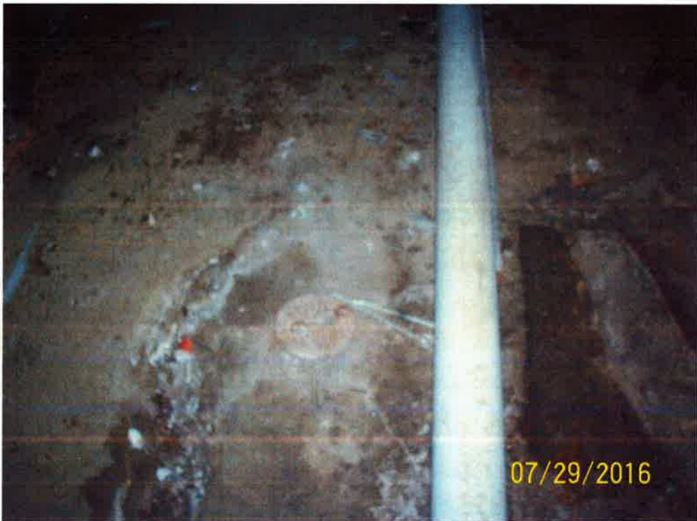
View of a two-holed apparent water well cap located in the basement of the assessed building.
