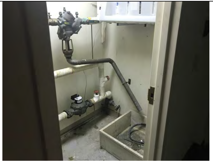
Mop sink and associated floor drain in Section 3
