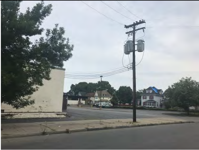
Pole-mounted transformer located on the southeastern Site boundary
