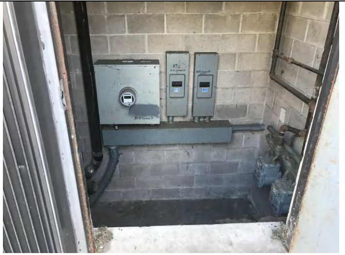
Typical view of the utility room on the western portion of the Site Building (Section 2)
