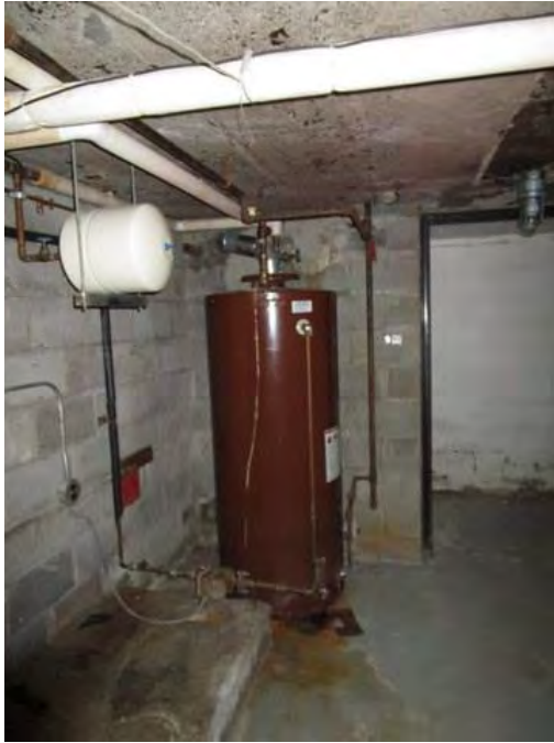
Water heater in basement
