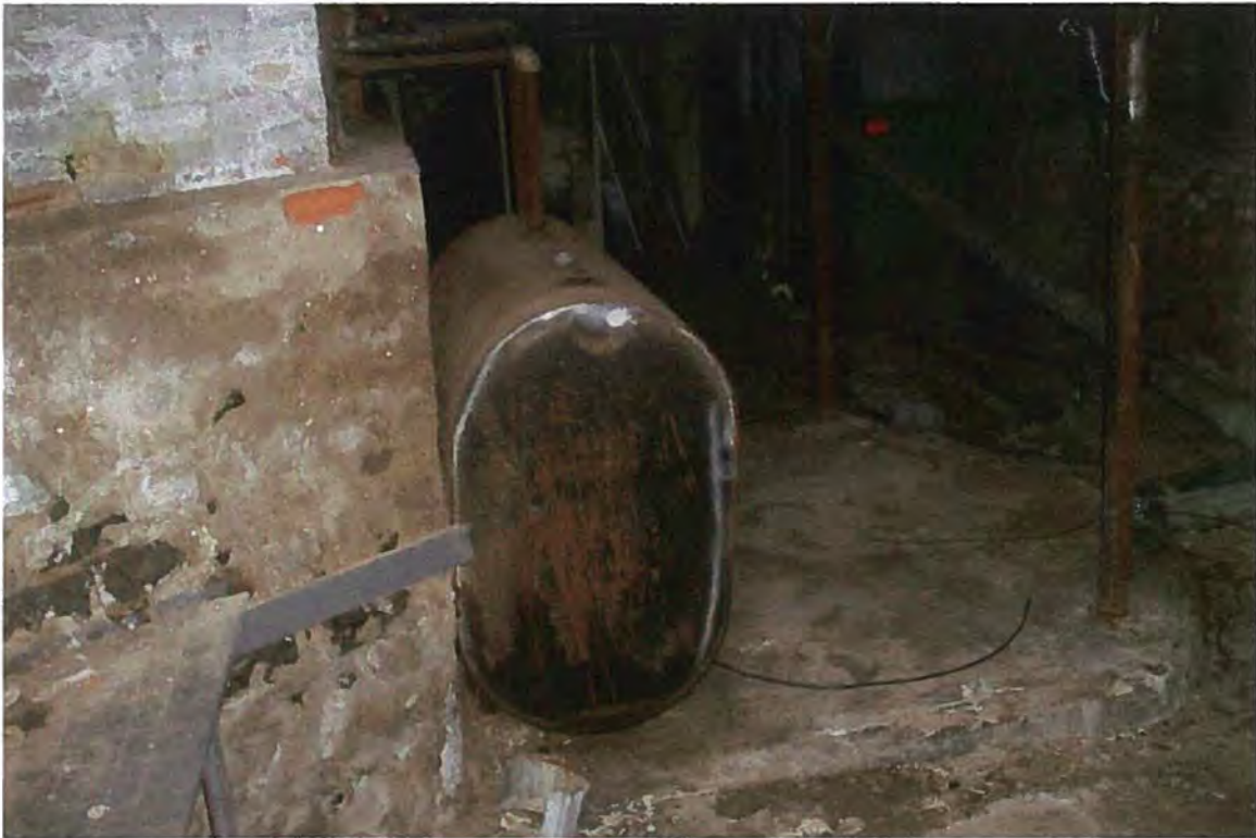
Property #84 (24 West Avenue) - View of heating oil AST in basement of building.
