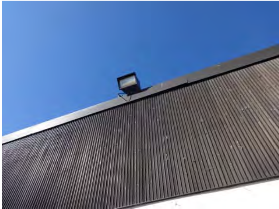
Building mounted lighting
