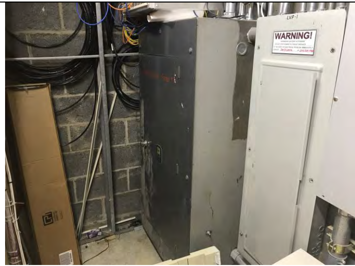
Representative distribution panel located on the second floor of Section 7
