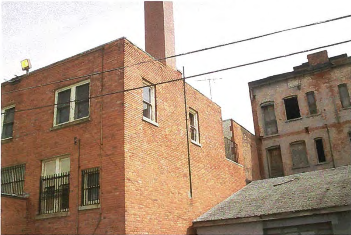
Property #74 (888-892 West Main Street) - View of vent pipe located on the west side of property.
