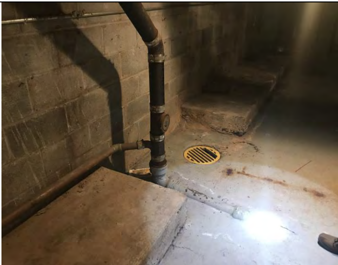
Representative floor drain in the basement of Section 9
