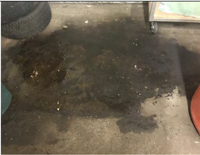
Apparent staining in Section 6
