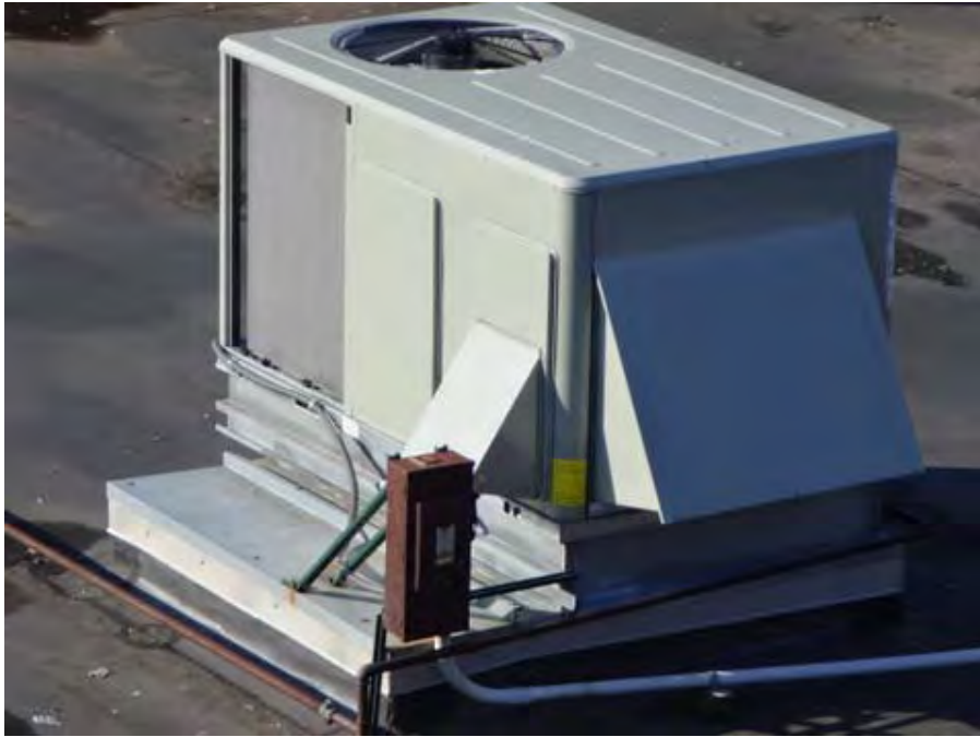
Rooftop packaged HVAC units
