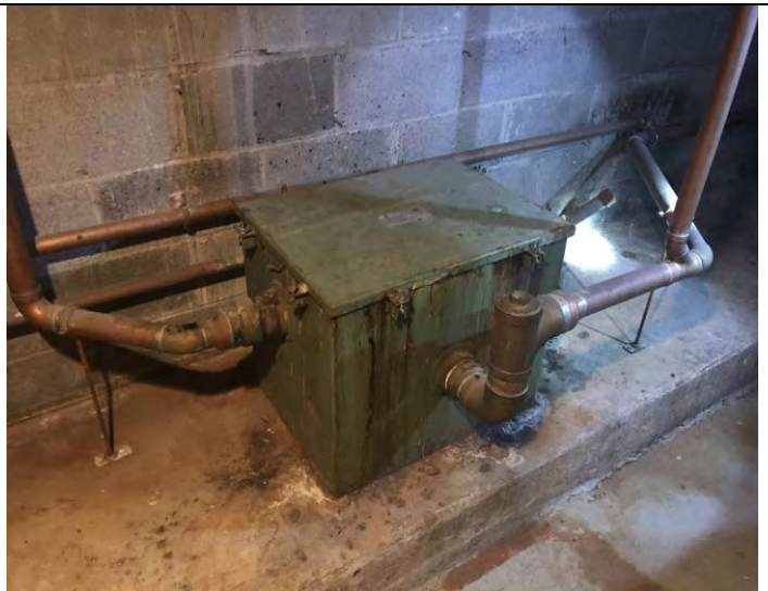
Typical view of the grease trap in the basement of Section 9
