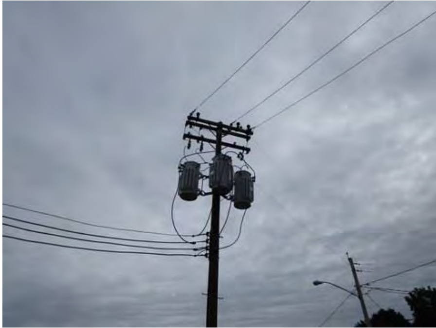
Pole-top electrical transformer
