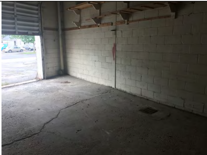
Typical view of floor drains in loading dock area in Section 8
