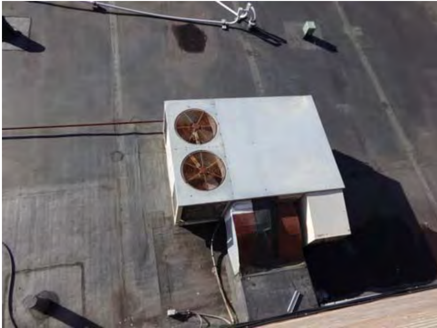
Rooftop packaged HVAC units
