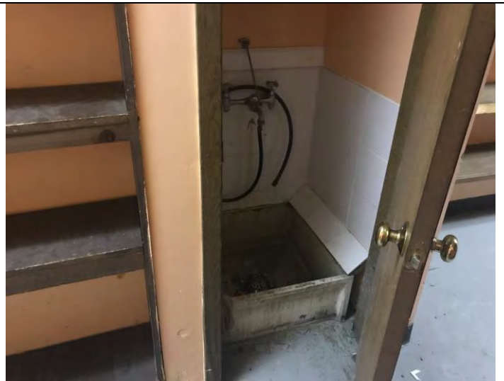
Mop sink and associated floor drain in Section 9
