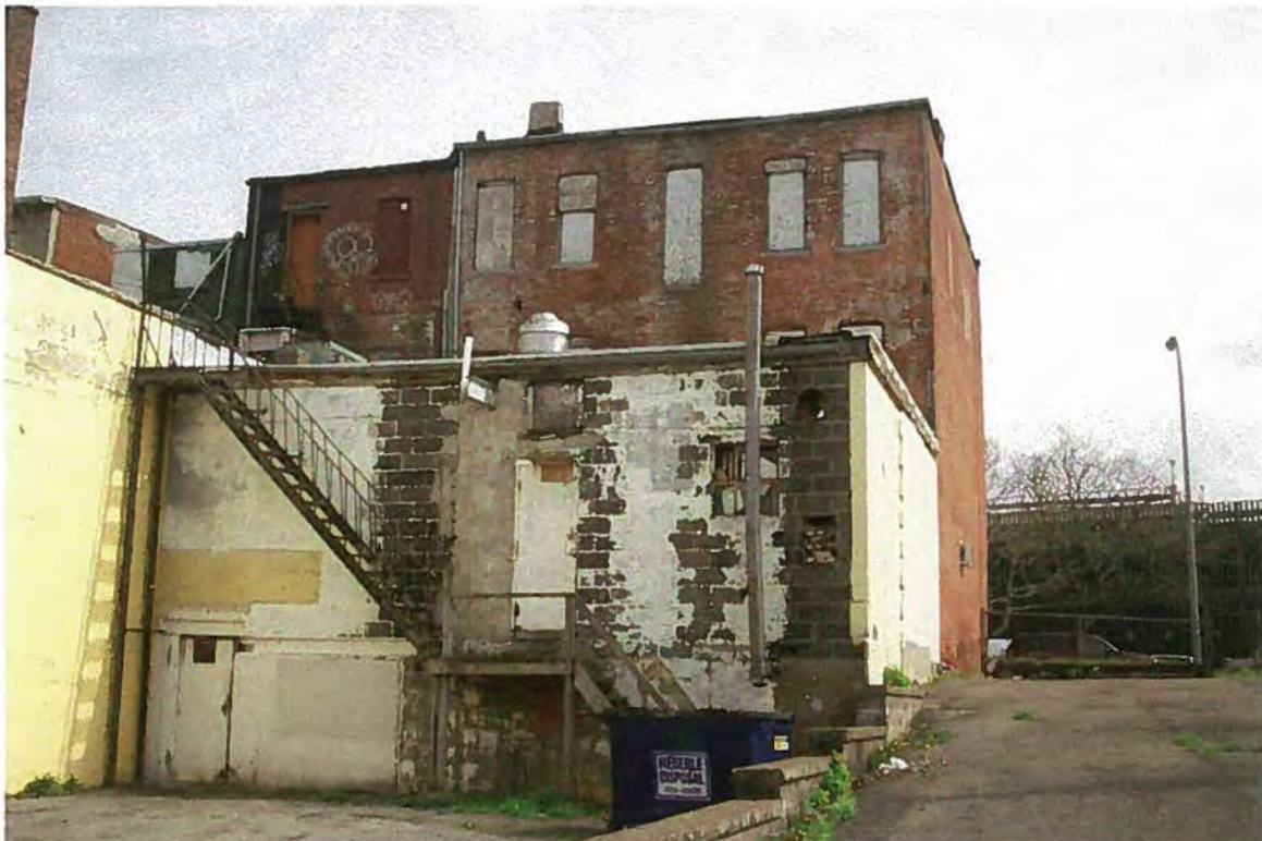
Property #78 (906-910 West Main Street) - View of two vent pipes on north side of building.
