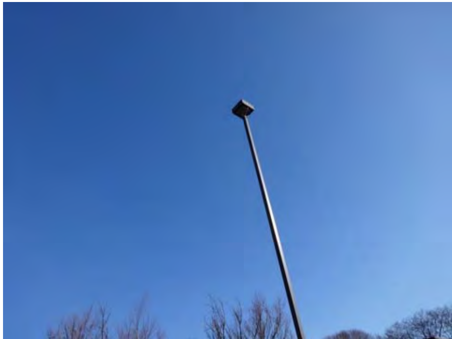
Pole top lighting
