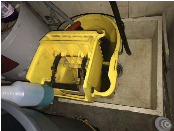
Mop sink and associated floor drain located on the first floor of Section 7
