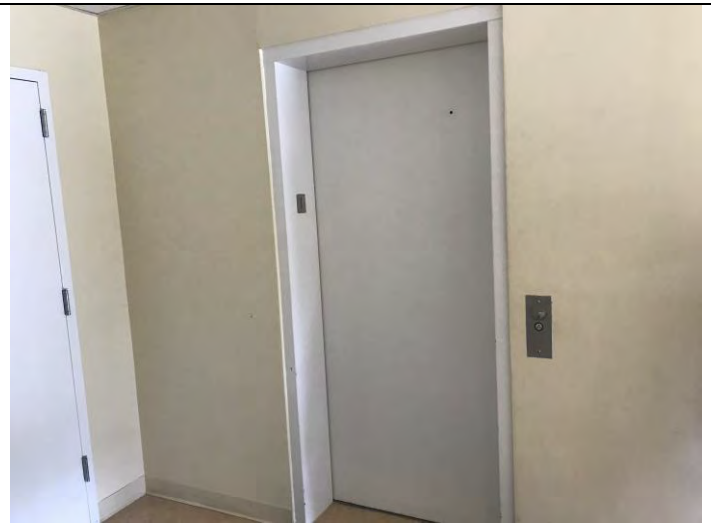
Typical view of the elevator in Section 7
