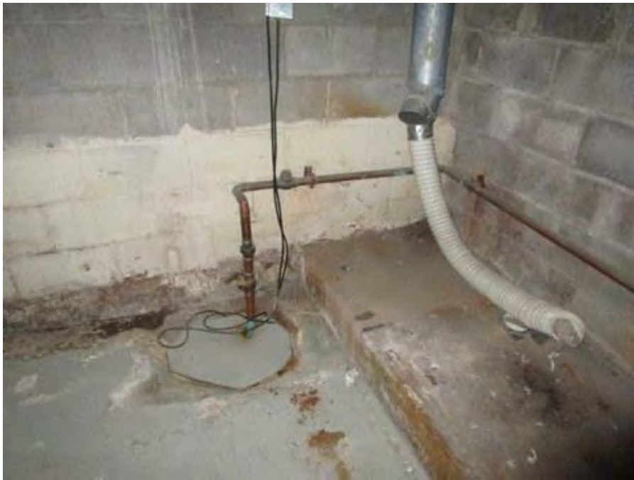
Sump pump in basement
