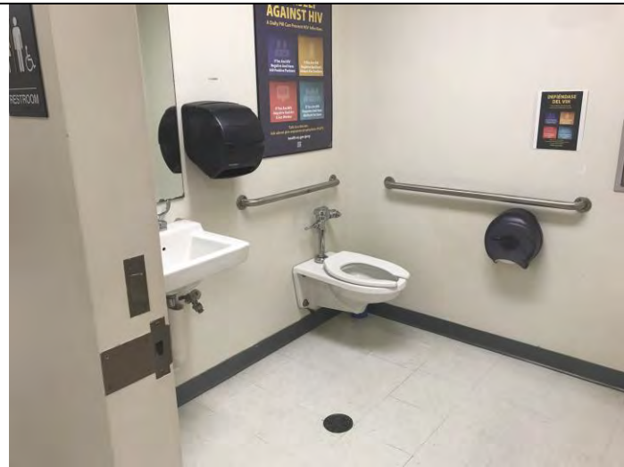
Representative restroom and associated floor drain located on the second floor of Section 7
