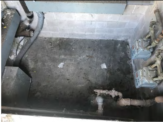
Typical view of the utility room on the western portion of the Site Building (Section 2)
