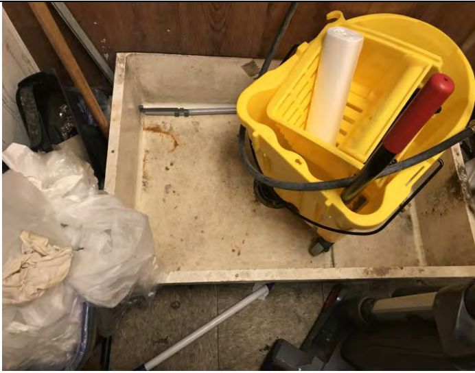
Mop sink and associated floor drain in Section 4
