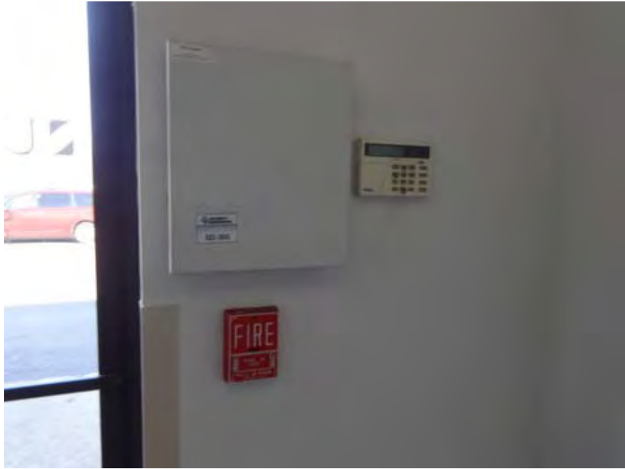
Fire and security systems
