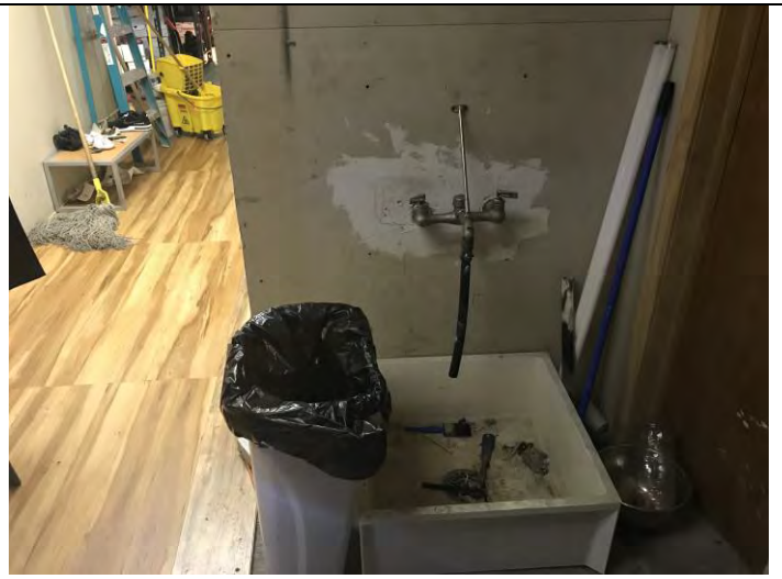
Mop sink and representative floor drain in Section 1
