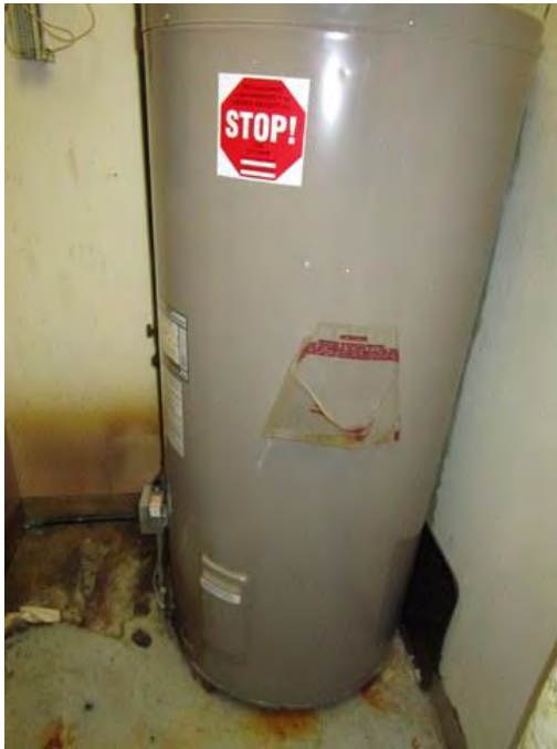
Typical tenant water heater
