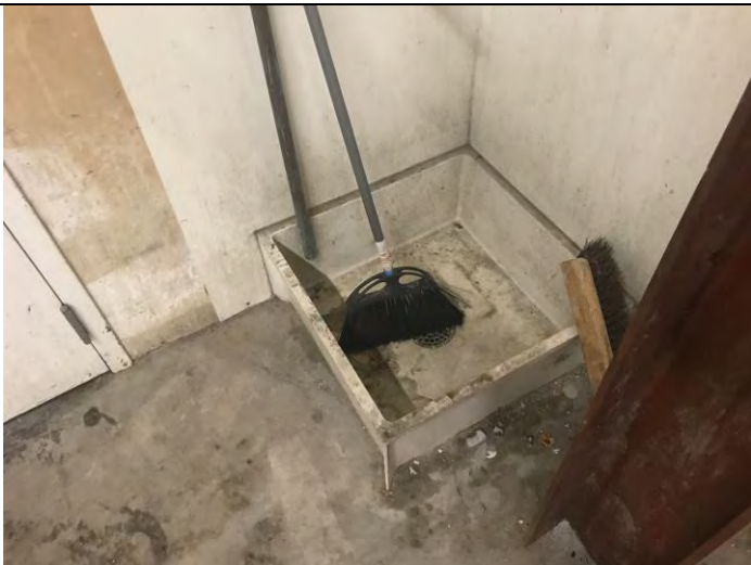
Mop sink and associated floor drain in Section 5
