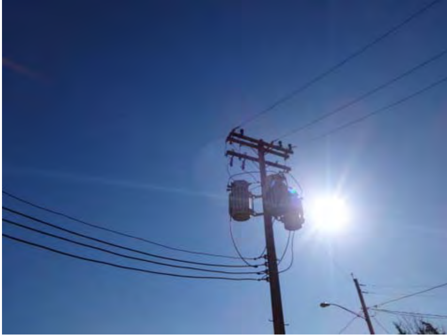
Utility electrical transformer
