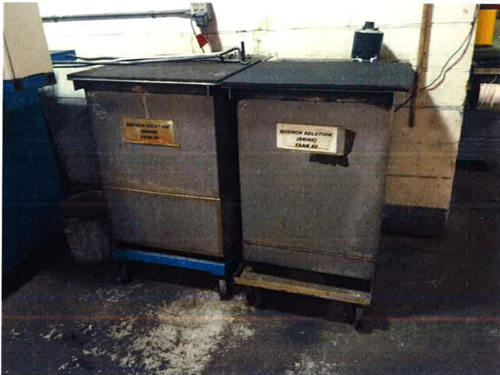
View of aboveground storage tanks in the former black oxide line area (i.e., on the north interior portion of the assessed building).
