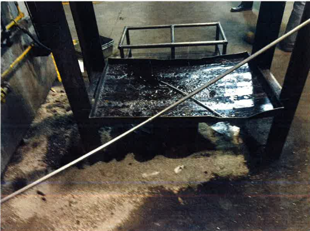
View of spillage of quench oil and absorbent material in the original manufacturing area (i.e., on the western interior portion of the assessed building).
