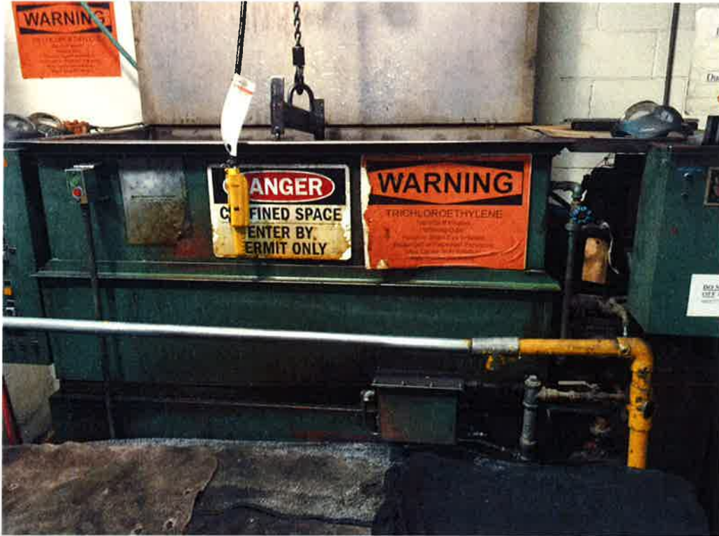
View of the TCE degreaser (i.e., on the southwest interior portion of the assessed building).
