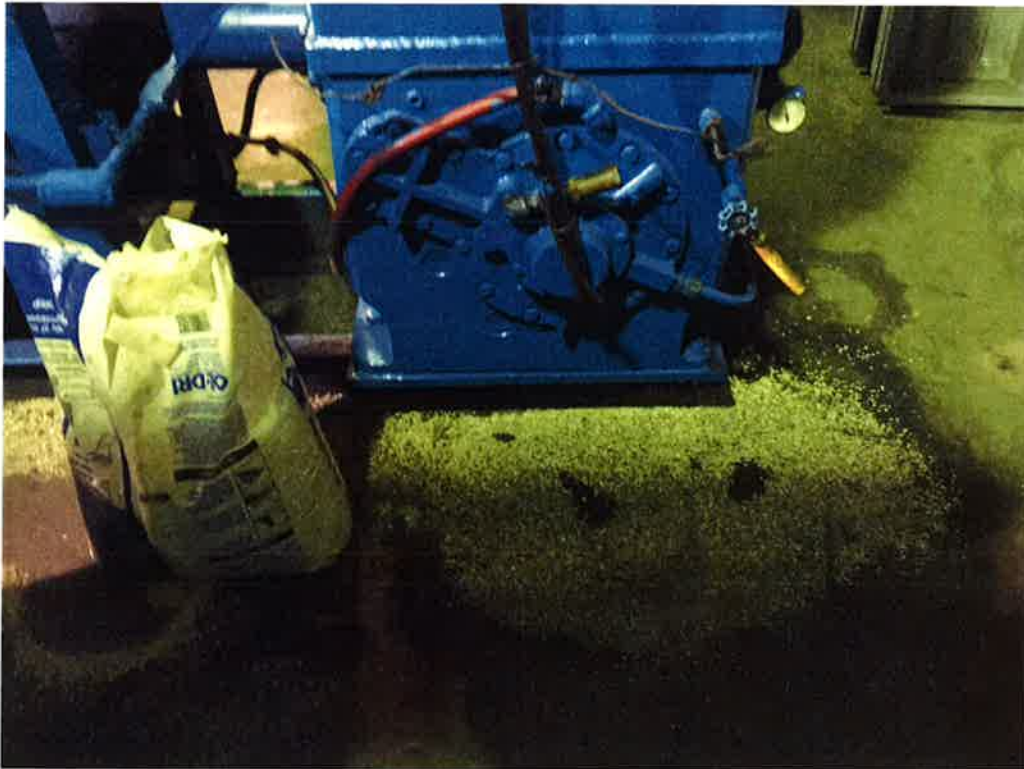
View of spillage of condensed oil and absorbent material located on the concrete floor of the new vacuum room (i.e., on the eastern interior portion of the assessed building).
