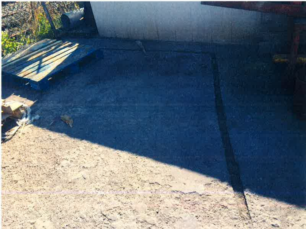
View of a cut in the concrete on the northern exterior portion of the assessed property used for drainage to the adjoining property to the east (i.e., railroad), looking southeast.
