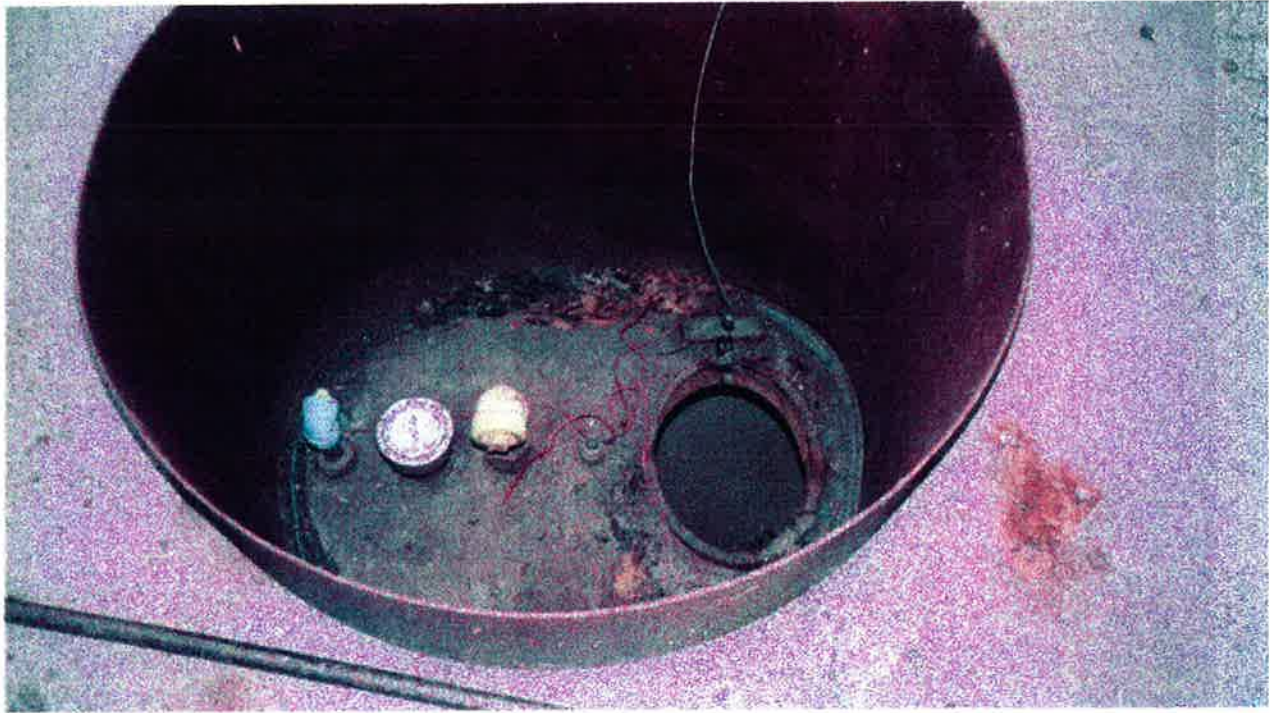
Methanol UST with pressure cover removed
