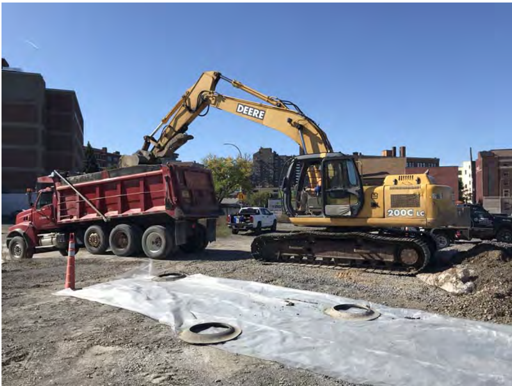
Remove and load out decontamination pad for disposal at High Acres Landfill - looking southwest (10-11-2019)
