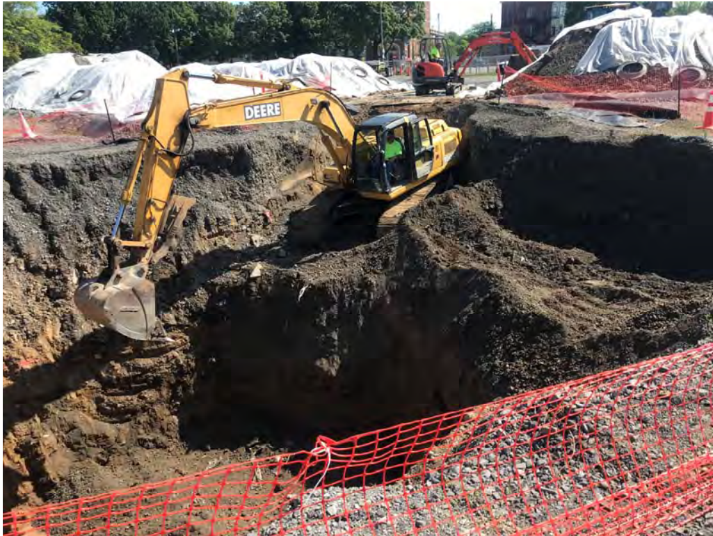
Commence backfilling of excavation with previously excavated and staged re-usable Site soil – looking southeast (9-16-2019)
