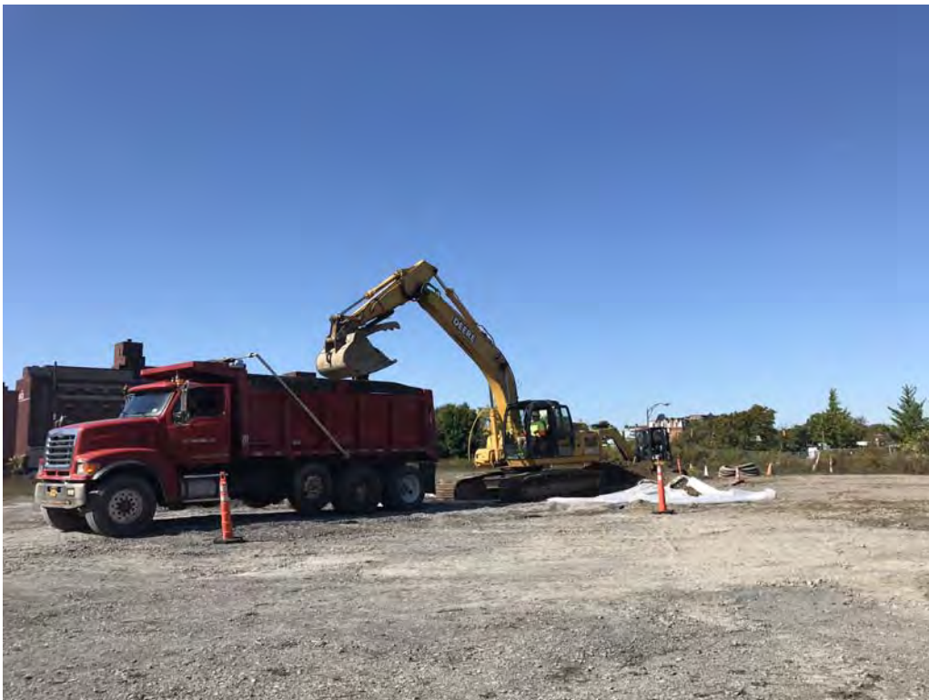
Load out of contaminated soil for disposal at High Acres landfill – looking northwest (10-10-2019)
