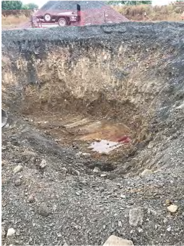
Contaminated soil removal from north end of removal area with field evidence of previously injected potassium permanganate in standing groundwater – looking northwest (9-12-2019)
