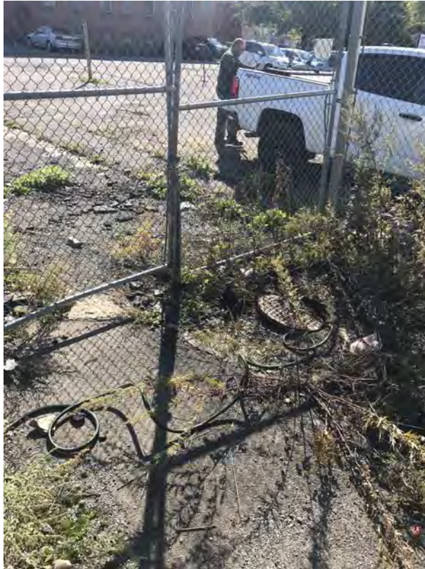
Frac tank discharge to sewer manhole in Bristol Street under Monroe County permit – looking southwest (10-10-2019)
