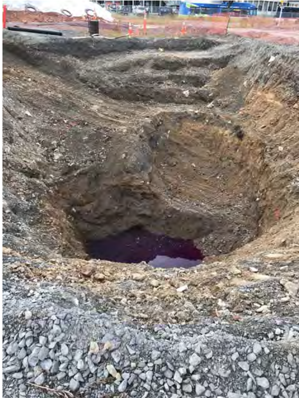
Standing groundwater with potassium permanganate that accumulated in excavation overnight and was pumped to frac tank – looking south (9-13-2019)
