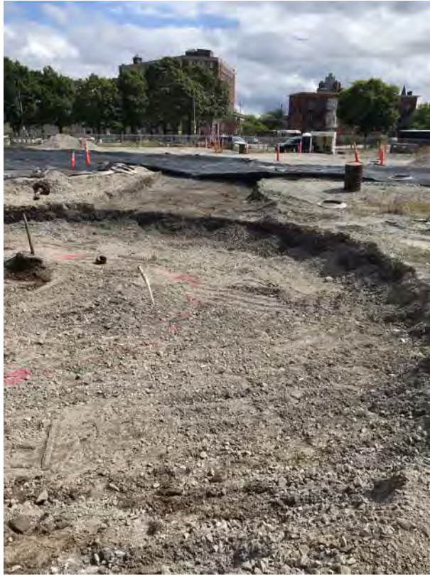
Earthen cover system material removed from excavation area and ramp area – looking southeast (9-9-2019)
