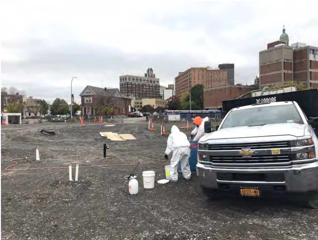
Mixing potassium permanganate for injection at ISCO piping system in backfilled excavation – looking southeast (10-18-2019)
