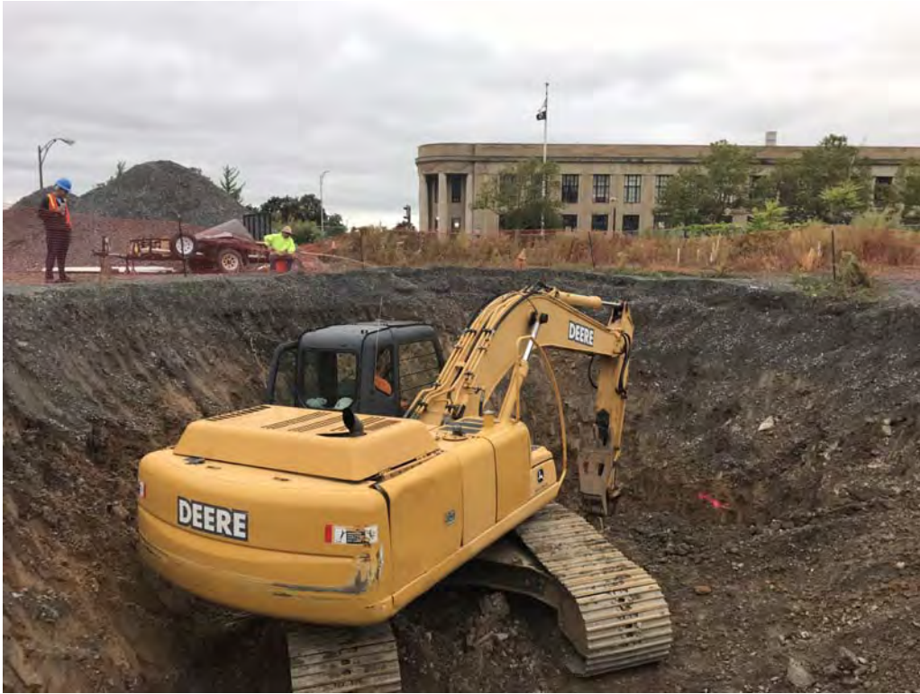
Application of Biosolve Pinkwater vapor suppressant during removal of contaminated soil – looking north (9-12-2019)
