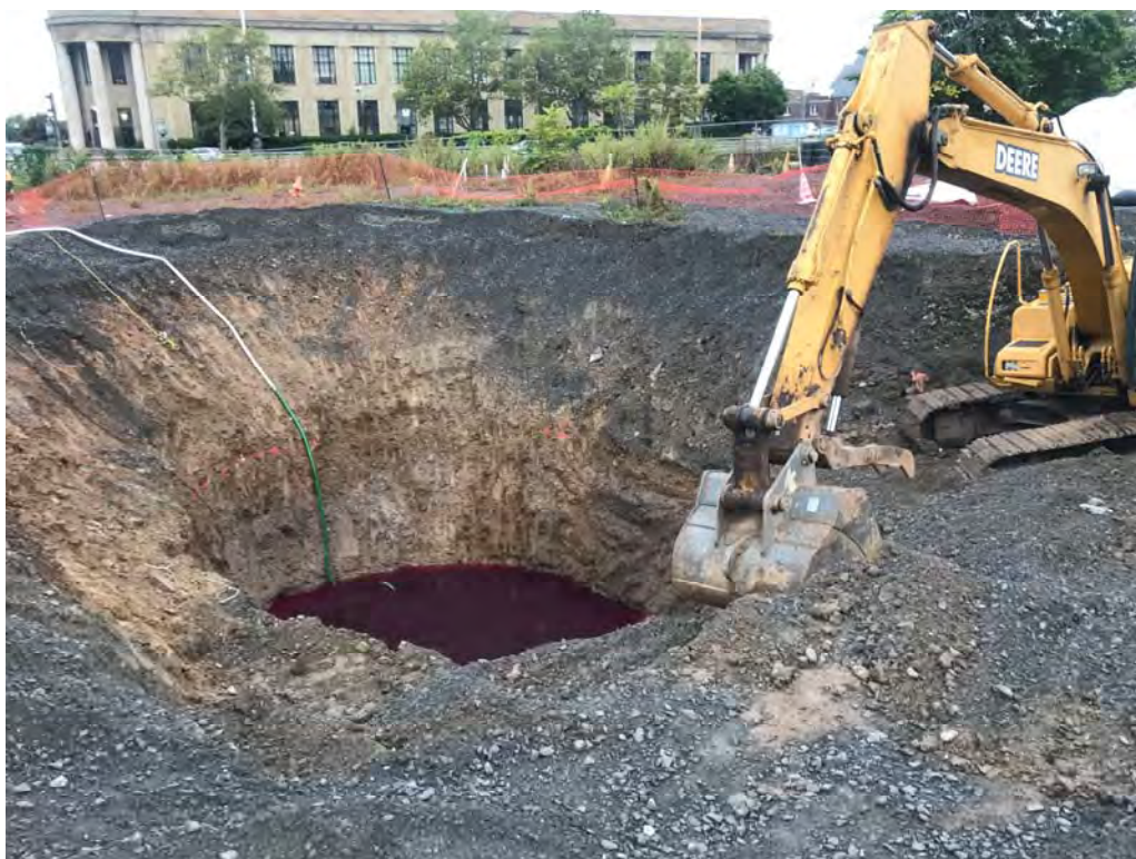
Standing groundwater with potassium permanganate that accumulate in excavation overnight being pumped to frac tank – looking northeast (9-16-2019)
