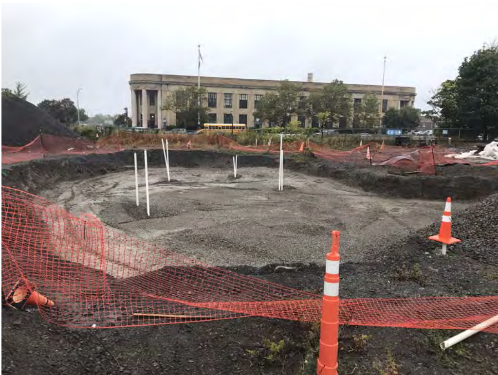
Excavation prior to placement of staged existing cover system material (e.g., crusher run #2) - looking northeast (9-23-2019)
