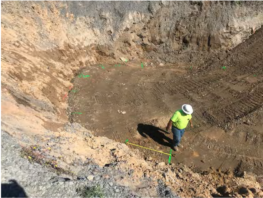
Mark out trench locations for installation of ISCO pipe hardware through backfill – looking northeast (9-17-2019)
