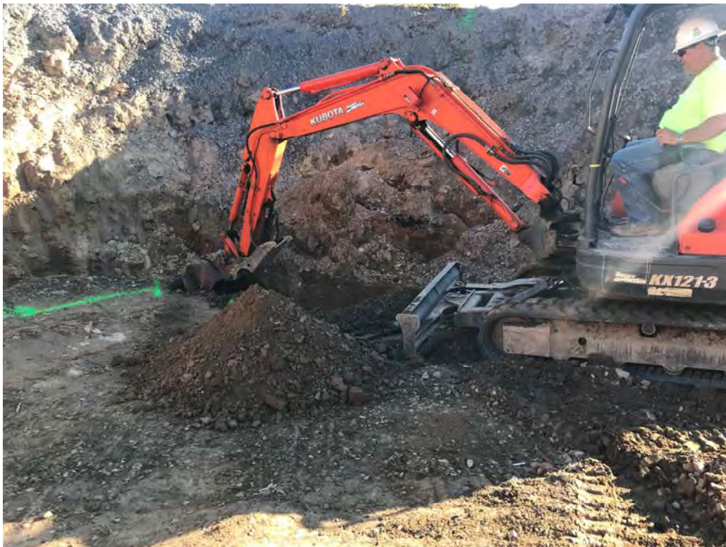
Trenching through partial backfill to install perforated ISCO piping at desired depth (9-18-2019)
