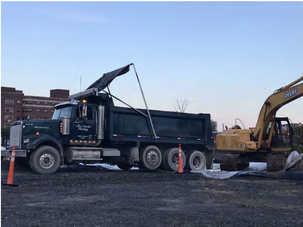
Load out of contaminated soil for disposal at High Acres landfill – looking northwest (10-9-2019)
