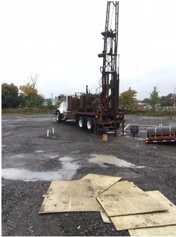
Rotary drill-rig set up to install replacement monitoring well MW-17A – looking northeast (10-17-2019)
