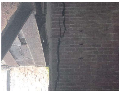
Figure 13 - Cracking of Masonry
