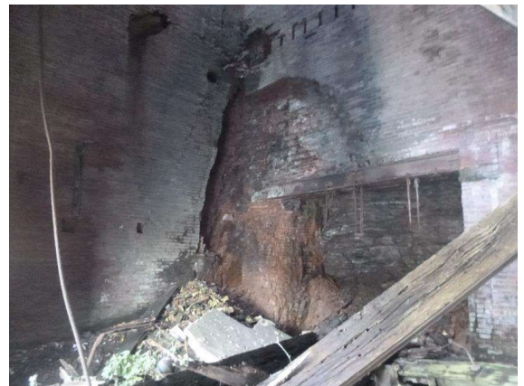
Figure 12 – Significant Cracking and Unsecured Brick
