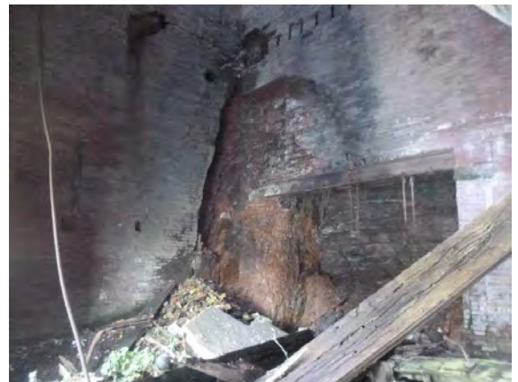
Figure 12 – Significant Cracking and Unsecured Brick
