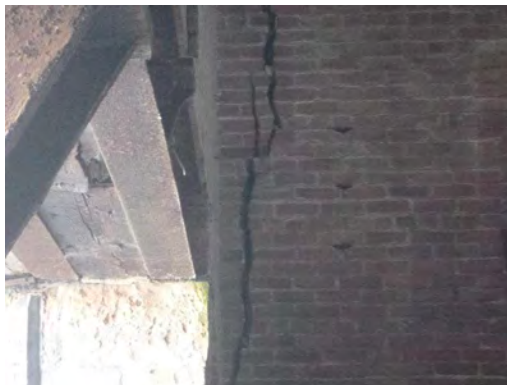
Figure 13 - Cracking of Masonry
