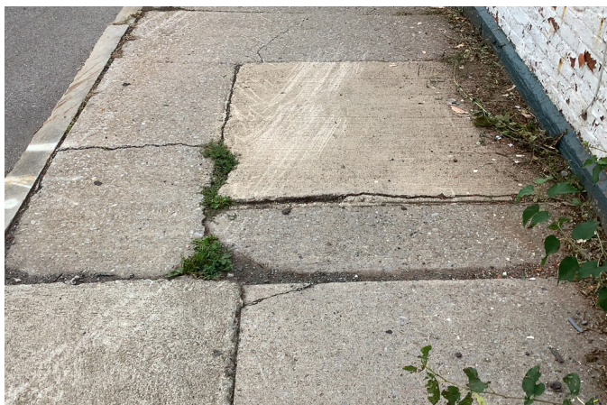
Uneven sidewalk on North Union Street
