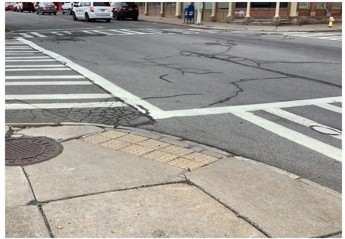
Diagonal curb ramp on North Clinton Avenue
