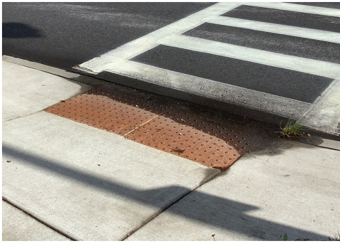
Water accumulation at the base of a curb ramp on Lake Avenue
