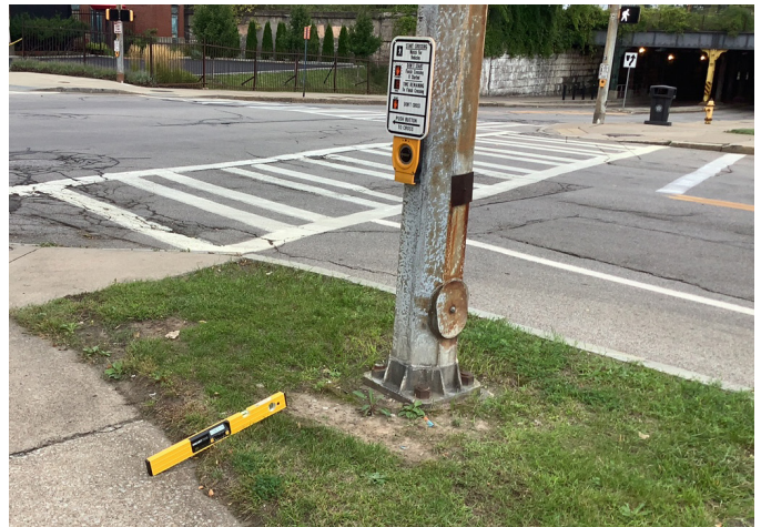
Pedestrian signal button located on an inaccessible surface on North Clinton Avenue
