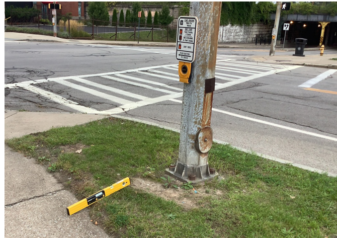
Pedestrian signal button located on an inaccessible surface on North Clinton Avenue
