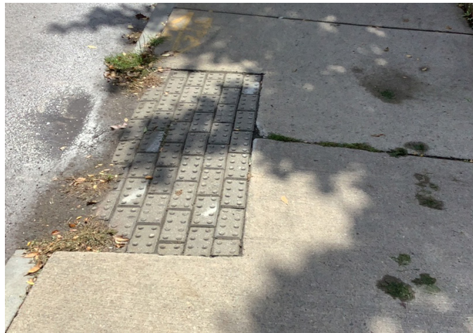
Detectable warning strip on Lake Avenue that does not provide sufficient color contrast
