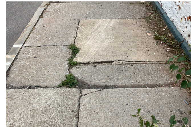
Uneven sidewalk on North Union Street
