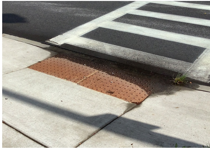
Water accumulation at the base of a curb ramp on Lake Avenue
