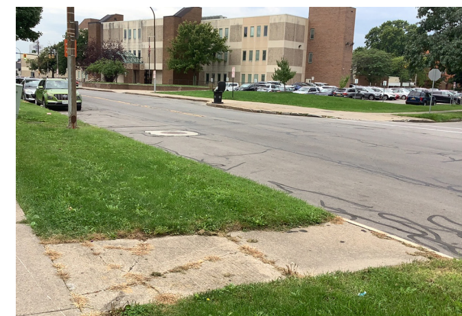
Deteriorating bus boarding area on North Clinton Avenue
