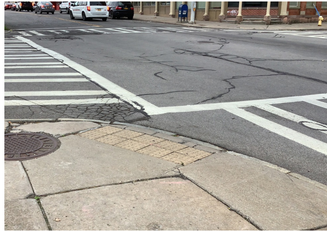
Diagonal curb ramp on North Clinton Avenue
