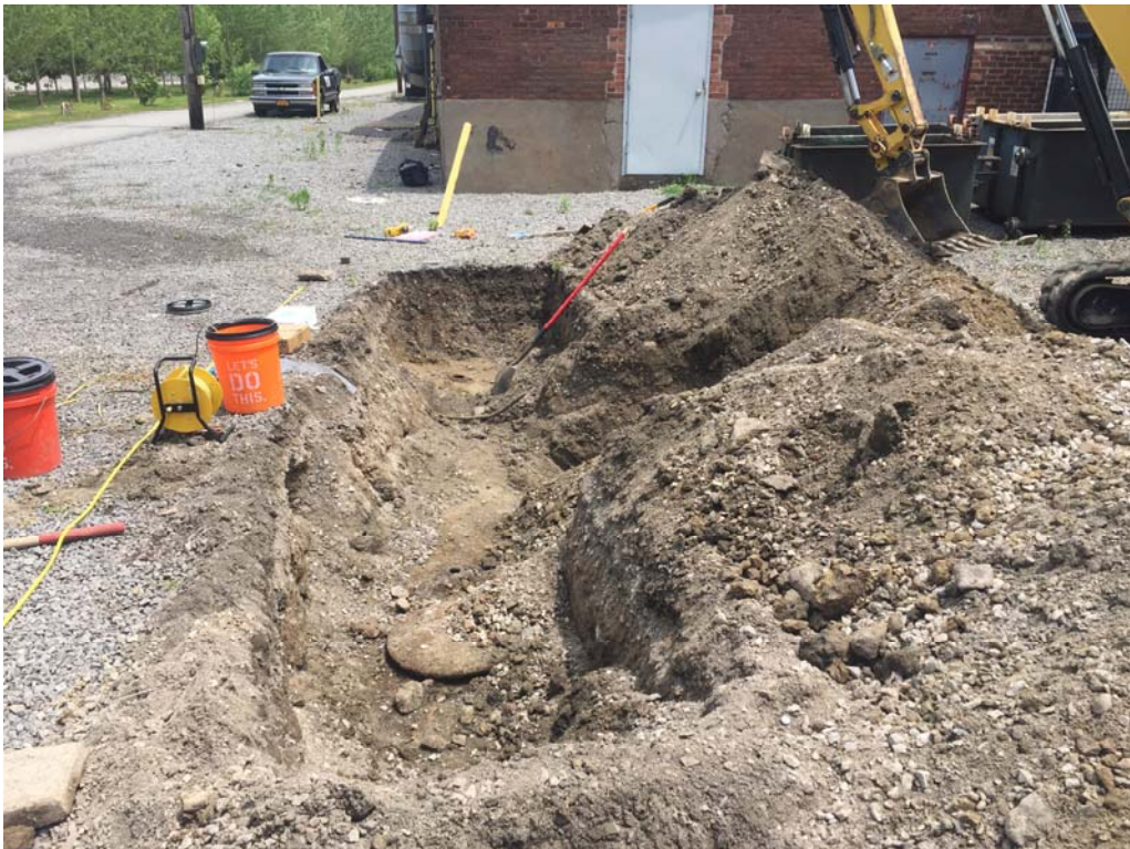
View of approximate 10,000-gallon UST located in north portion of courtyard area north of Main Building, looking east
