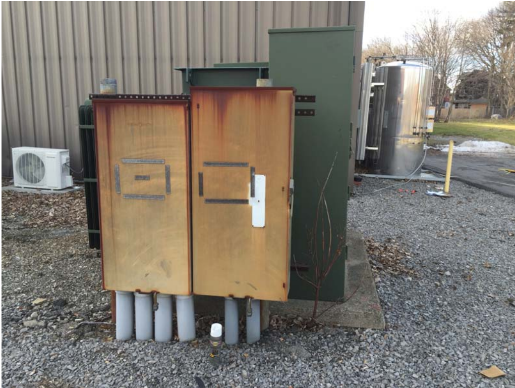
Transformer located on north portion of main building courtyard
