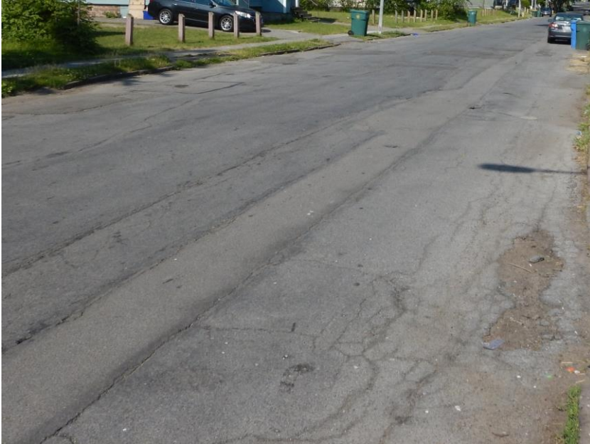
Cracking and Deteriorated Pavement Conditions
