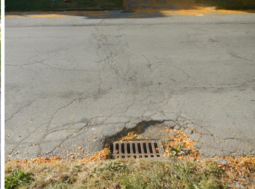
Sunken Cast-Iron Rectangular Grate (Non-Bicycle Friendly) Drainage Inlets
