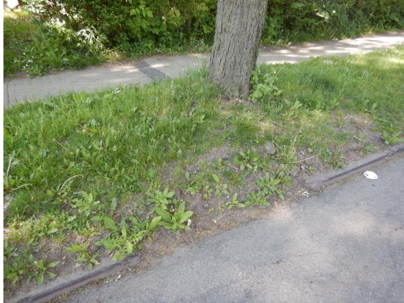
Broken and Missing Sections of Stone Curb Damaged By Mature Trees
