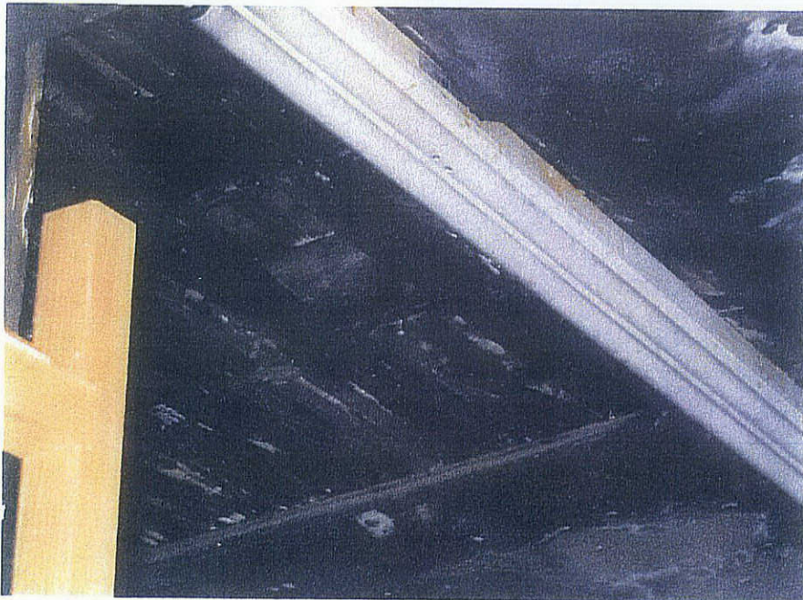
Photo 22 Looking at the ceiling/roof structure of Building - 9. Notice the structure is full of moisture.
