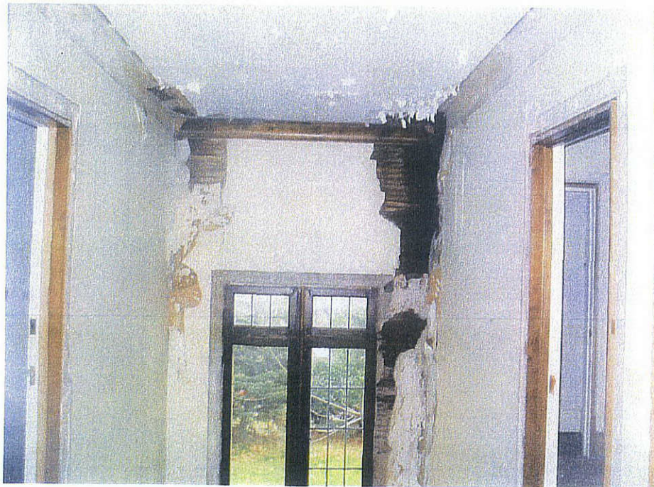
Photo 20 Looking at one of the areas (east stair wall of Building - 8) where dryrot/wetrot issues could exist.
