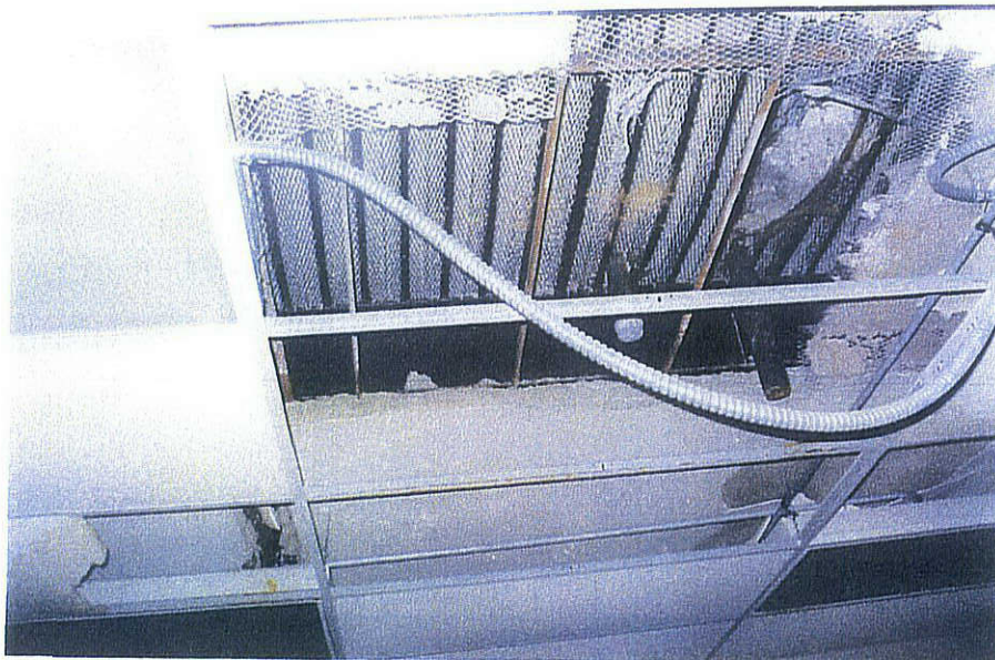
Photo 18 Looking at a section of the floor of Building - 7. The concrete slabs were supported on metal lath.
