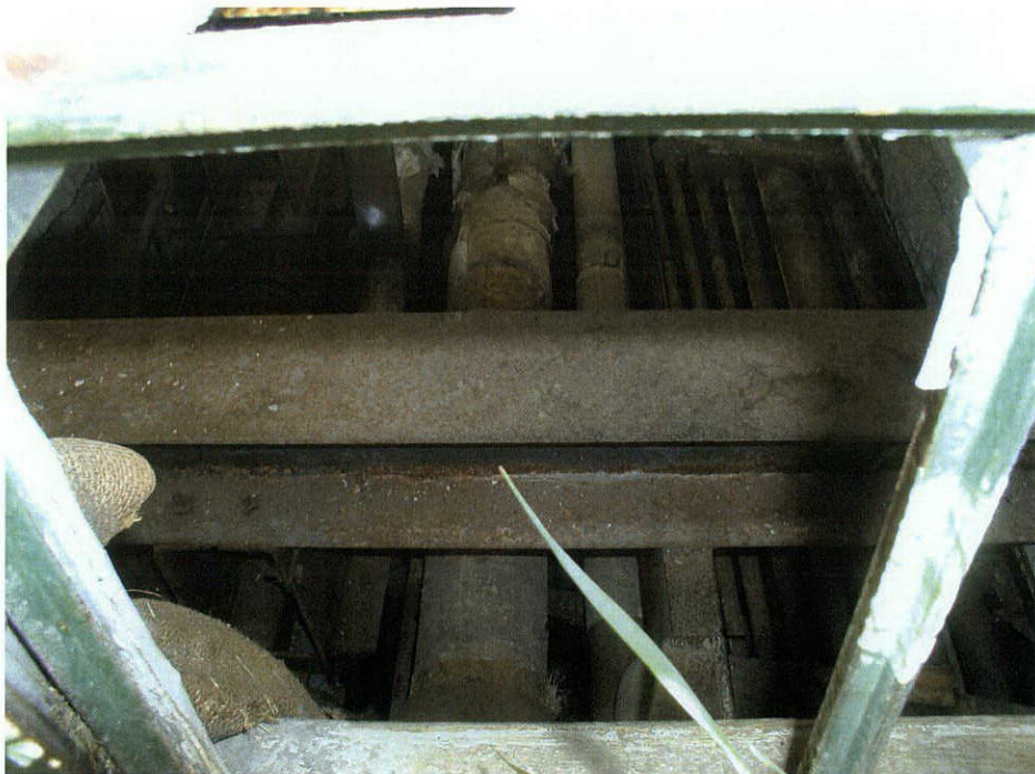
Photograph 42: View of underground pipelines supplying and powering the Iola campus, facing west.
