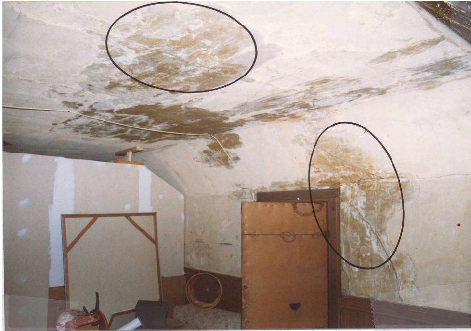
42. Plaster and paint damage at attic level.
