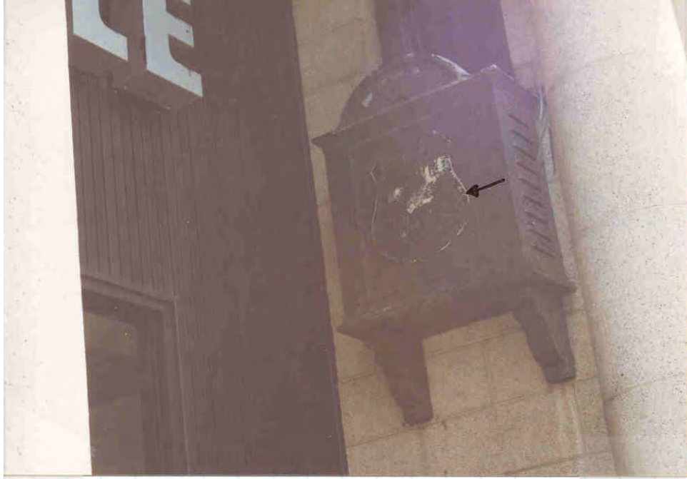
21. Rusted bank alarm. 1
