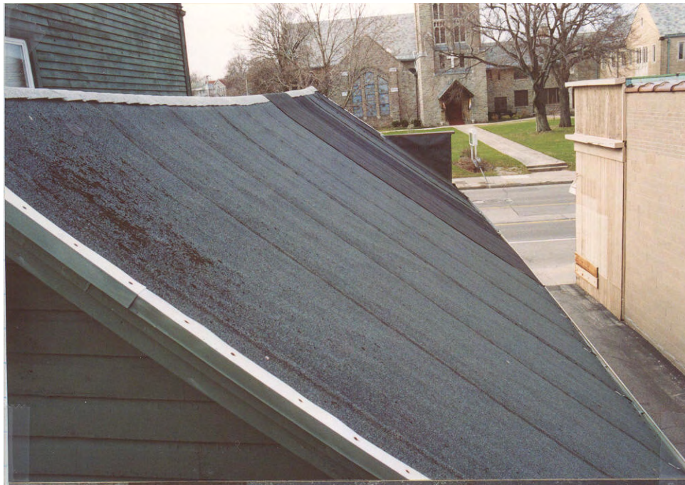
4. Deteriorated roofing on building 1. Note sag in roof structure.
