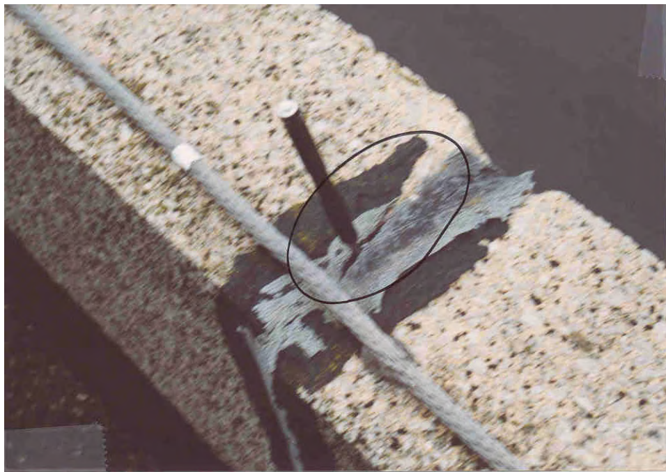
18. Open joints at south facade coping.
