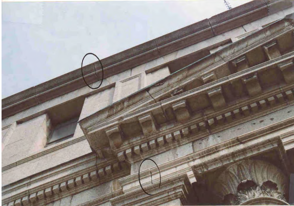
13. Open joints at south facade.
