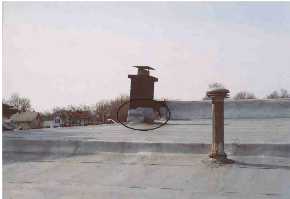
8. Missing counter flashing on east chimney.
