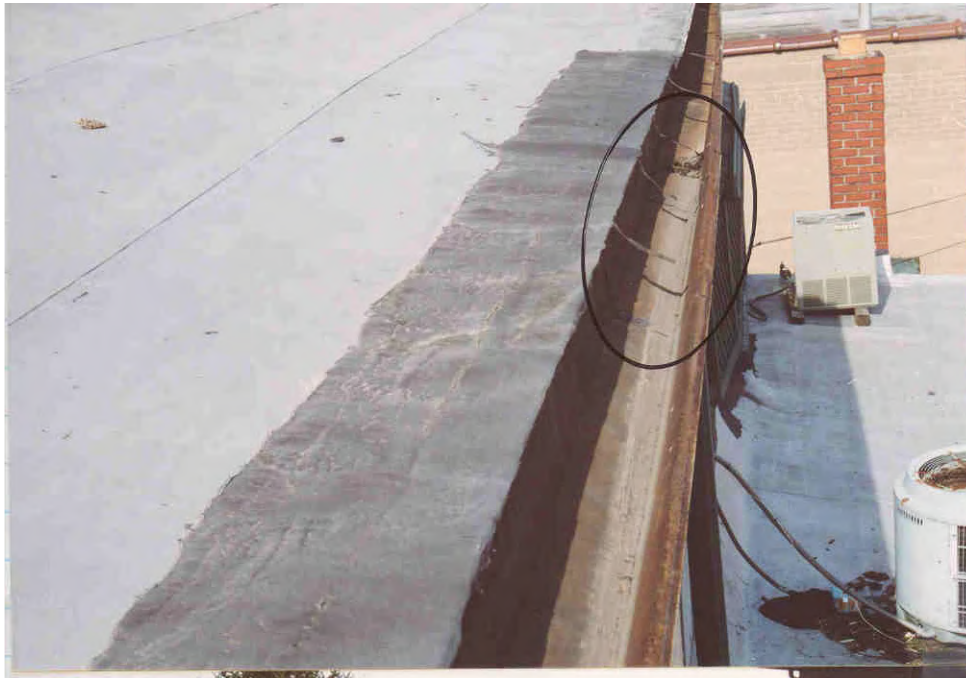
14. Rusted, failing gutter at north
