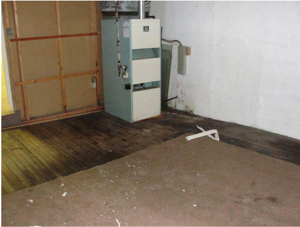
25. Building 1A sagging floor, west side at junction with Building 1.
