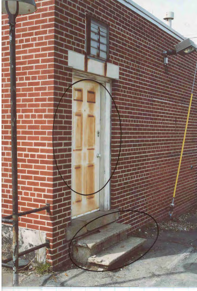
23. Rusted door and vent at north, note stair deterioration.
