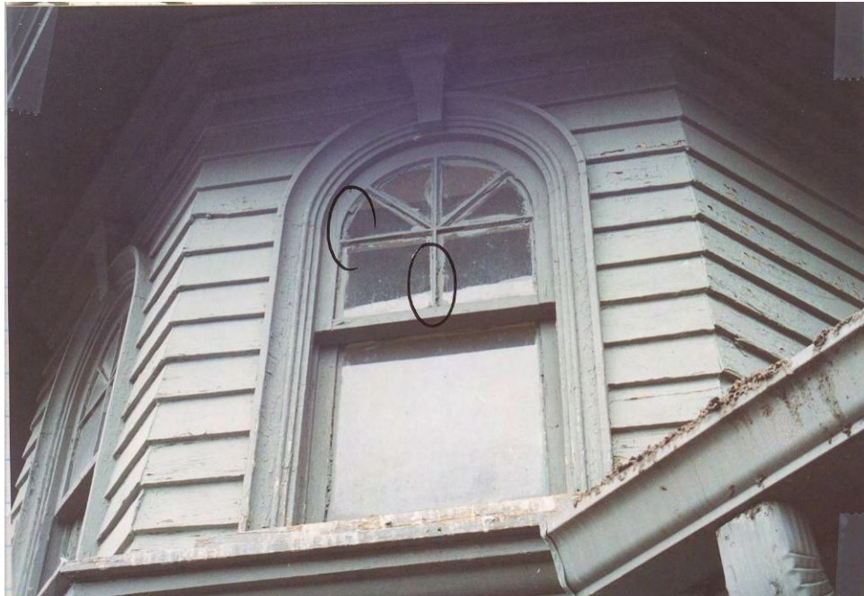
41. Paint and glazing failure at south window.
