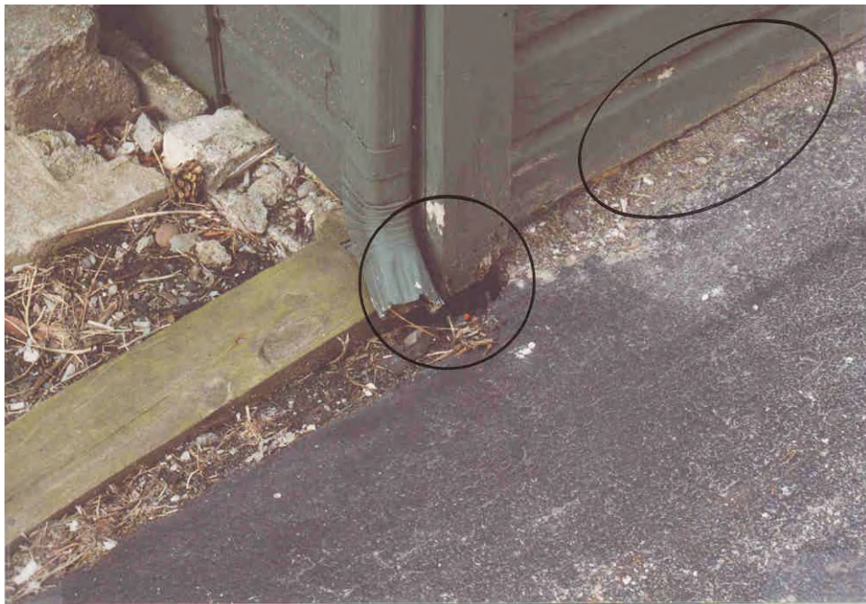
12. Downspout dumping water at wood sill note all wood in contact with contact to the ground.
