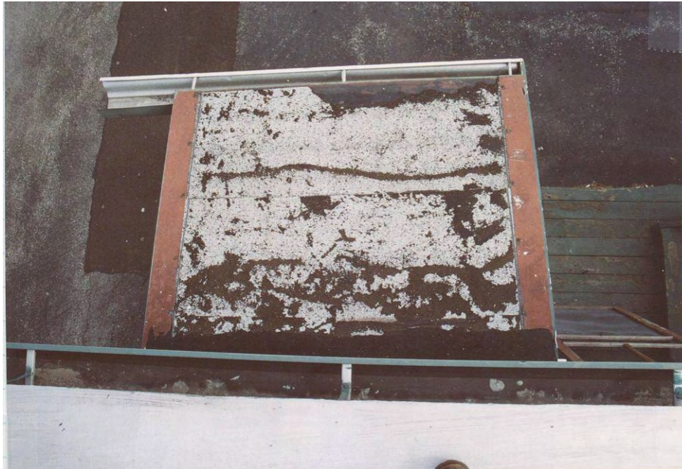
5. Deteriorated roofing at NW of building 1 Deteriorated roofing at NW of building 1a.
