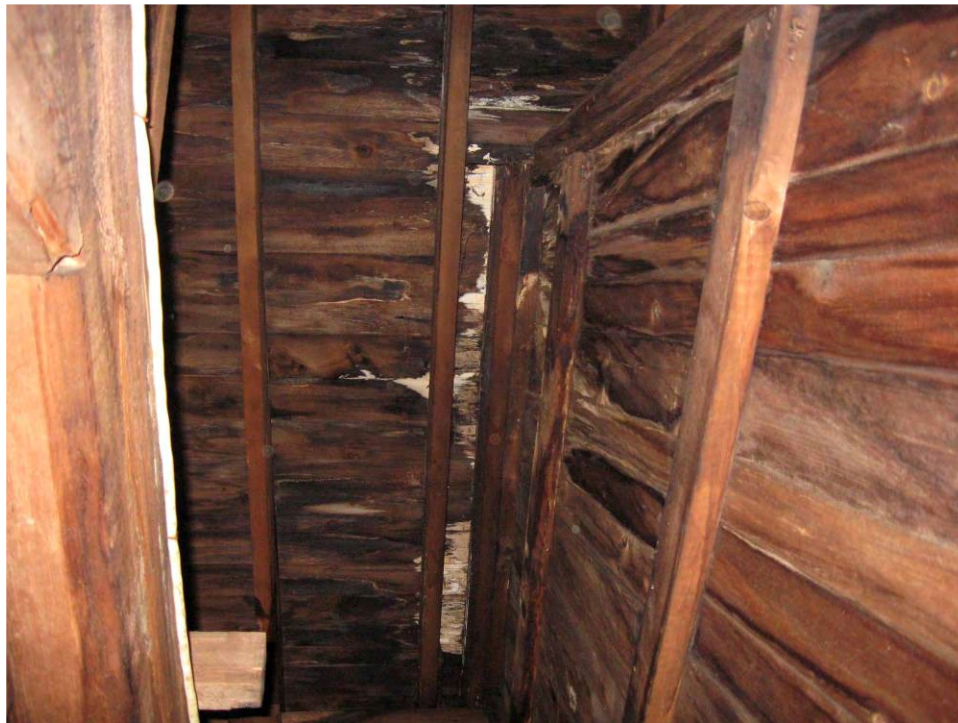
55. Roof sheathing deterioration in west attic. Refer to 2004 photo 28
