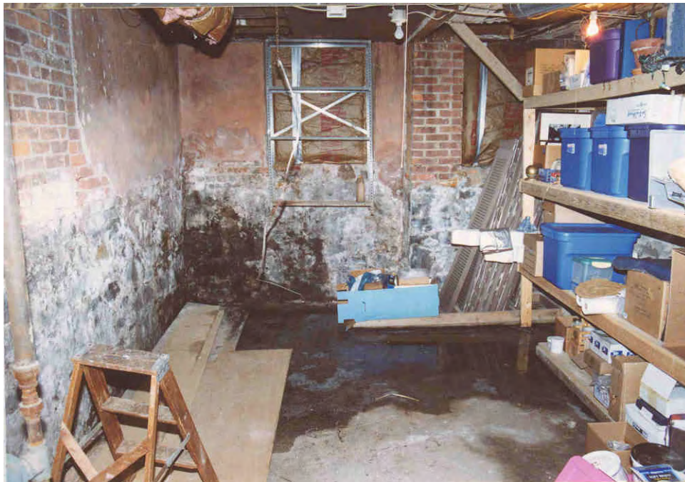
17. Wet basement at northwest, possible storm drain leak/clog.
