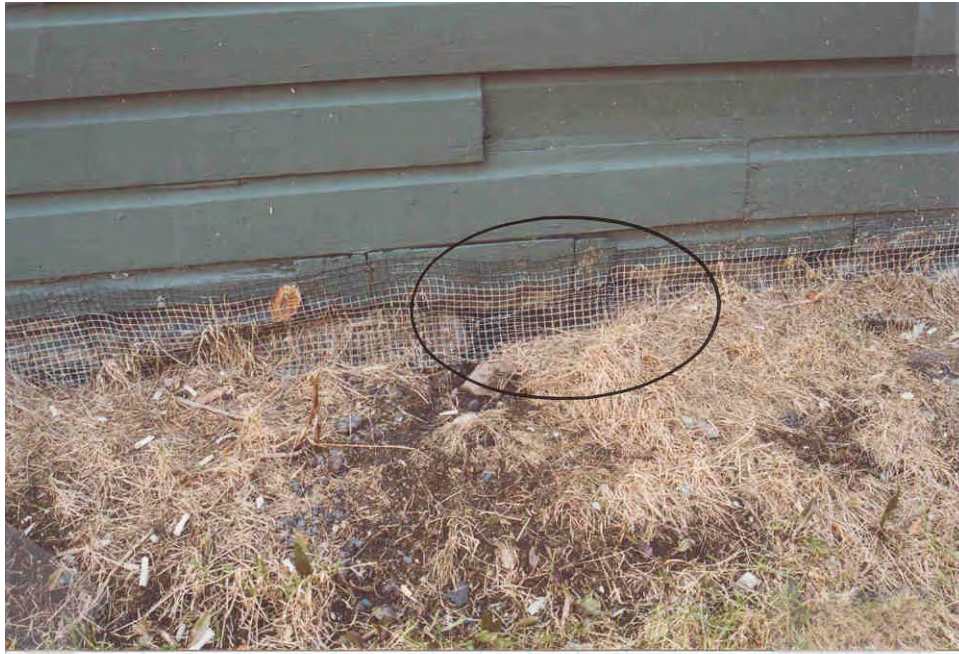
15. Foundation stones missing at west wall, note rotted wood in contact with ground.
