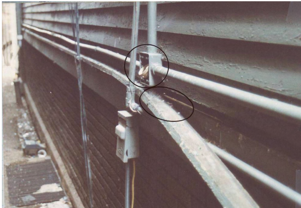
29. Loose water table at east, note open electric box.
