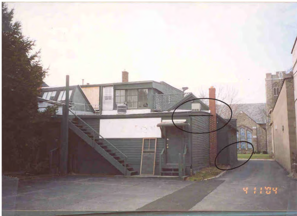
14. Suspected foundation failure, note arch and bow of west walls.
