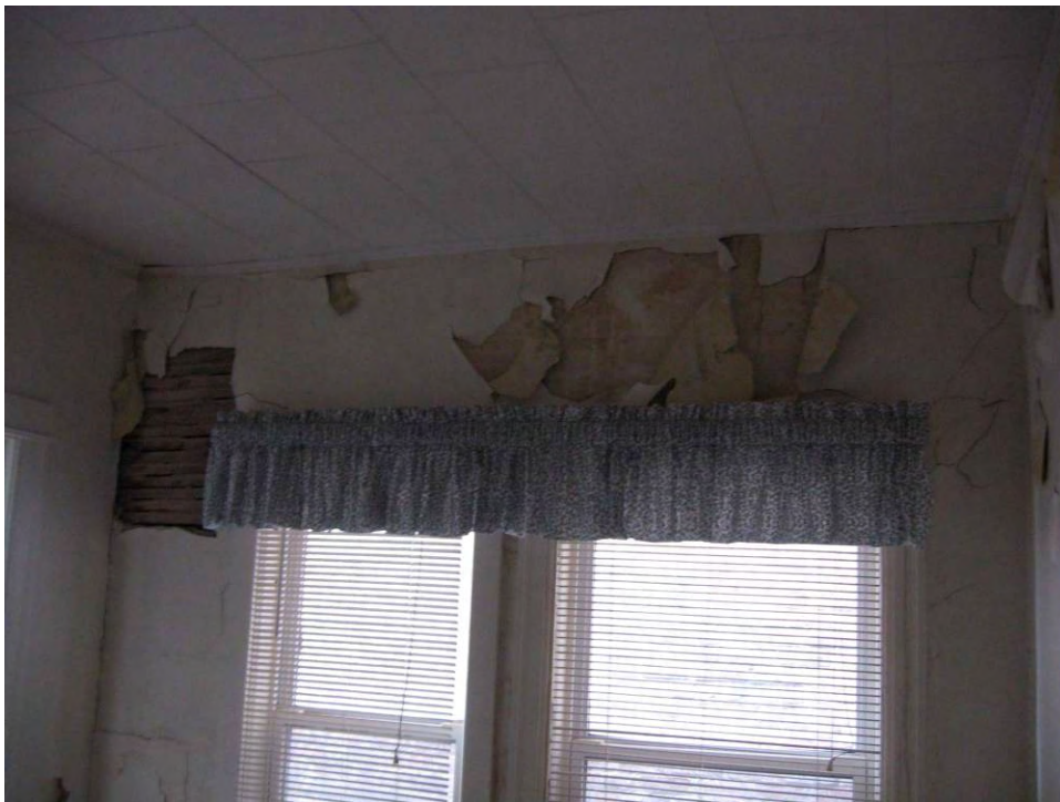
57. Interior finish damage, third floor, west side.
