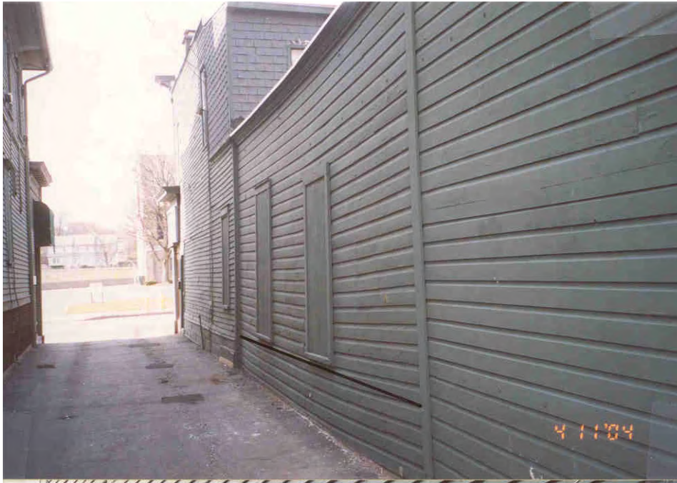
22. Settlement of east wall suggesting sill and foundation deterioration.
