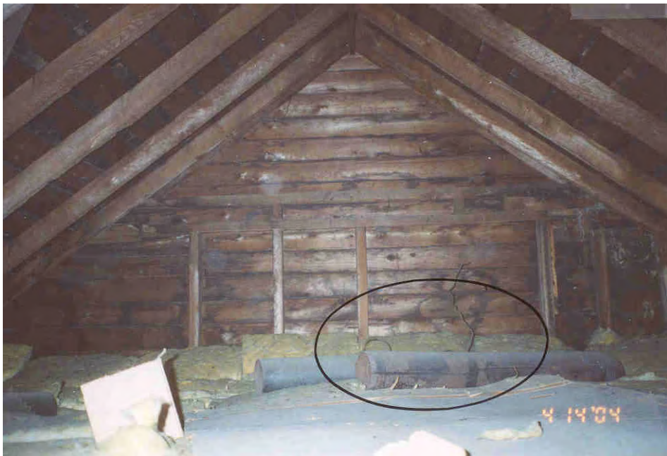
22. Abandoned mechanicals and debris in building 1 attic.
