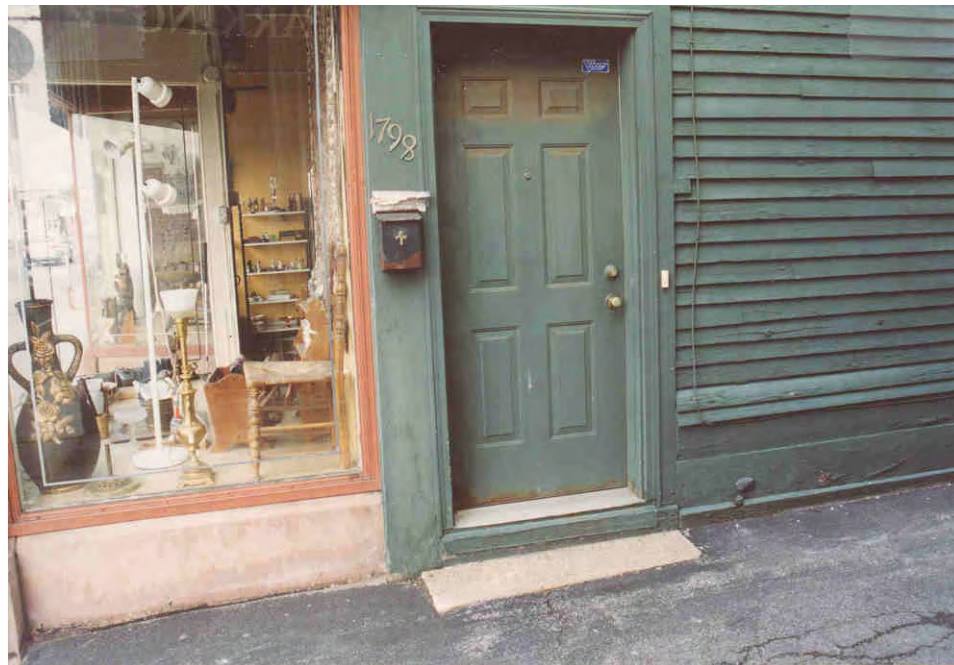
28. Failing paint on siding and rusted door.
