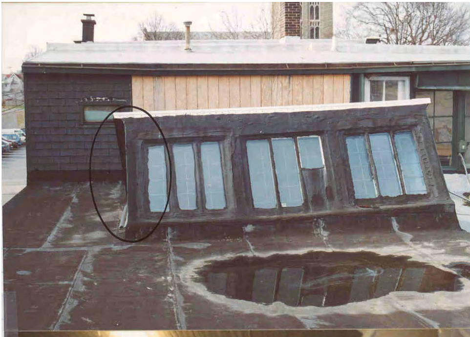
20. Roof sag at skylight east corner.
