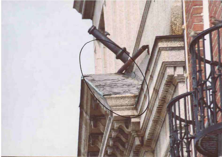
5. Worn out pediment roofing.
