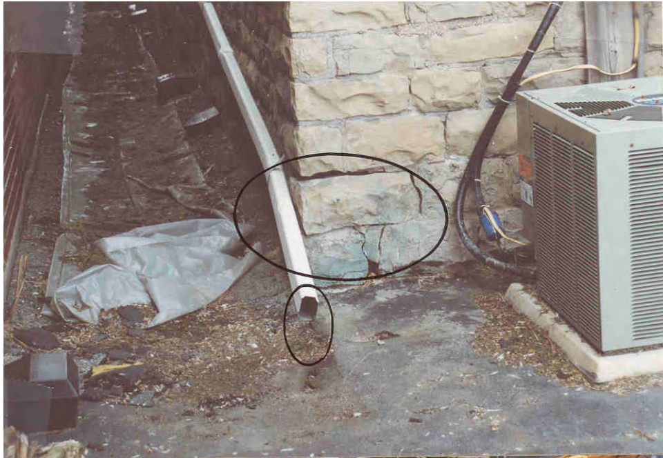
16. Storm water dumping in wet alley note foundation stones.
