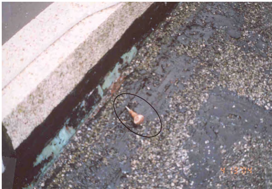
8. Open seam at roof 4.
