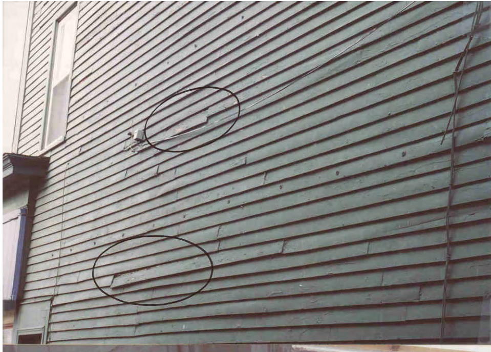
23. Loose and damaged east wall clapboards.
