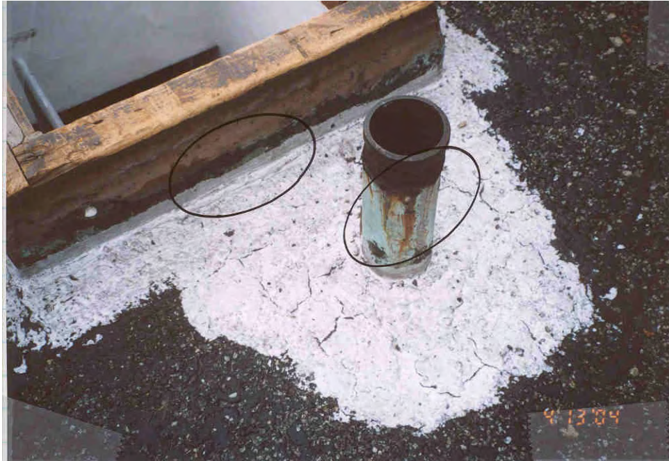
9. Poor flashing at roof 4 penetrations.
