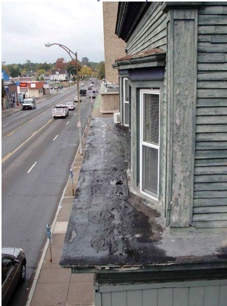
42. South roof deterioration. Refer to 2004 photo 11.
