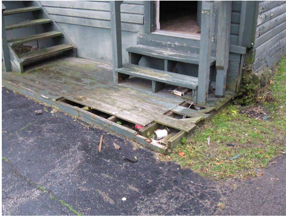
23. North porch construction failure. Unsafe condition.
