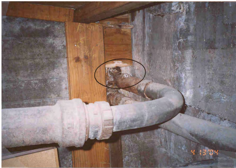
25. Rusted abandoned piping.
