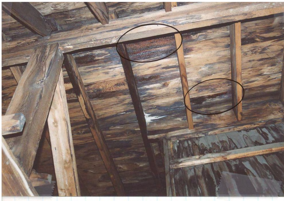
27. Damage at underside of roof deck.
