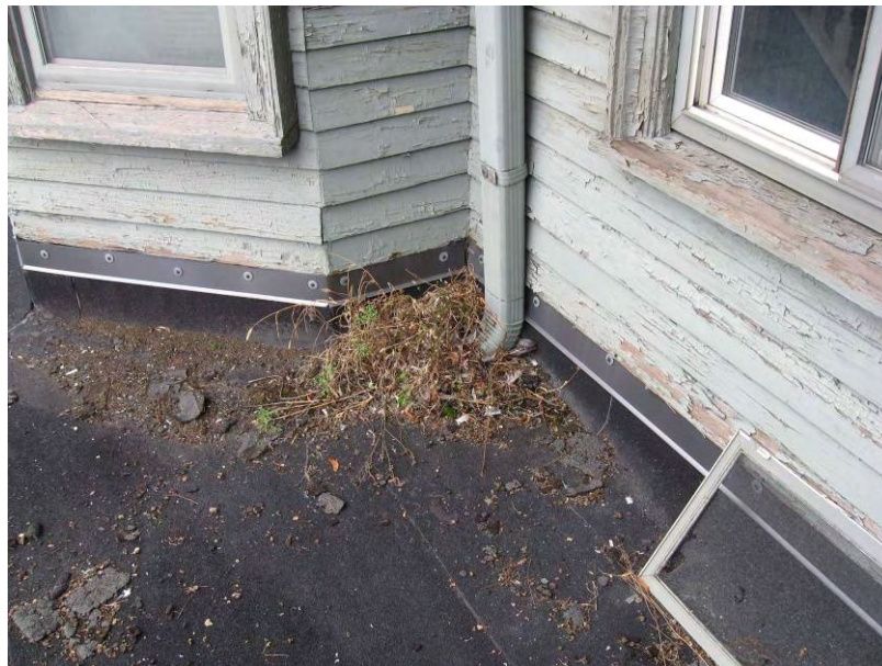
59. South, first floor roof – downspout blocked.
