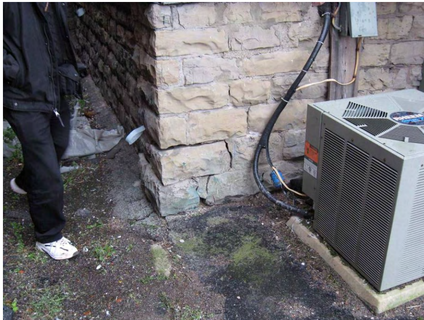
63. North-east deteriorated masonry foundation wall at grade. Note open masonry joints. Possible settlement. Refer to 2004 photos 4, 16.
