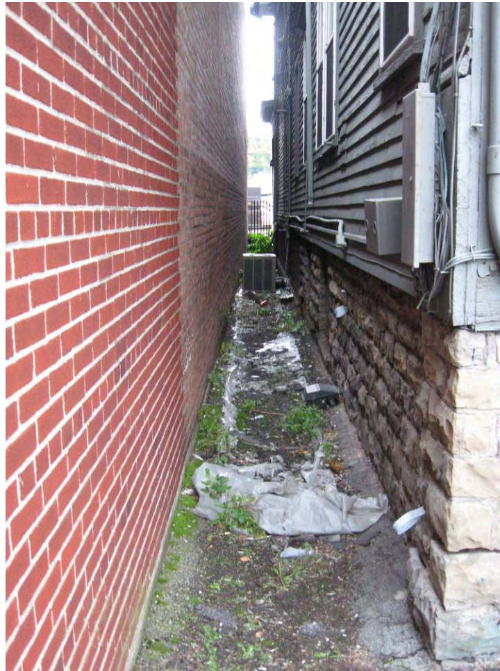
58. Alley between buildings 3 and 4 – holding water – missing downspout. Refer to 2004 photo 4.
