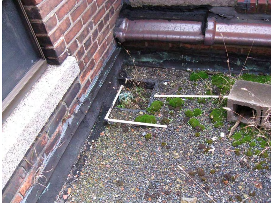
28. Roof 4C – blocked roof drain and sump. Refer to 2004 photos 11, 12.
