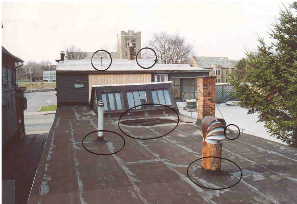
10. Poor flashing at penetrations, note ponded water.
