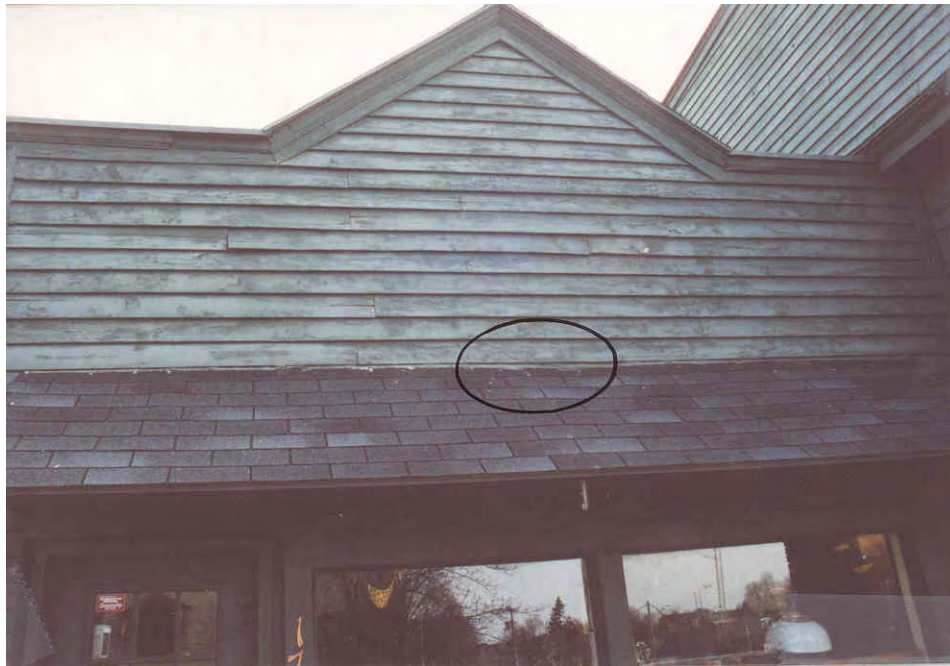
9. Poor flashing at south roof.
