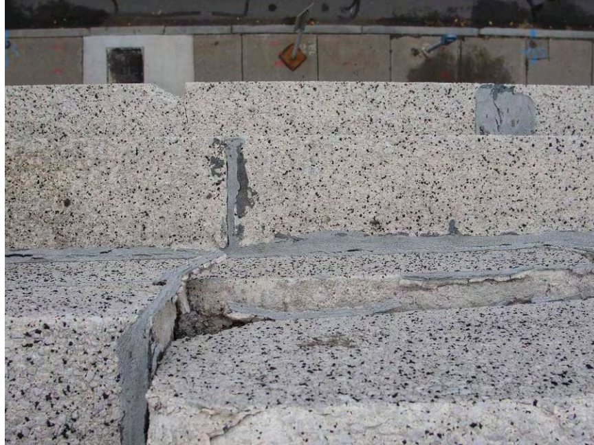
30. South cast stone parapet – open joints and stone shifting. Refer to 2004 photo 18.
