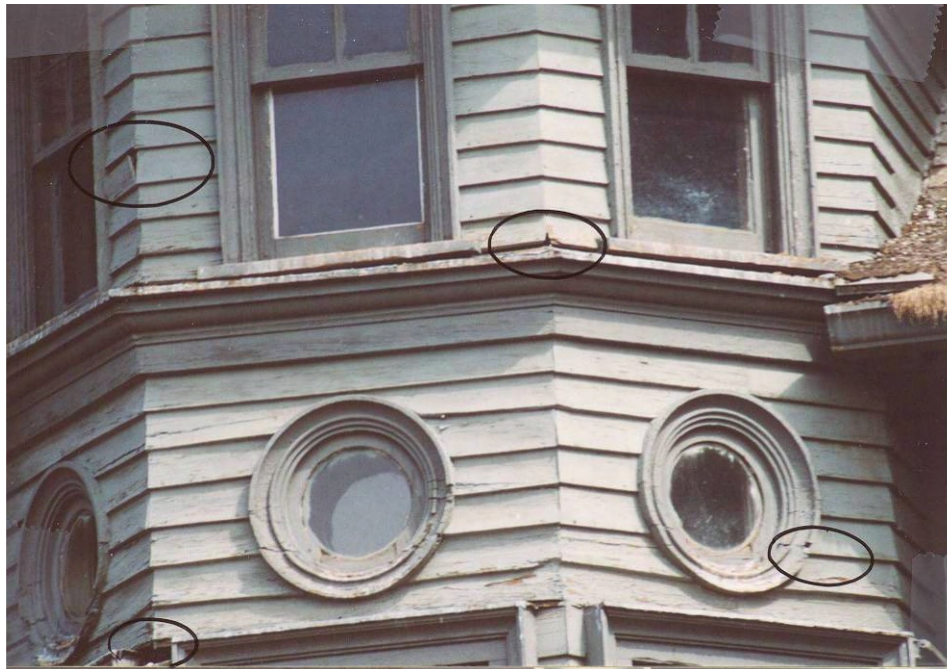
25. Typical window, cornice side wall damage.
