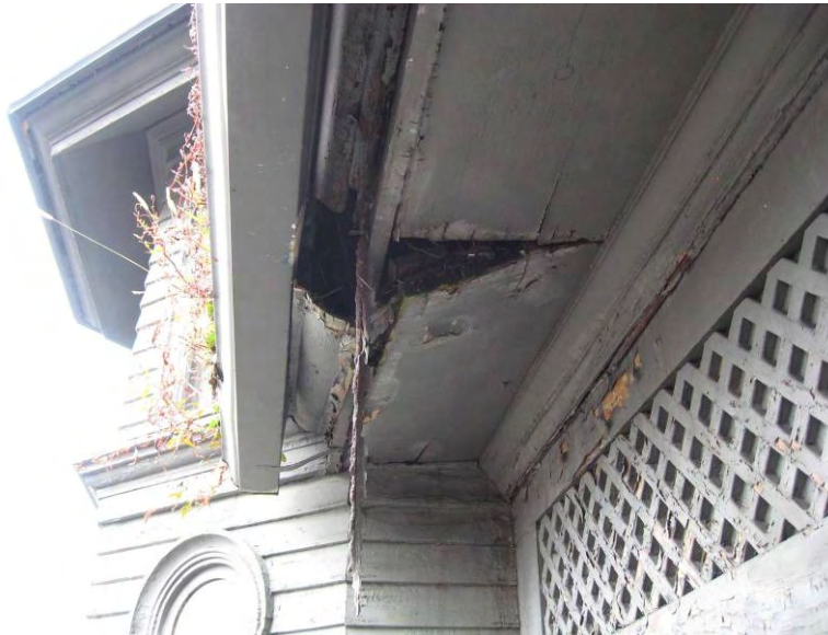
61. South soffit deterioration.
