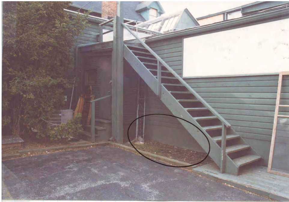
3. Grade sloped to building 1a at north.
