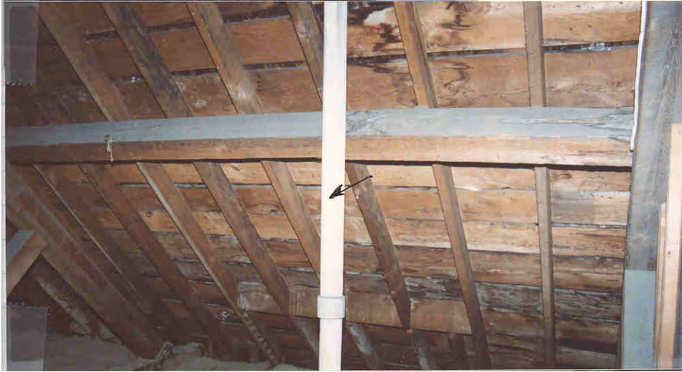
44. Possible asbestos containing pipe.
