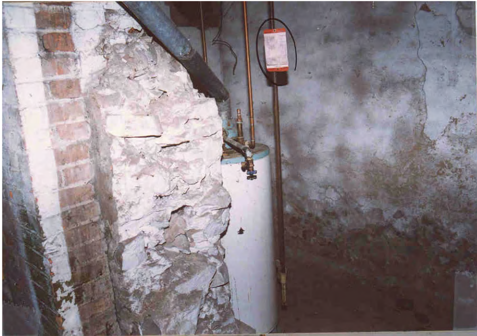
47. Unsafe water heater per RG&E tag.
