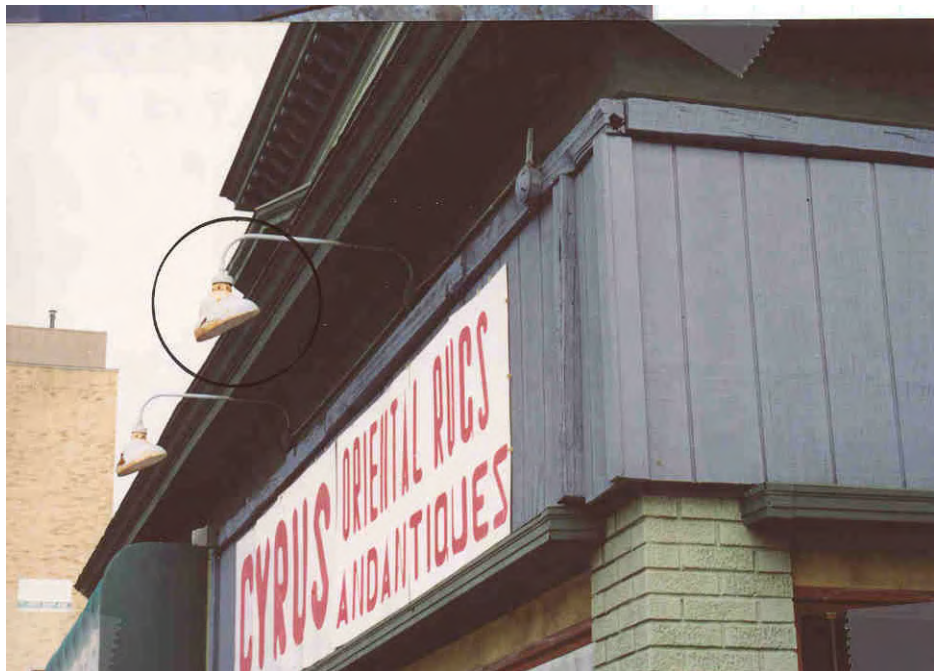
36. Rusted lights at south.
