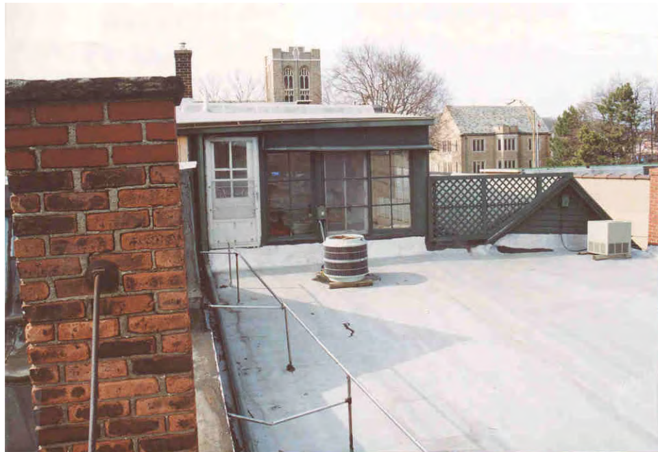
16. Deteriorated chimney on building 2a .
