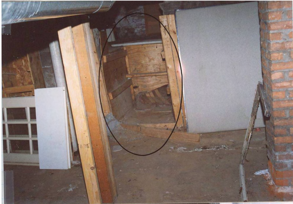
32. Missing stair in basement.
