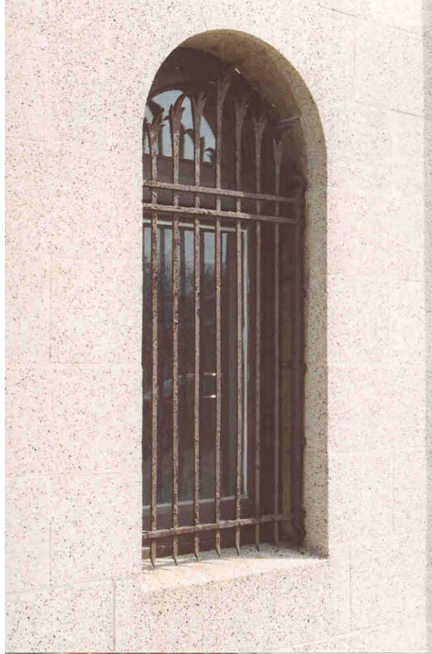
22. Rusted window and bars at south. 1
