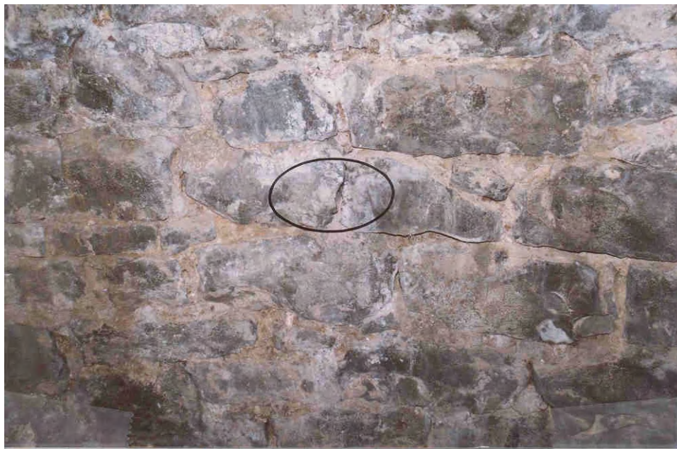
21. Open joints at interior basement wall.
