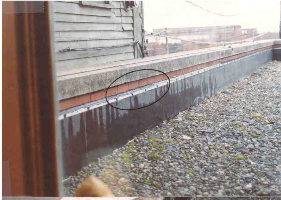
7. Missing counter flashing at roof 4a.
