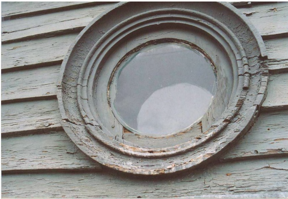
39. Rot at south window.
