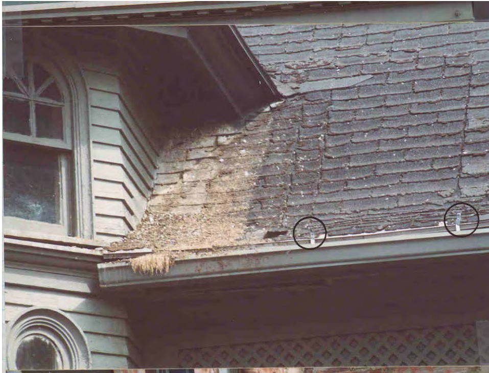
14. Exposed fasteners at gutter hangers.
