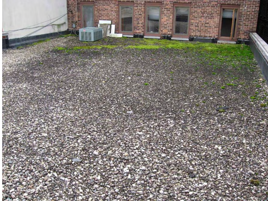
36. Roof 4B showing moss cover and general deterioration.
