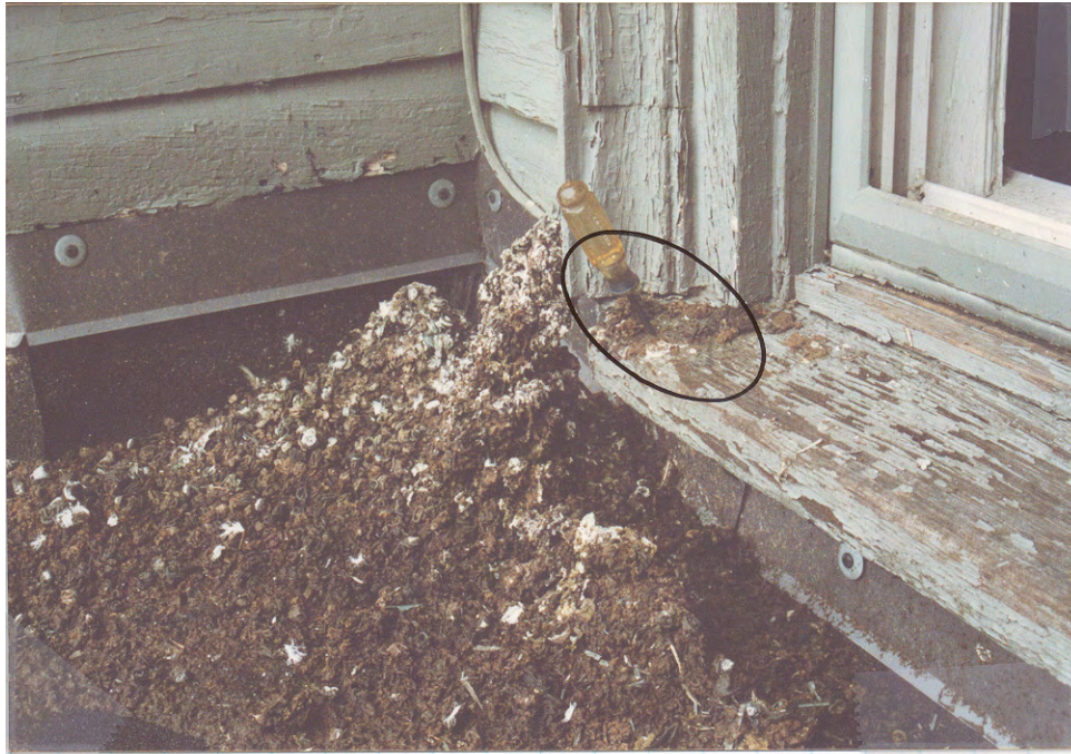
24. Rot at south window sill.
