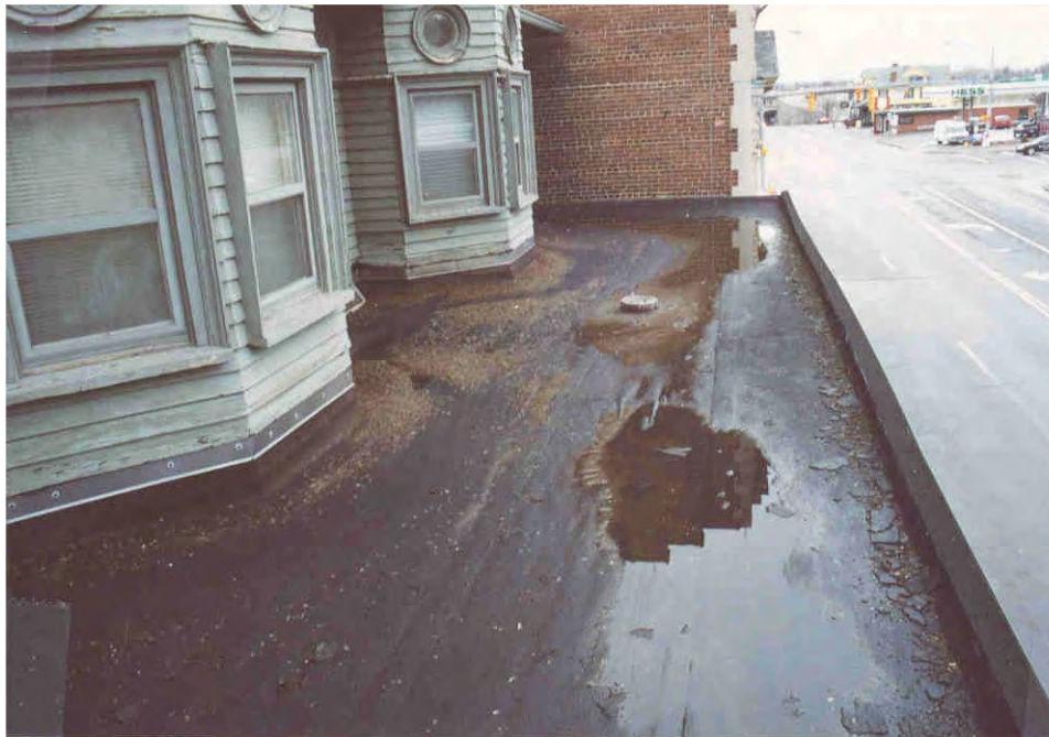
5. South roof, note accumulated pigeon droppings and roof shingles.
