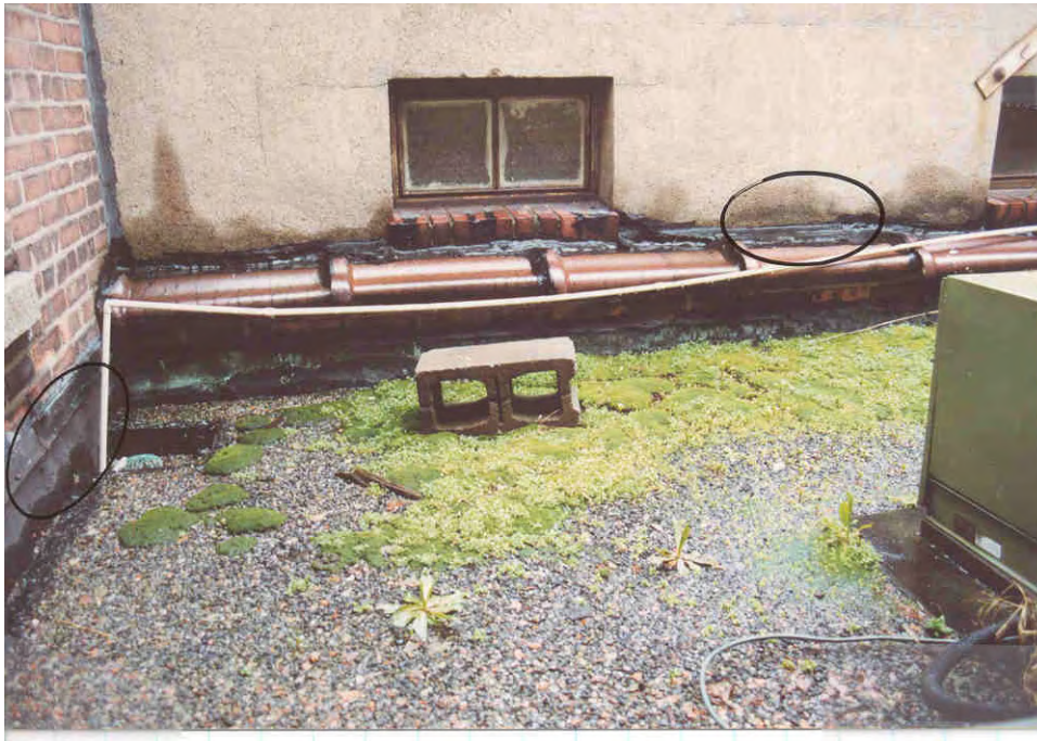
12. Tar coated flashing and connection neighbor building.
