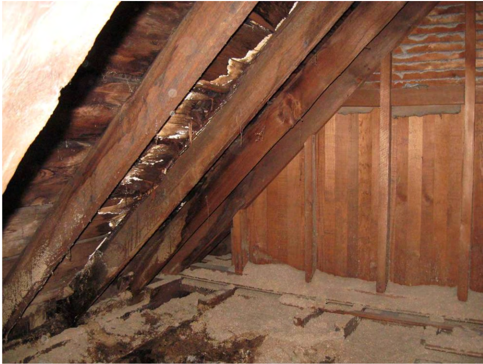
56. Roof sheathing deterioration and insulation damage in west attic.
