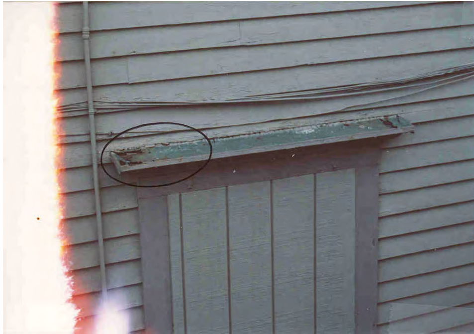
12. Deteriorated window cap flashing.
