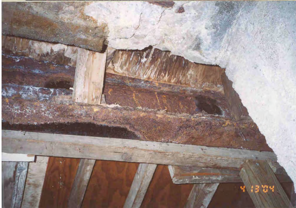
17. Deteriorated beam at south of basement.
