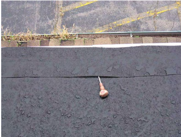
41. North roof membrane separation.
