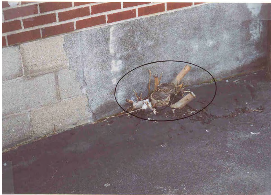
4. Tree stump at west wall.
