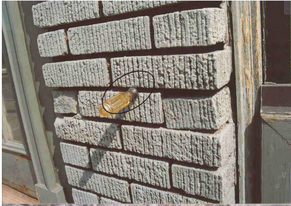
20. Repointing required at south.
