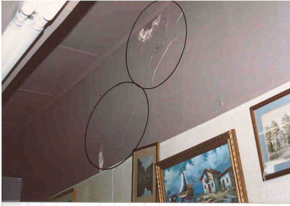
27. Interior paint and plaster damage.
