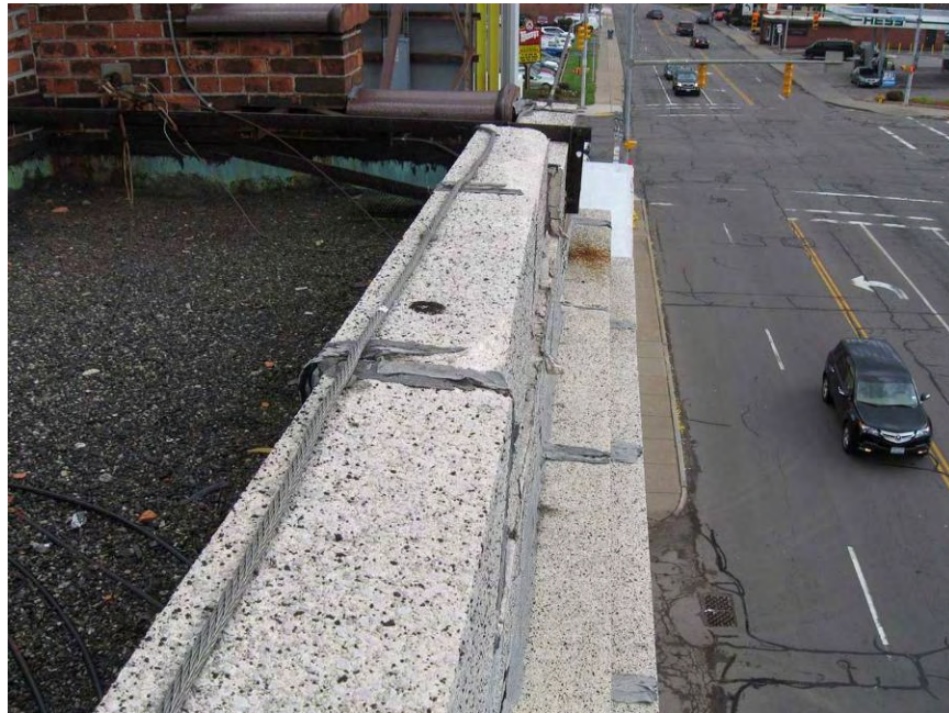
29. South cast stone parapet – open joints and stone shifting. Refer to 2004 photo 18.
