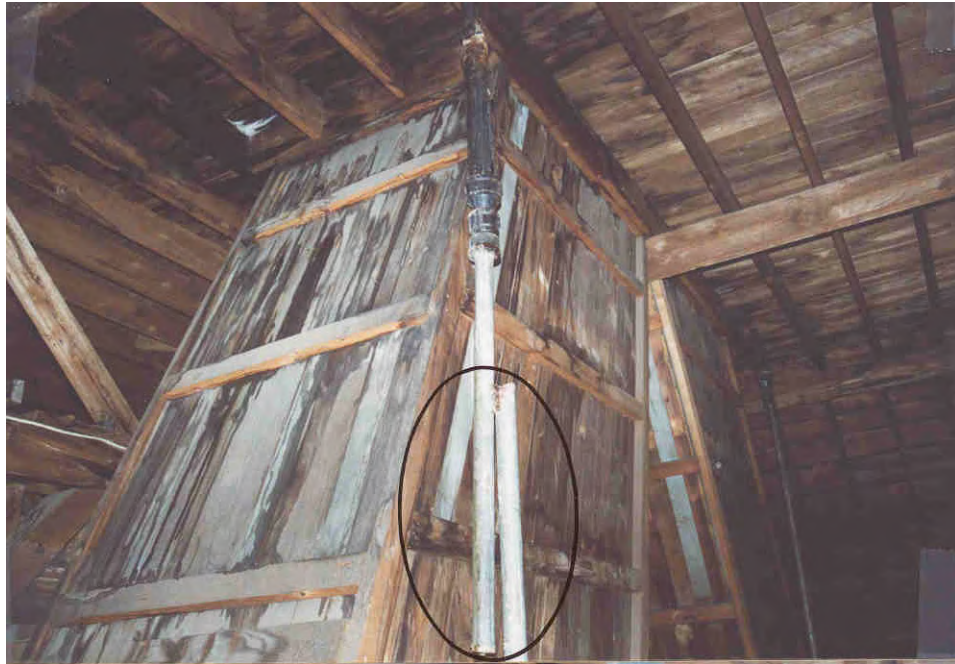
50. Broken plumbing vent pipe.
