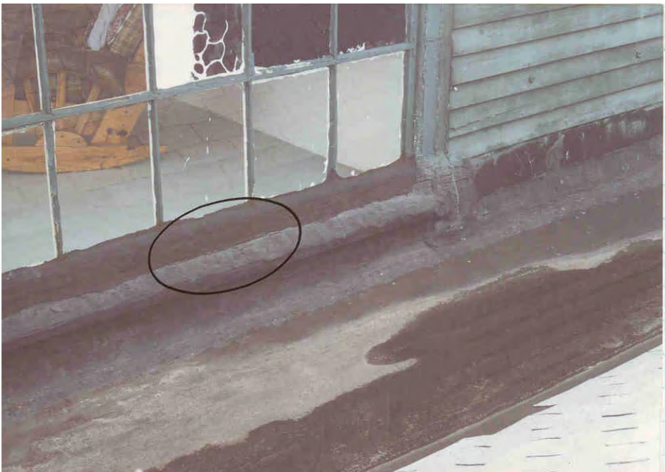
26. Tar covered northwest 2nd floor windows
