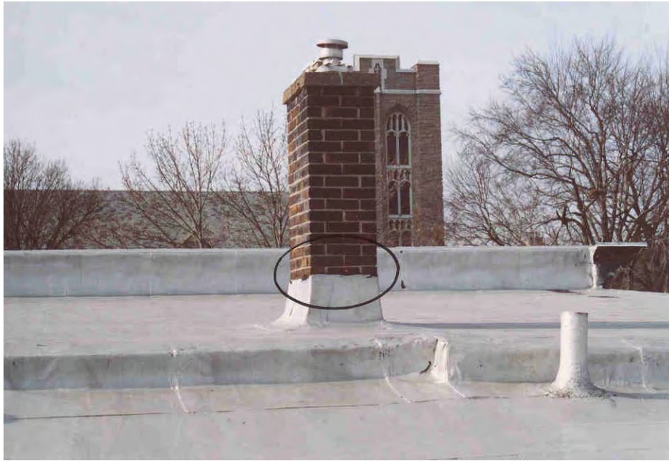
9. Missing counter flashing on west chimney.
