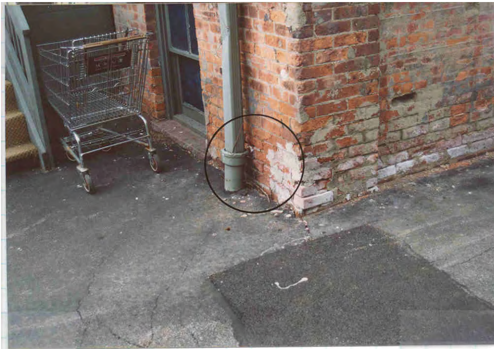
15. No clean-out at storm drain.
