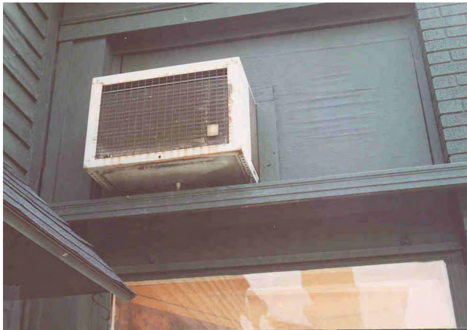
32. Rusted air conditioner and deteriorated trim.
