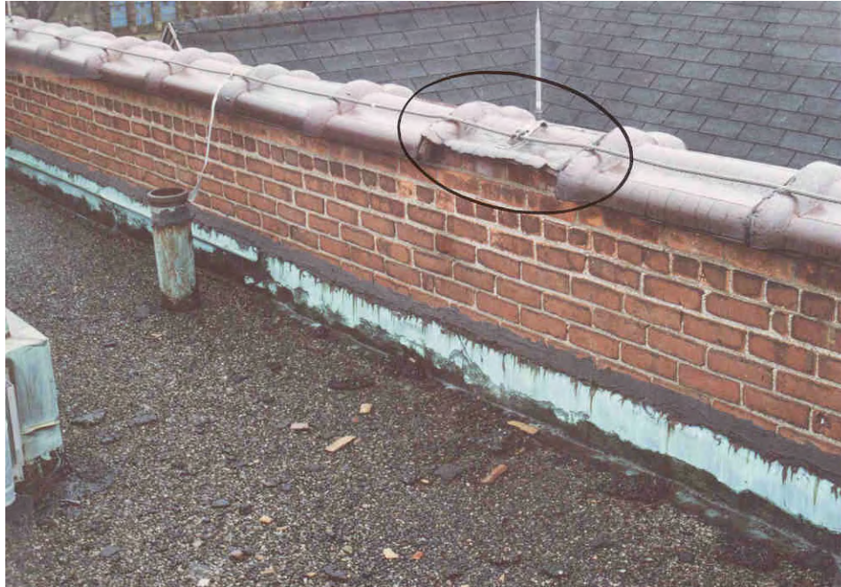
19. Broken coping tile at roof 4.
