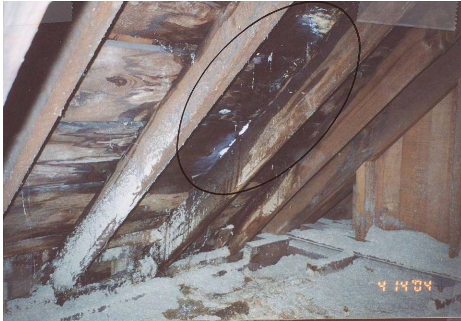
28. Rot at roof rafter and deck.
