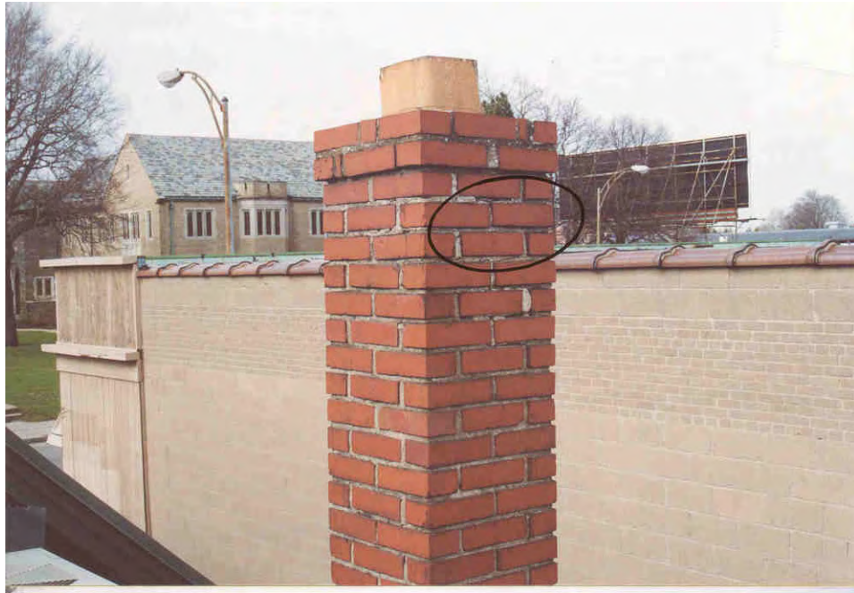
13. Deteriorated mortar joints and missing cap.
