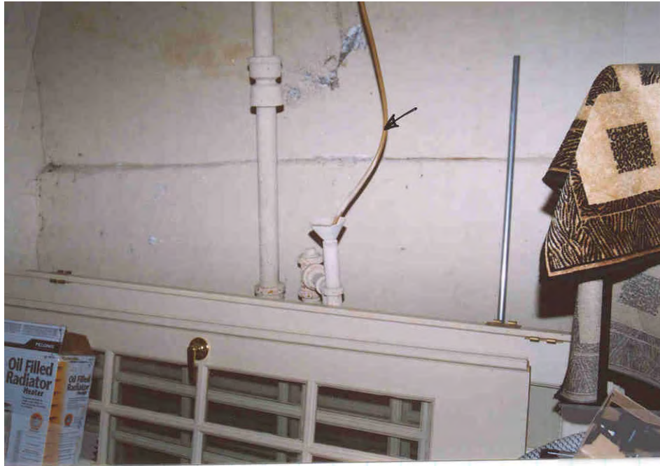
48. Furnace condensation hose 35' long.
