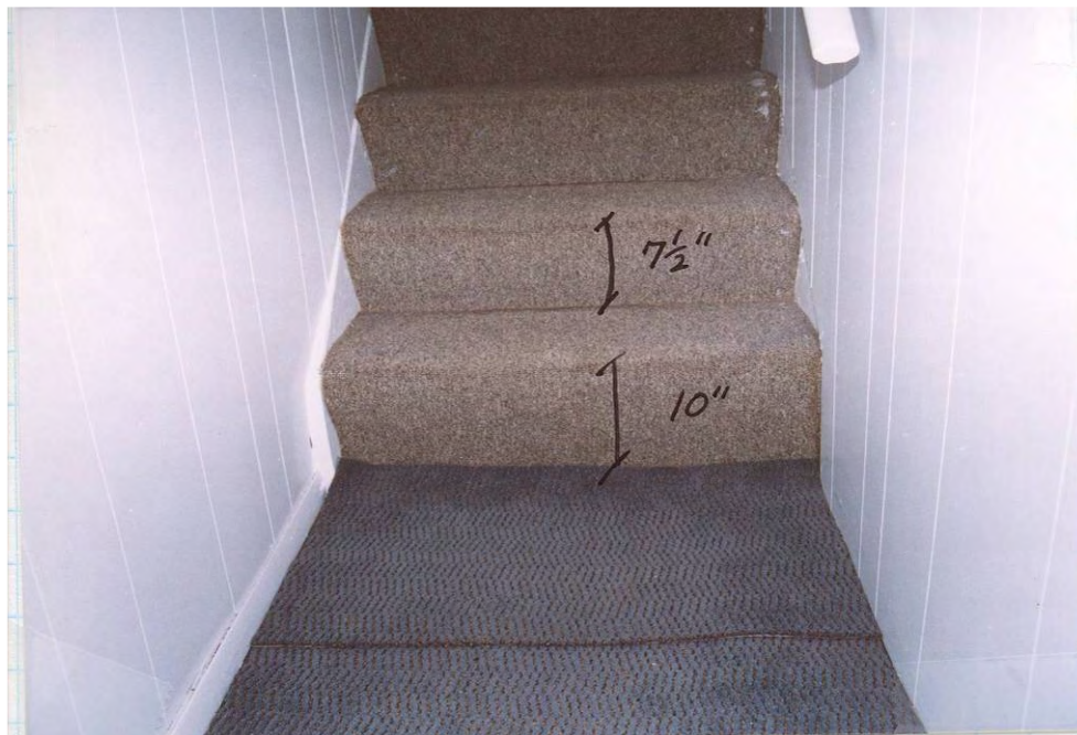
33. High first step in basement.
