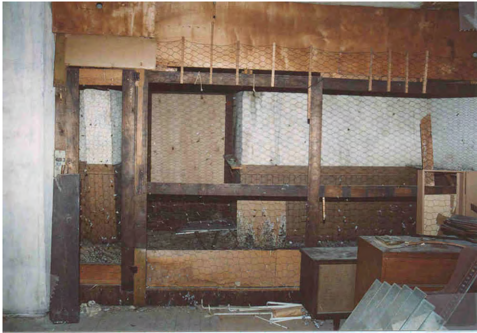
45. Chicken wire attic wall.
