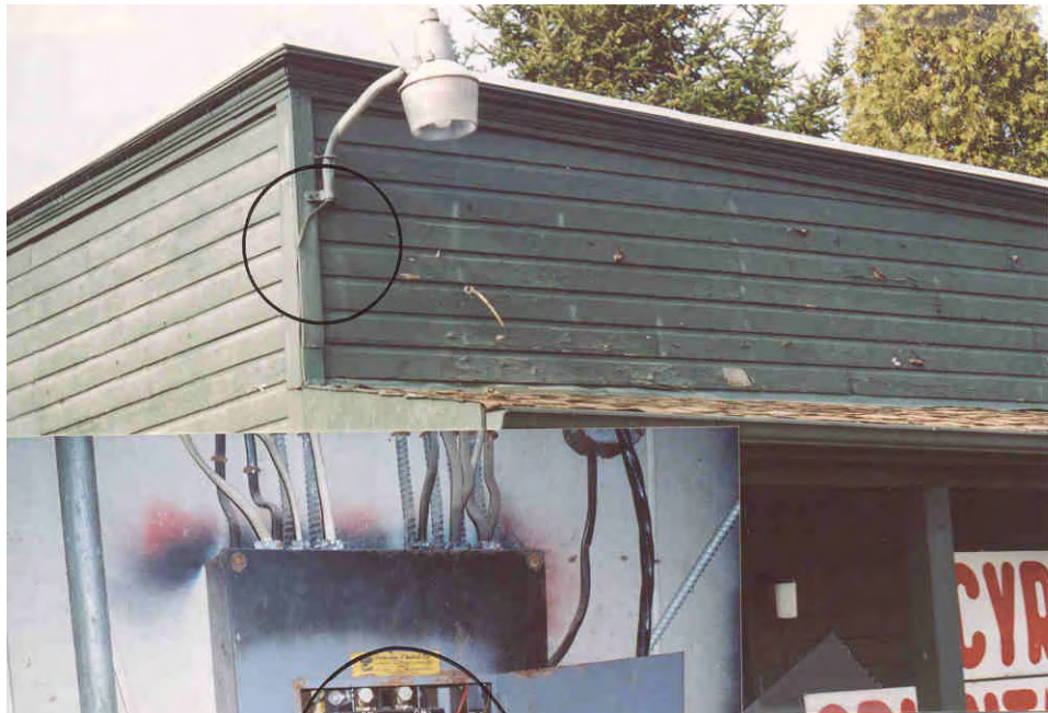
34. Exposed wiring at north.
