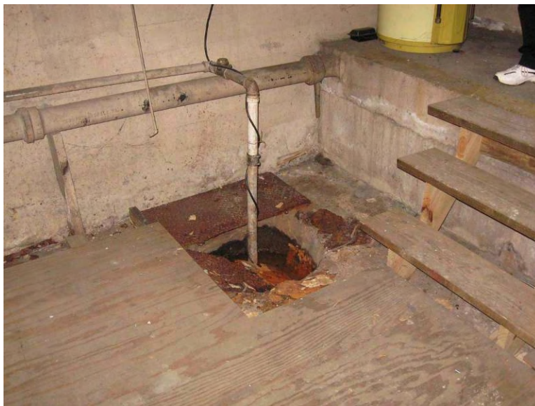
35. Basement sump with broken cover near stair. This is a safety issue.
