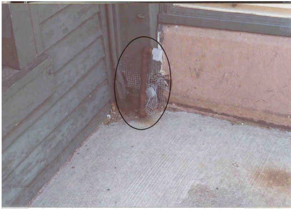
24. Damage to trim at fuel oil fill pipes.
