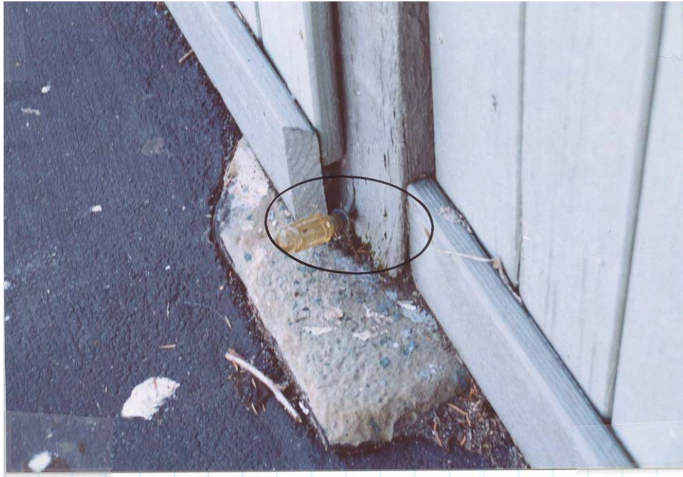
36. Rot at north porch column.
