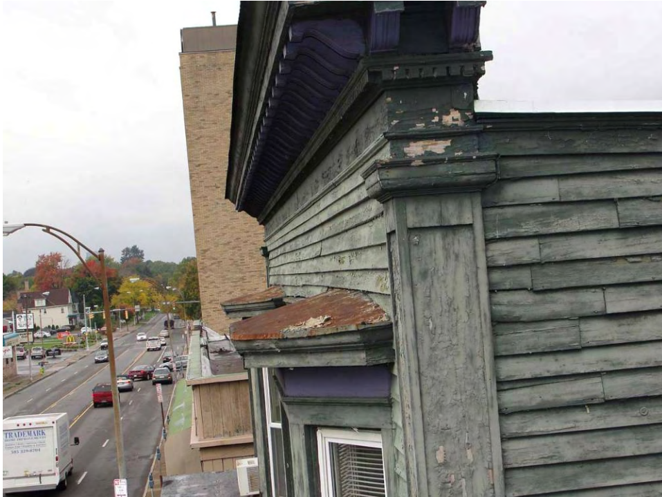
43. South bay window roof deterioration.
