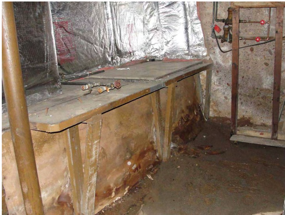
40. Basement – NE corner – water and silt intrusion.
