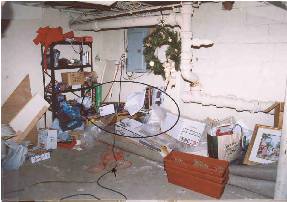
52. Storage and debris in front of electric panel.
