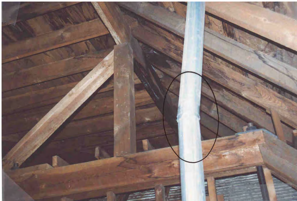
51. Inappropriate connection of flue pipe.
