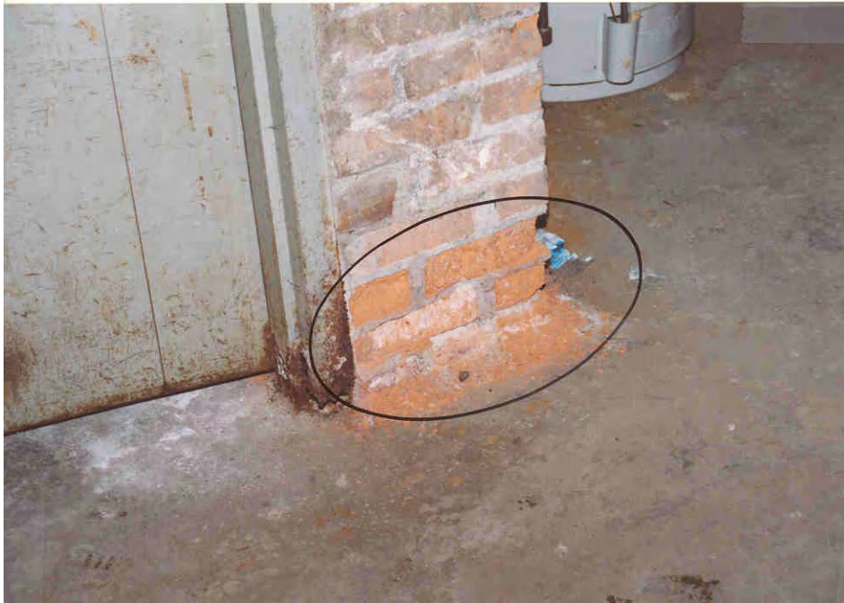
22. Deteriorated basement column.
