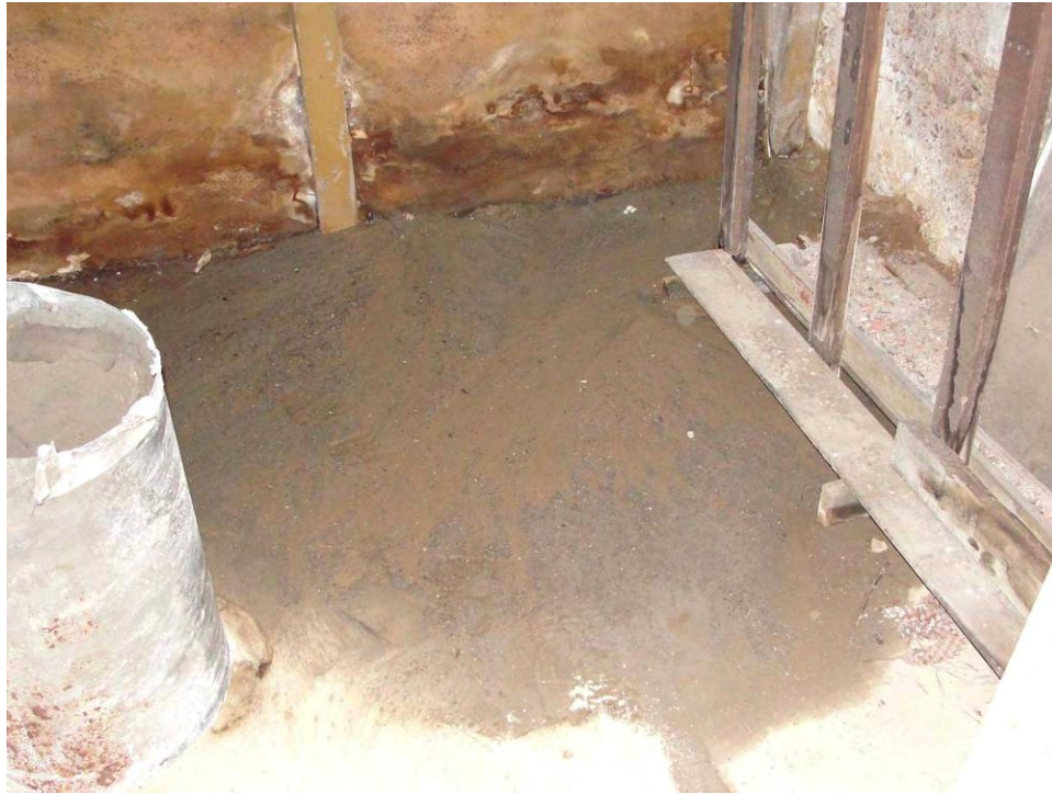
39. Basement – NE corner – water and silt intrusion.
