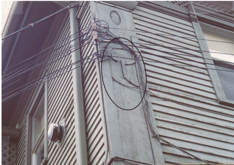
31. Deteriorated pilaster trim.
