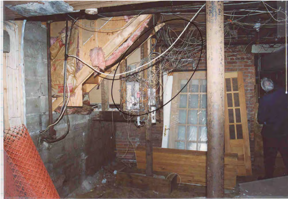
54. Abandoned and unsupported wiring
