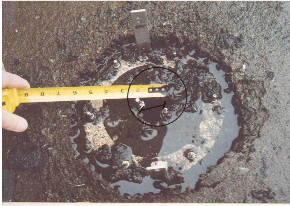
8. Constricted south roof drain.
