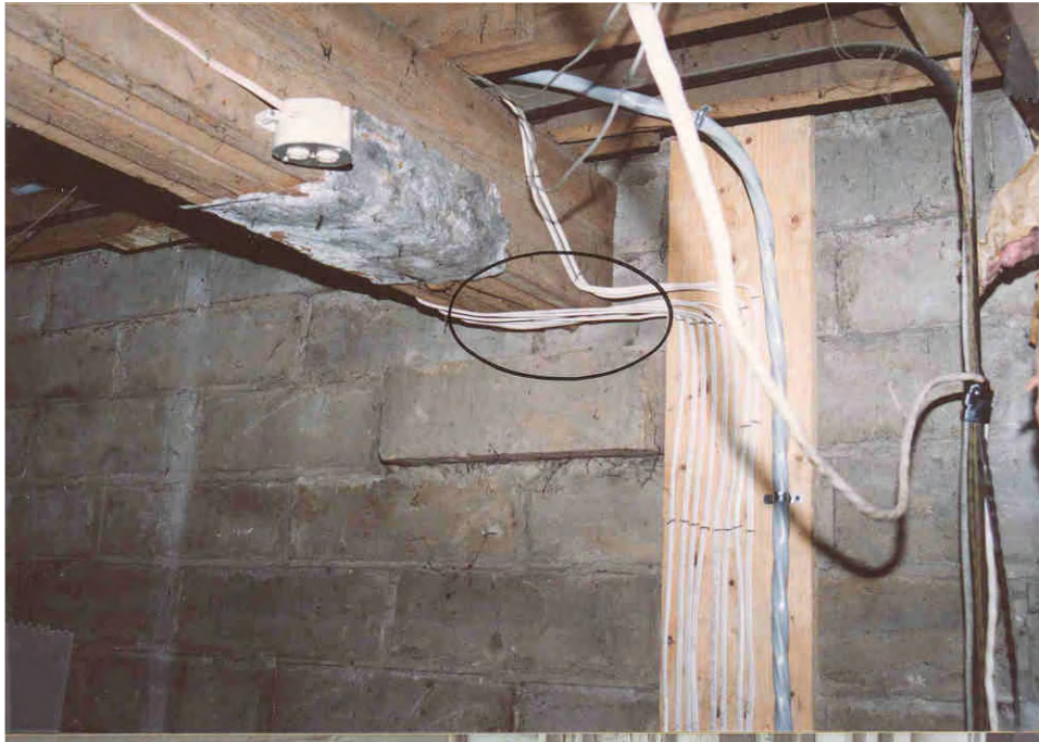
22. Beam end without bearing.
