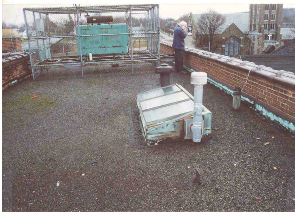
10. Tar covered flashings and multiple penetrations.
