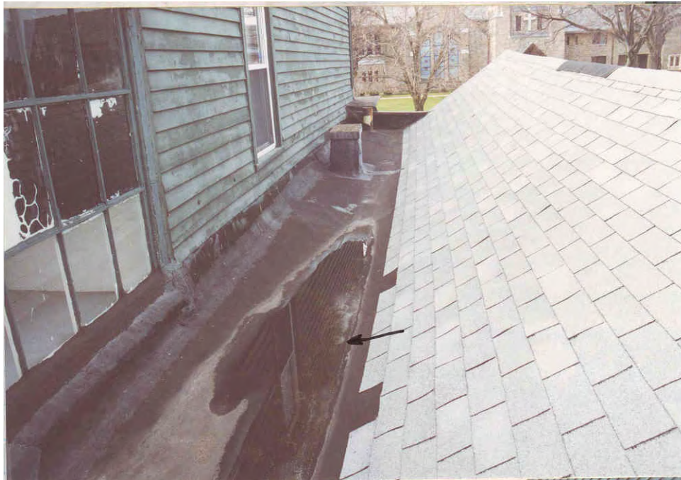
8. Valley between buildings 1 and 2, note standing water.
