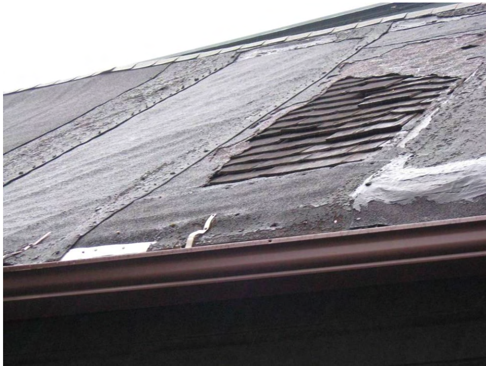
24. West gable roofing deterioration. Compare to 2004 photo #11.
