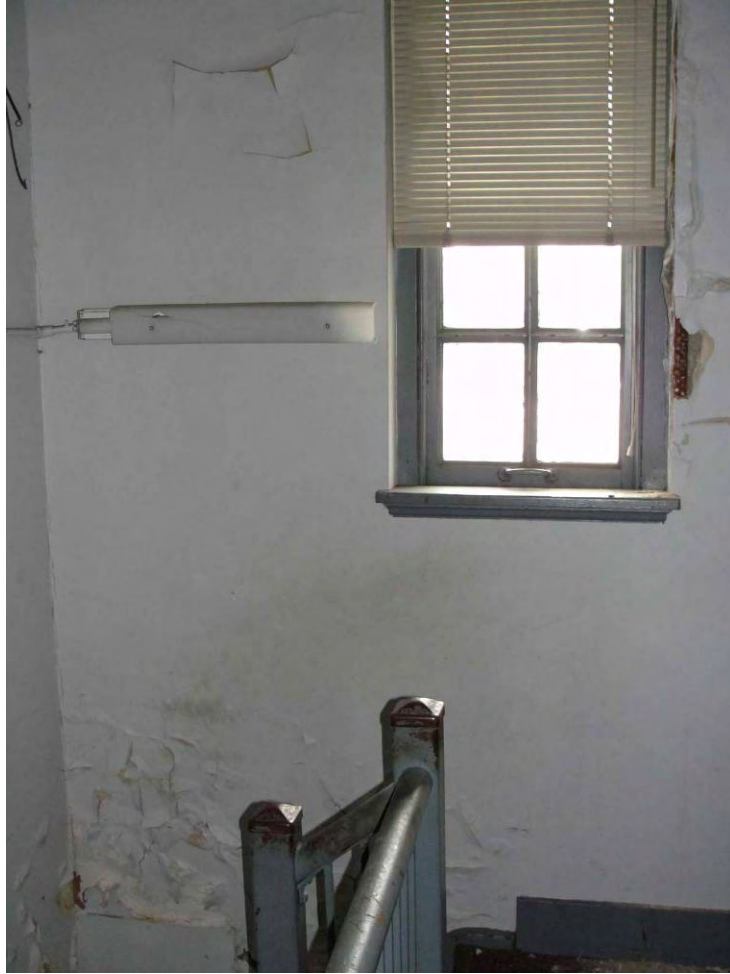
26. Continuing interior finish deterioration due to moisture intrusion.
