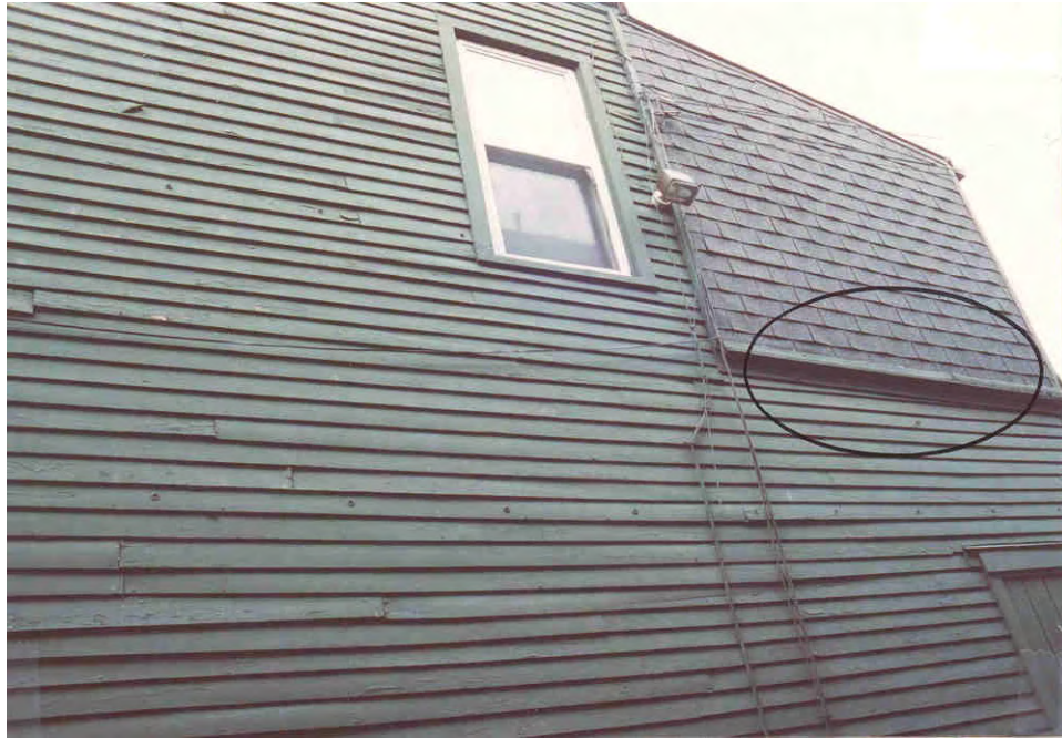
13. Missing flashing at shingle sidewall.
