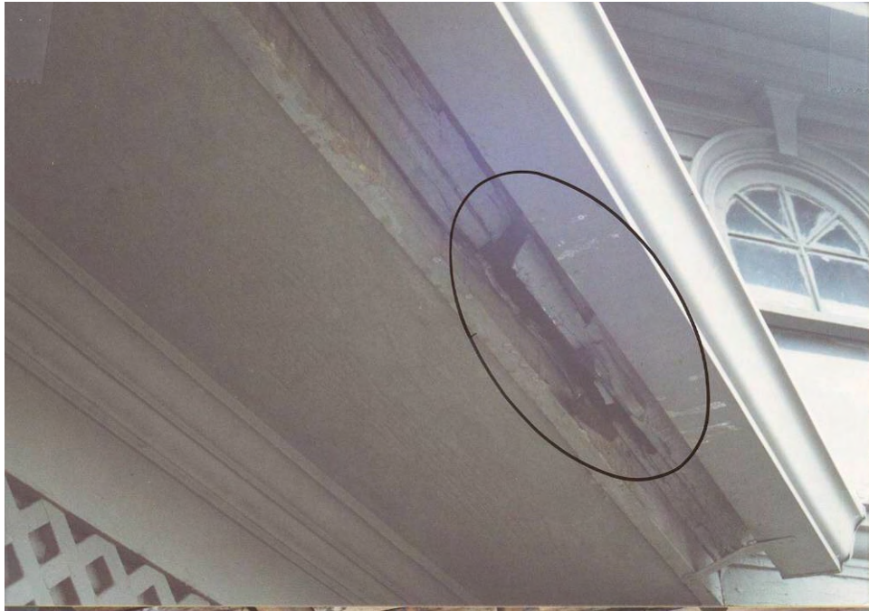
26. Rot at cornice.
