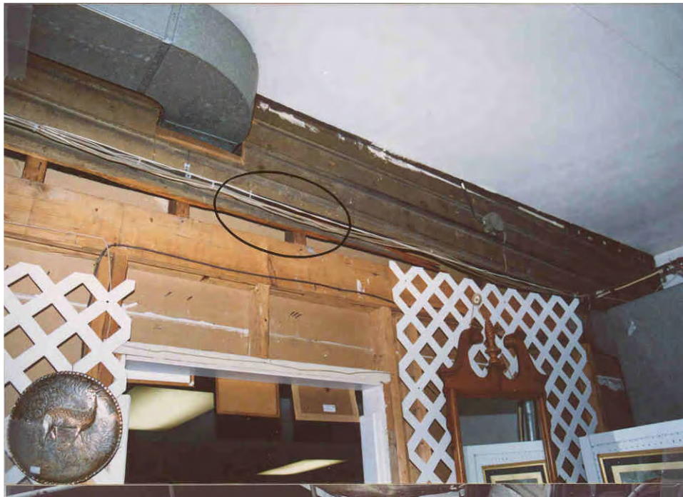
20. Unfinished wall and exposed wiring at north wall of building 1.
