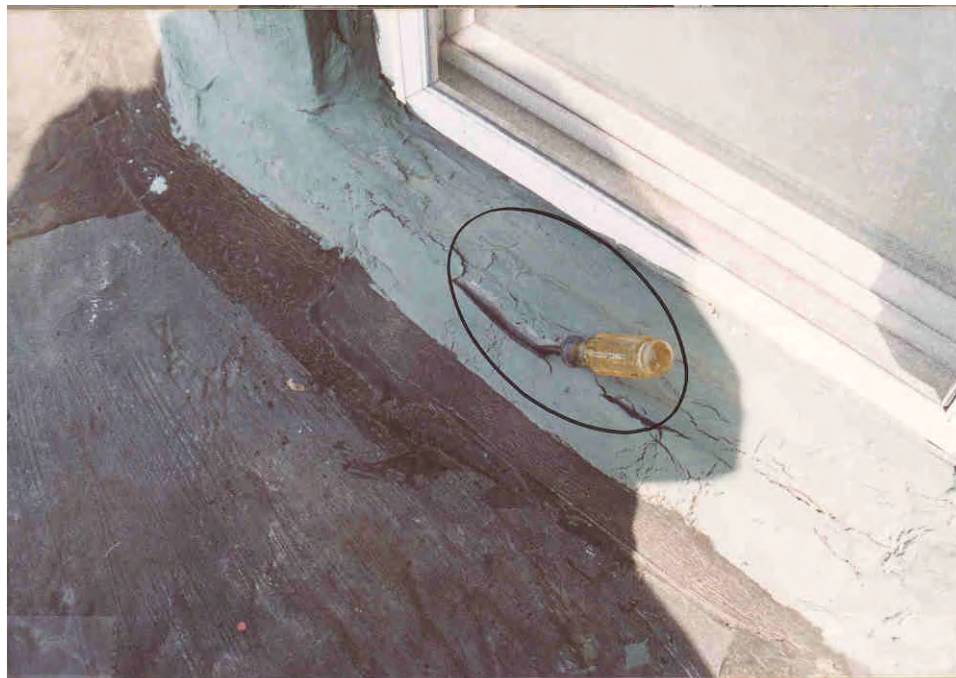
12. Failed flashing at south roofing. 1
