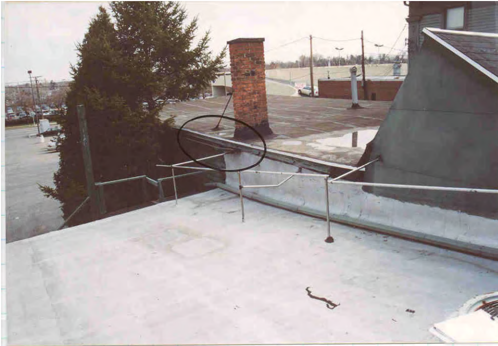
15. Partially missing and deteriorated gutter at west.
