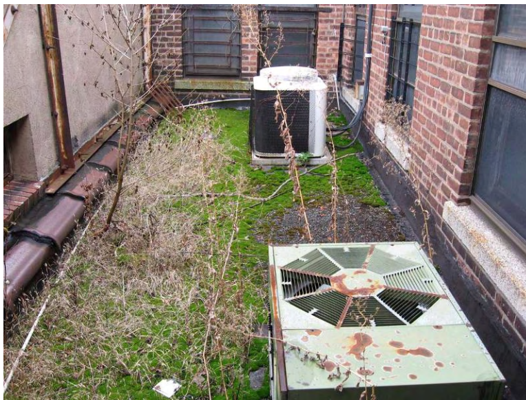
27. Roof 4C – continued vegetation growth and debris. Refer to 2004 photos 11, 12.
