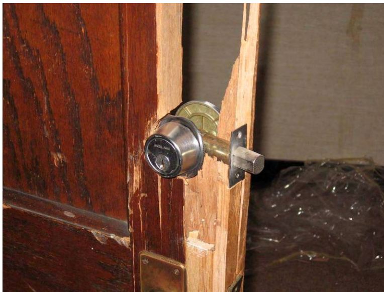
33. Third floor damaged wood door.
