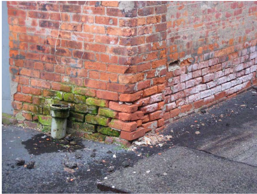
62. North-west deteriorated masonry foundation wall at grade. Note open joints and masonry spalling. Missing downspout. Refer to 2004 photos 3, 15.
