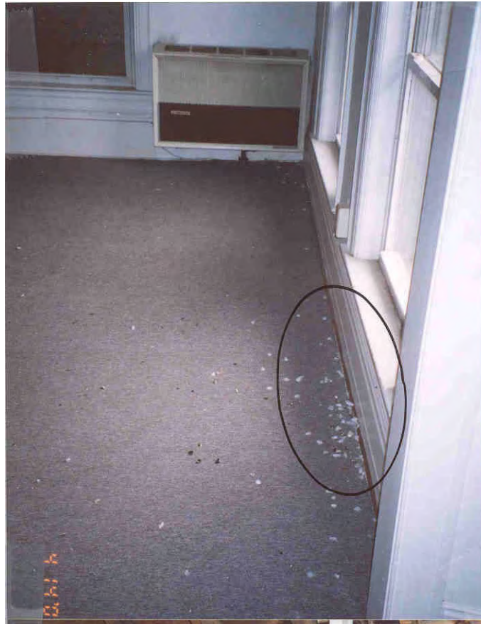
43. Pigeon droppings in second floor apartment.
