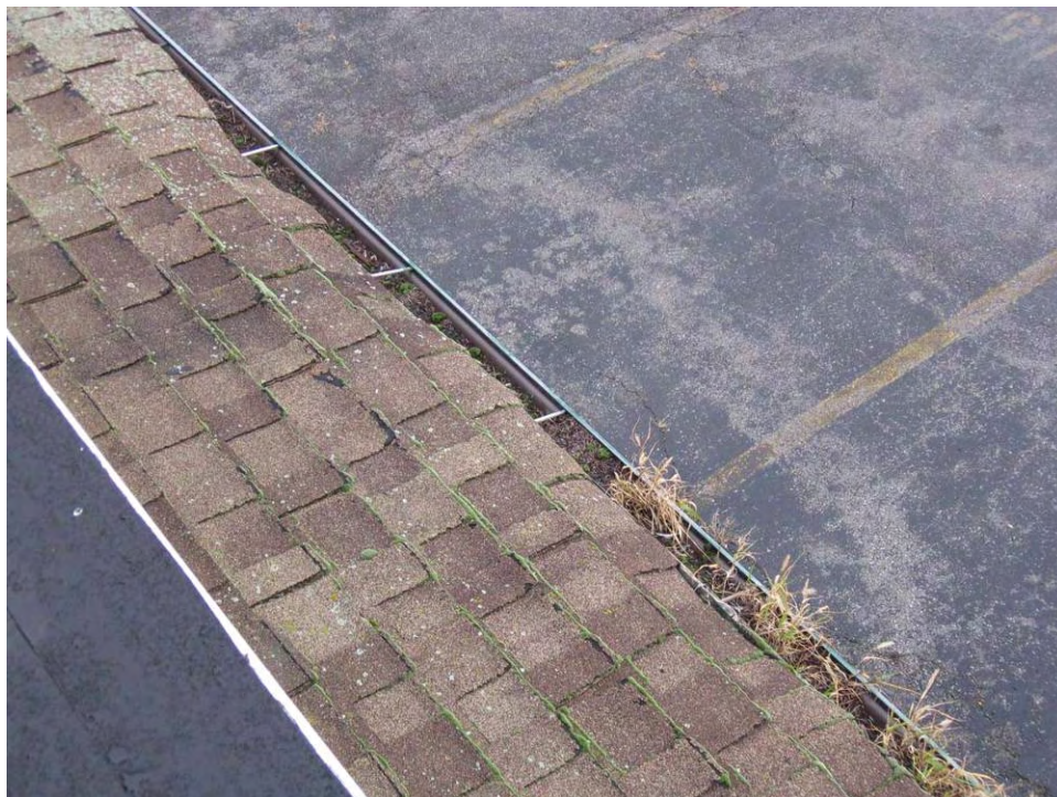
38. North porch roof and gutter deterioration. Refer to 2004 photos 3, and 4.
