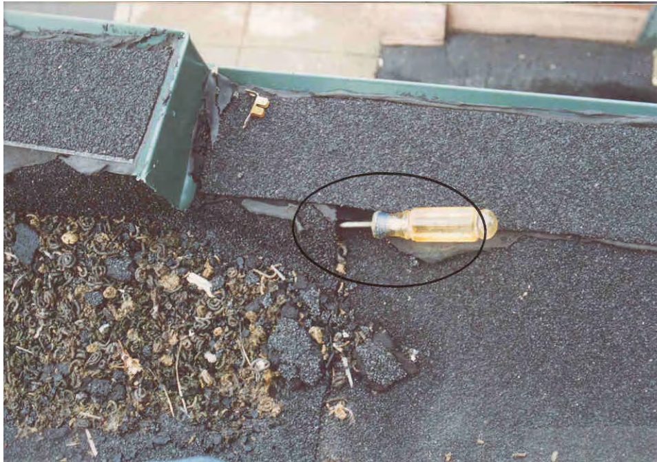
6. Hole at south roof coping.
