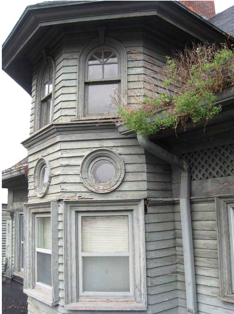
60. South gutters blocked with vegetation.. Refer to 2004 photos 13, 14.
