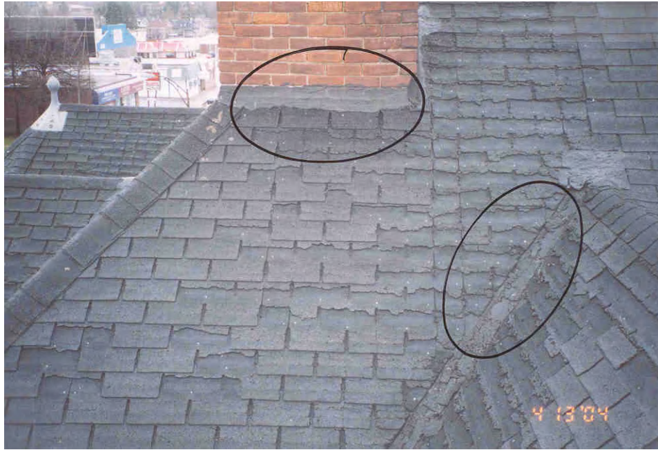
10. Worn main sloped roofing.
