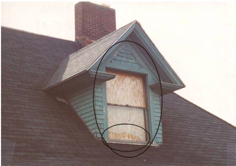
38. Broken west dormer window.
