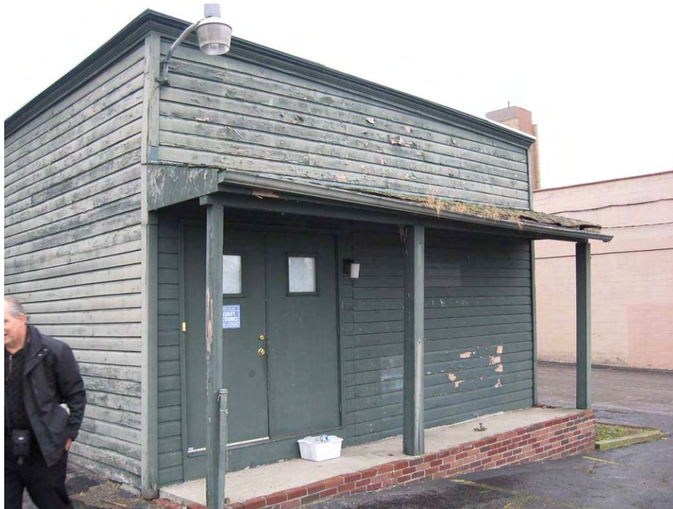
37. North porch roof and framing deterioration. Refer to 2004 photos 3, 4, and 17.
