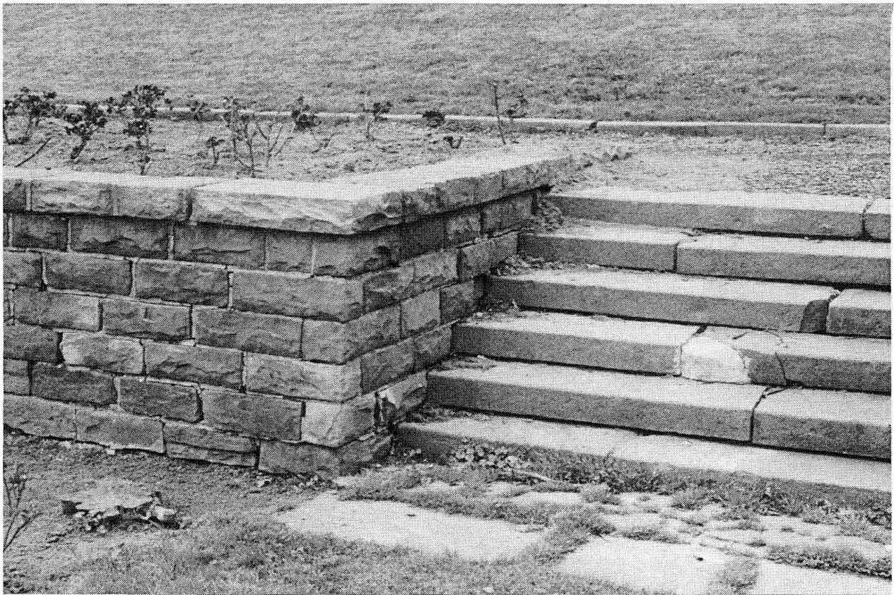
Figure III.7: Maplewood Rose Garden portion of the wall and stairs. Notice the major losses of mortar in the wall and the disintegration of the stair. Courtesy of George Wheeler, 1993.
