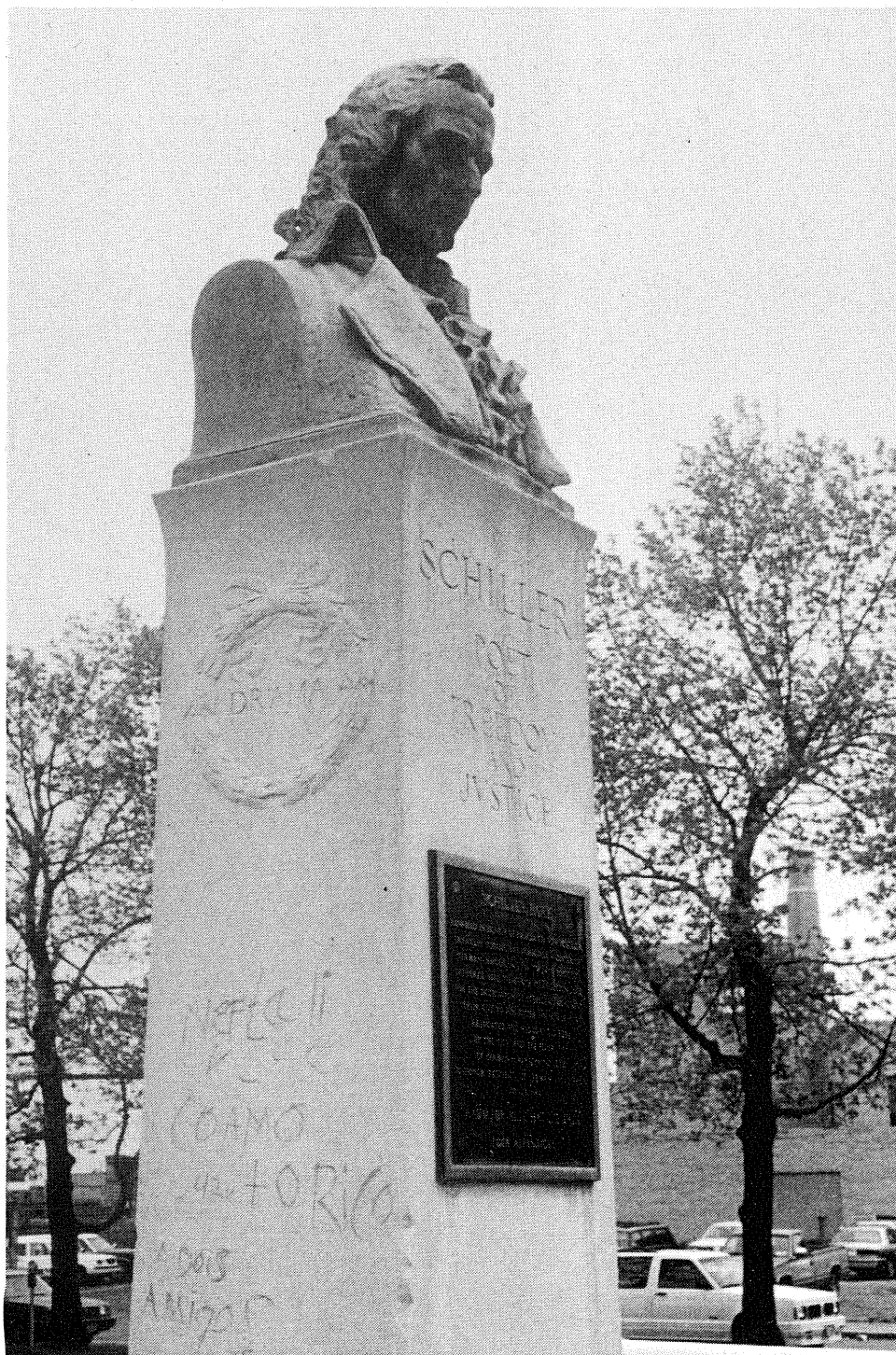
Figure III.8: Schiller Monument in Schiller Park. Notice the run-off from the bronze bust which has stained the limestone. Courtesy of George Wheeler, 1993.
