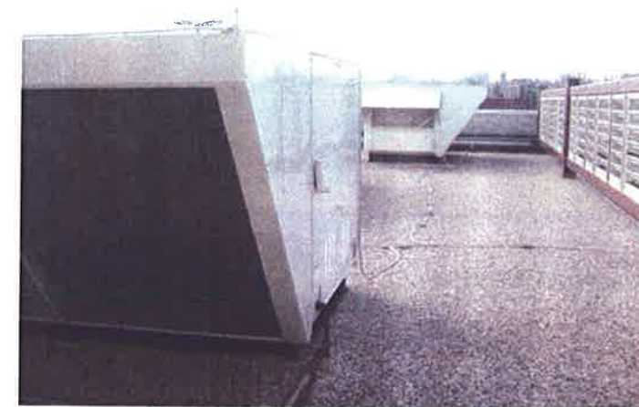
Figure 18. Roof top units
