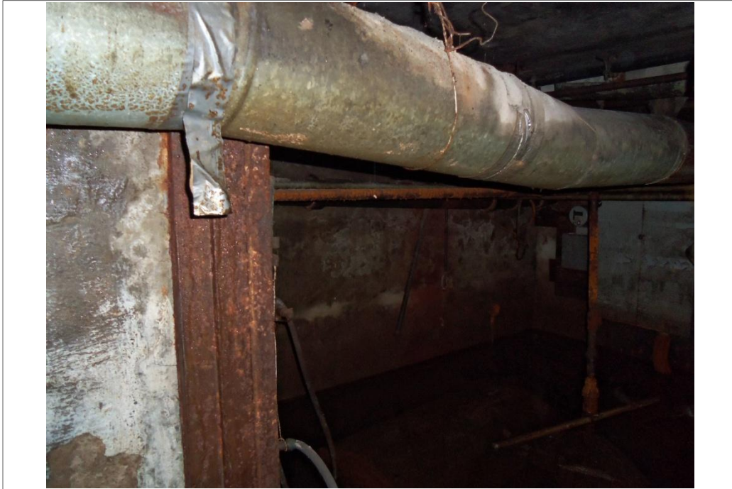
Small tank beneath the water surface in the basement of the vacant former United Cleaners building.
