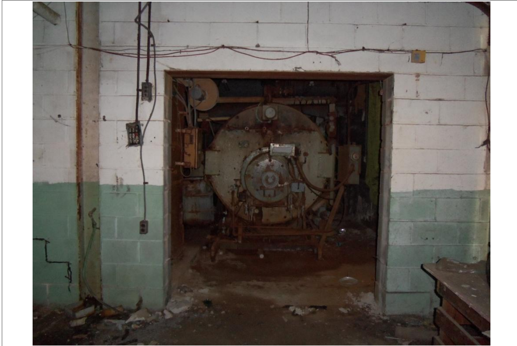
Boiler room in the southeast corner of the vacant former United Cleaners building.
