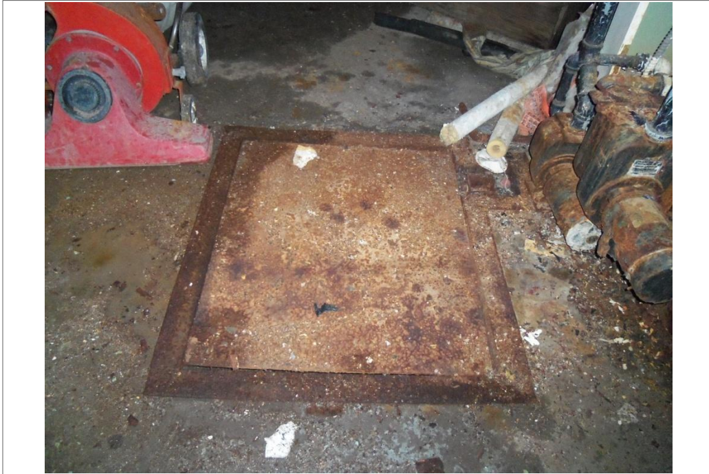
Manway in the main room of the vacant former United Cleaners building.
