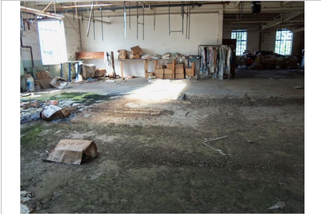
Bird droppings covering the floor on the second floor of the vacant former United Cleaners building.
