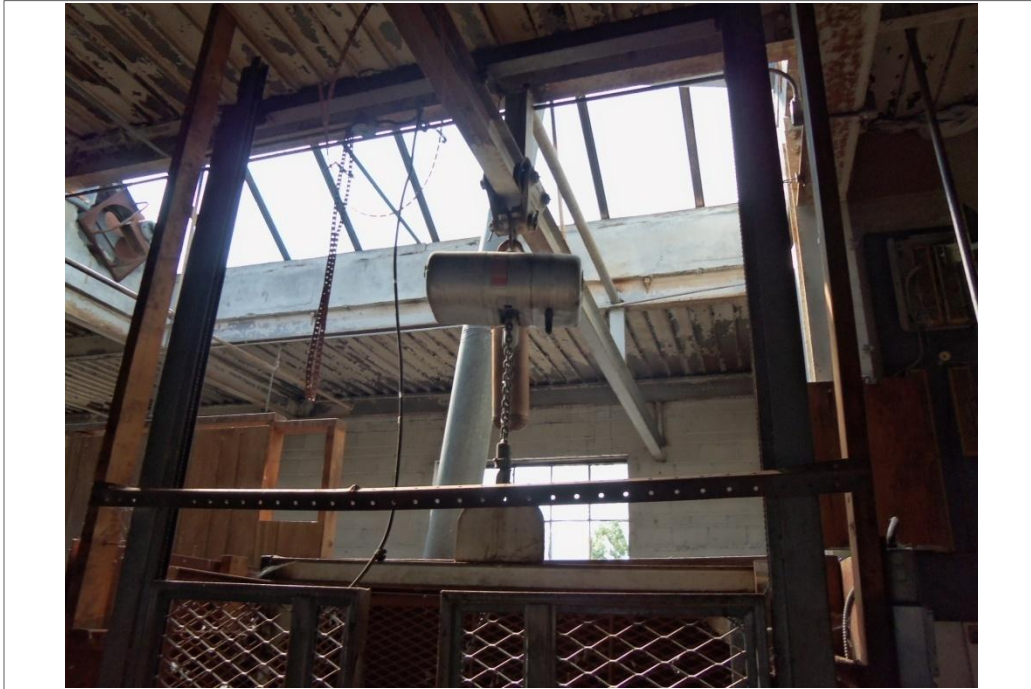
Elevator on the second floor of the vacant former United Cleaners building.
