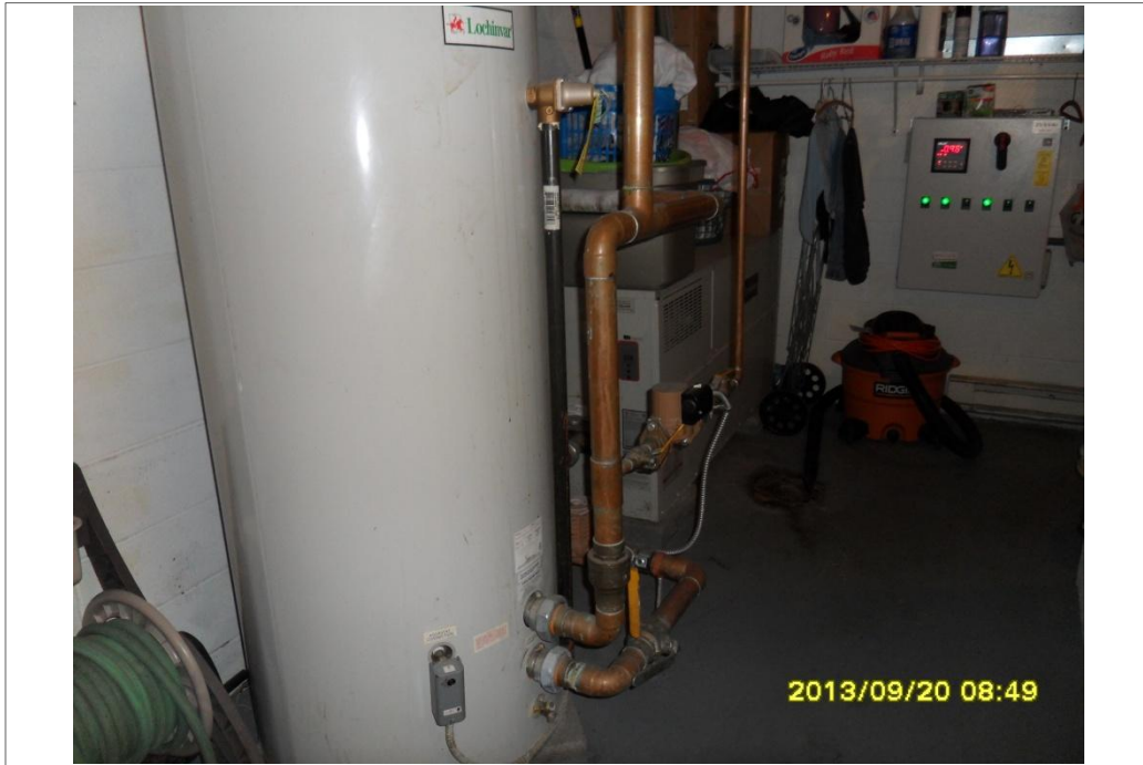
Boiler room in the Canopy Laundromat building.
