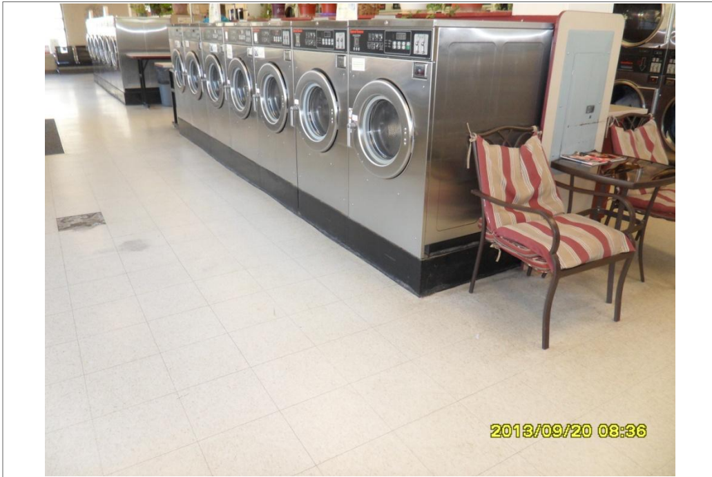
Washing machines in the Canopy Laundromat building.
