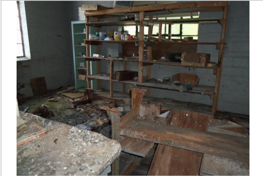
Storage room on the second floor of the vacant former United Cleaners building.
