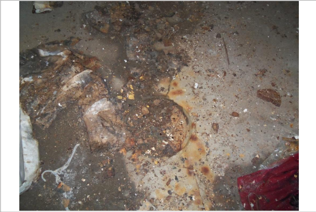
Floor drain in the main room of the vacant former United Cleaners building.
