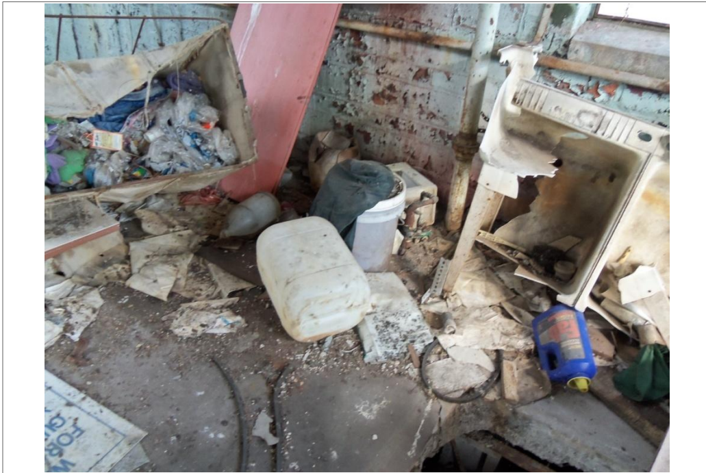
Garbage and empty containers on the second floor of the vacant former United Cleaners building.
