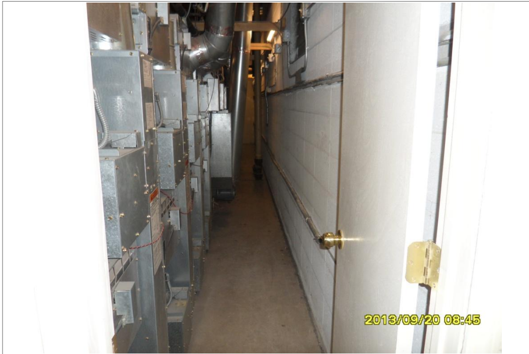
Machine servicing room in the Canopy Laundromat building.
