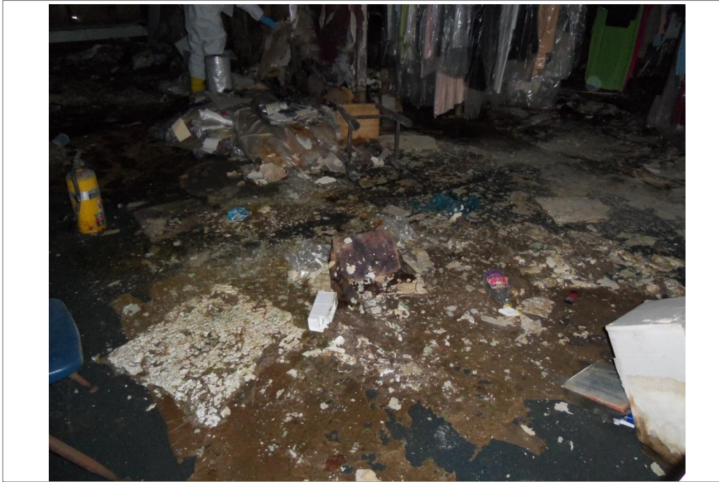
Garbage and mold in the western section of the vacant former United Cleaners building.
