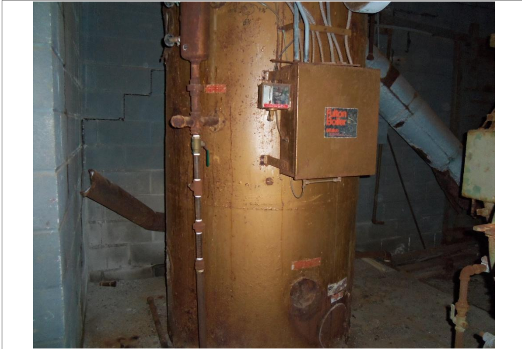
Hot water heater in the boiler room of the vacant former United Cleaners building.
