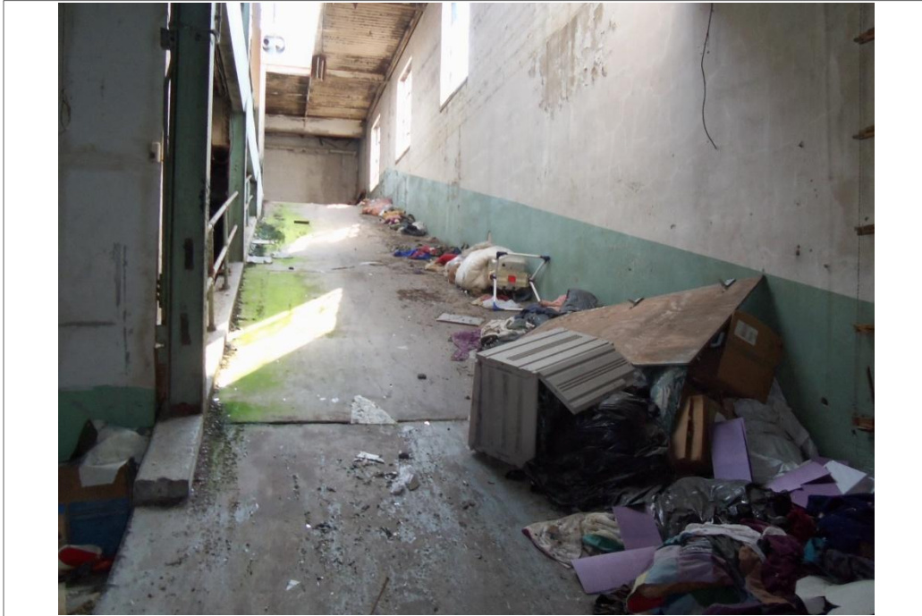
Ramp to the second floor on the south side of the vacant former United Cleaners building.
