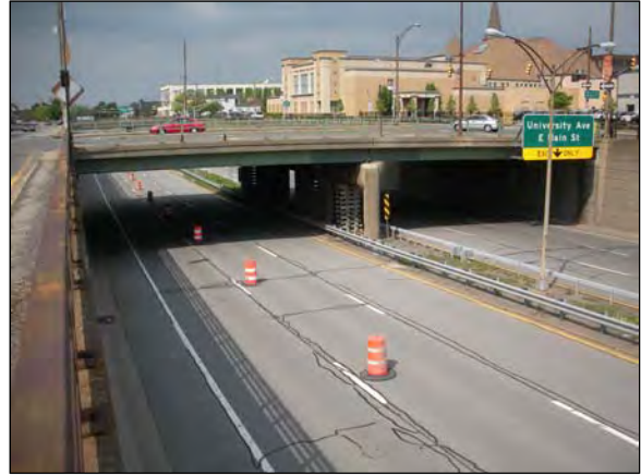
Aging features include; bridge railings, light poles, signals, sign structures, guiderail, bridges, and retaining walls.
