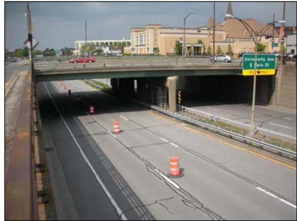
Aging features include; bridge railings, light poles, signals, sign structures, guiderail, bridges, and retaining walls.
