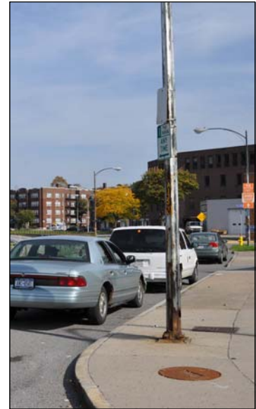
Deteriorated light poles are throughout the project corridor
