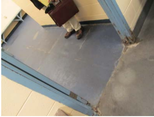
Worn and deteriorated interior finishes
